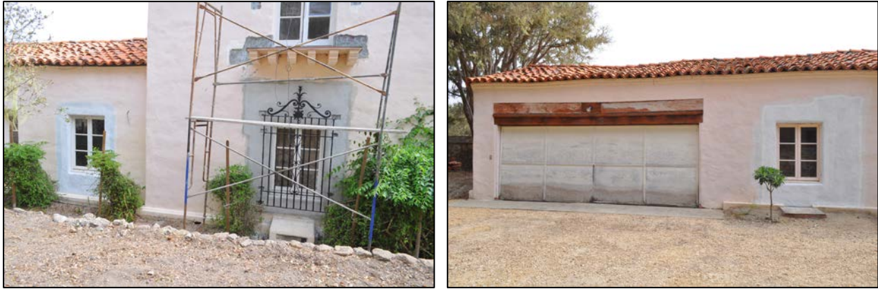
Figures 3 and 4. Left image details the west elevation showing typical stucco decay at window corners and at balcony, due to waterproofing issues. Wood balcony supports and balcony paving will be repaired or replaced in-kind and balcony rails raised to 42 inches to accommodate current code requirements. Right image details the west elevation garage, showing the present non-historic, single garage door. This deteriorated door will be removed and the opening returned to its original two-door configuration.
