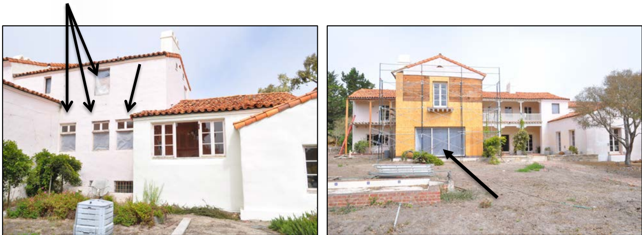
Figures 1 and 2. Left image details the rear (south) elevation, where windows will be replaced in-kind (arrows). Right image shows the rear (south) elevation. The large area of plaster repair was due to poor waterproofing, allowing water to enter behind the wall. Stucco will be reapplied in-kind to match the original stucco. The wide picture window (arrow) can be replaced because it is a non-historic addition to the building.
