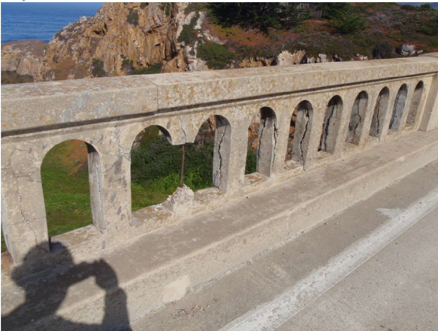
Photo #4 Gross deterioration of bridge railing.
