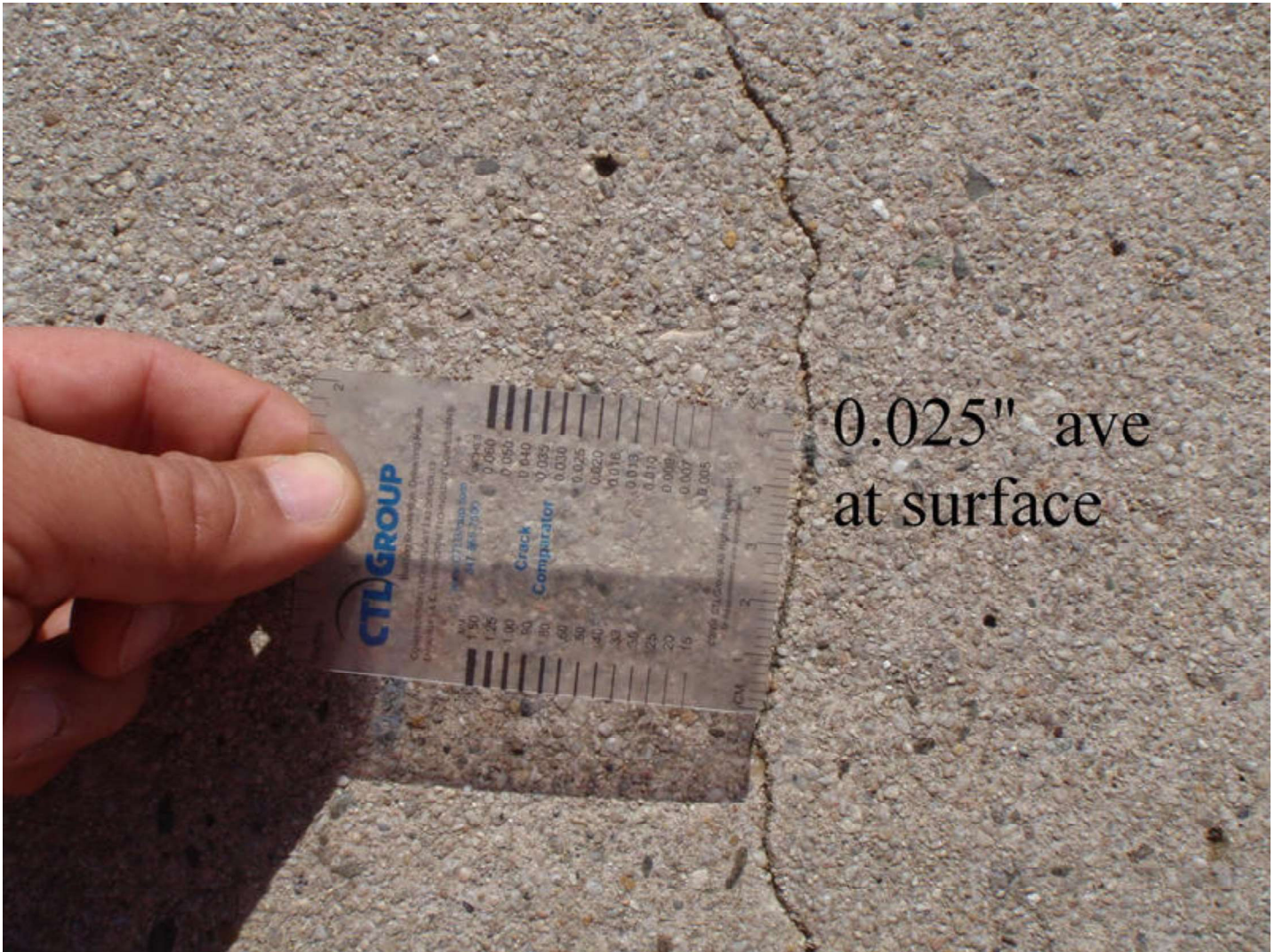
Photo #2 Typical deck crack size.
