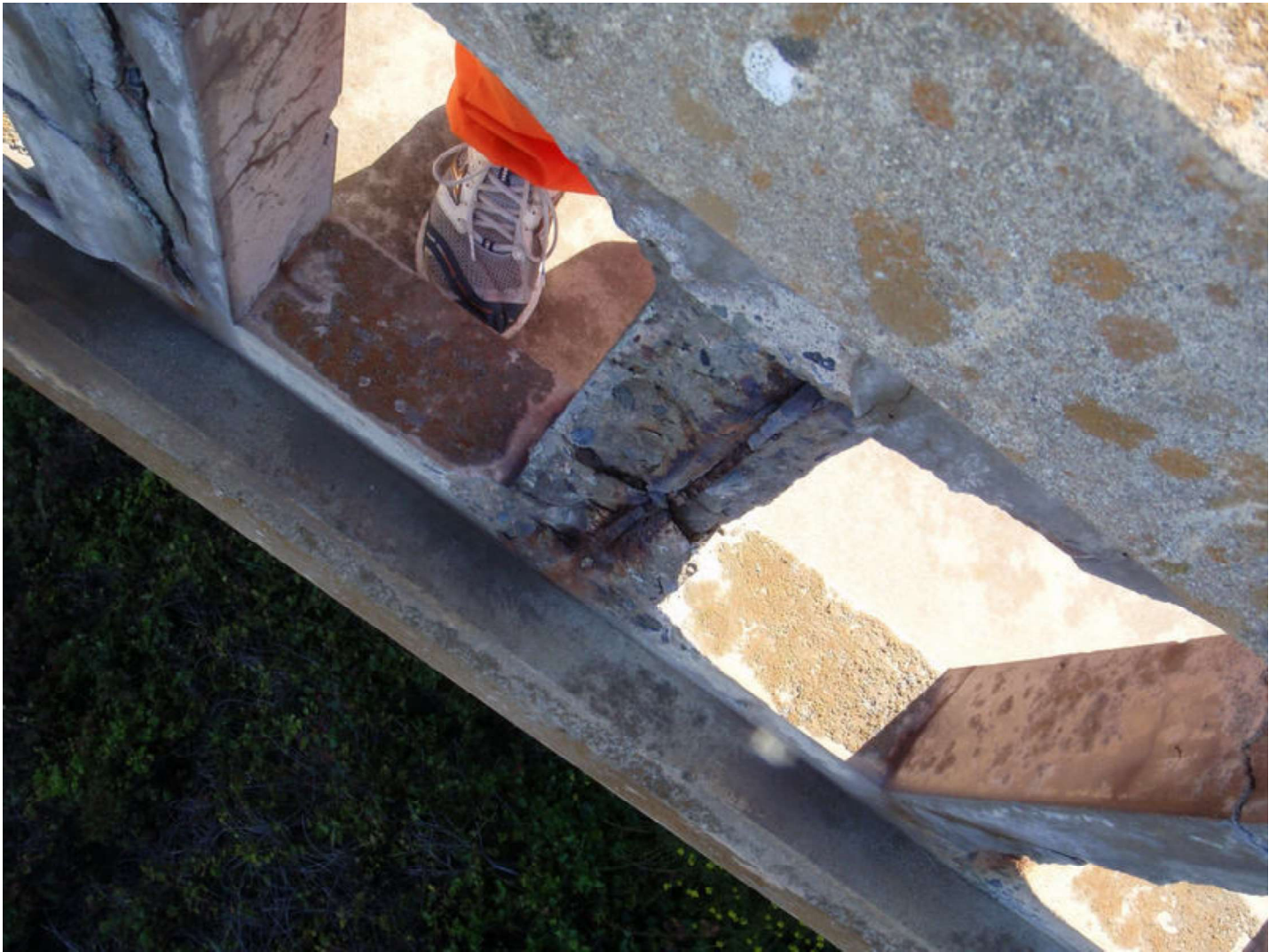
Photo #6 Gross deterioration of bridge railing.
