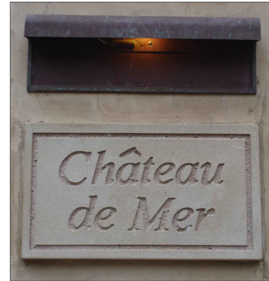
FIXTURE B LED LIGHT UNDER CAP
