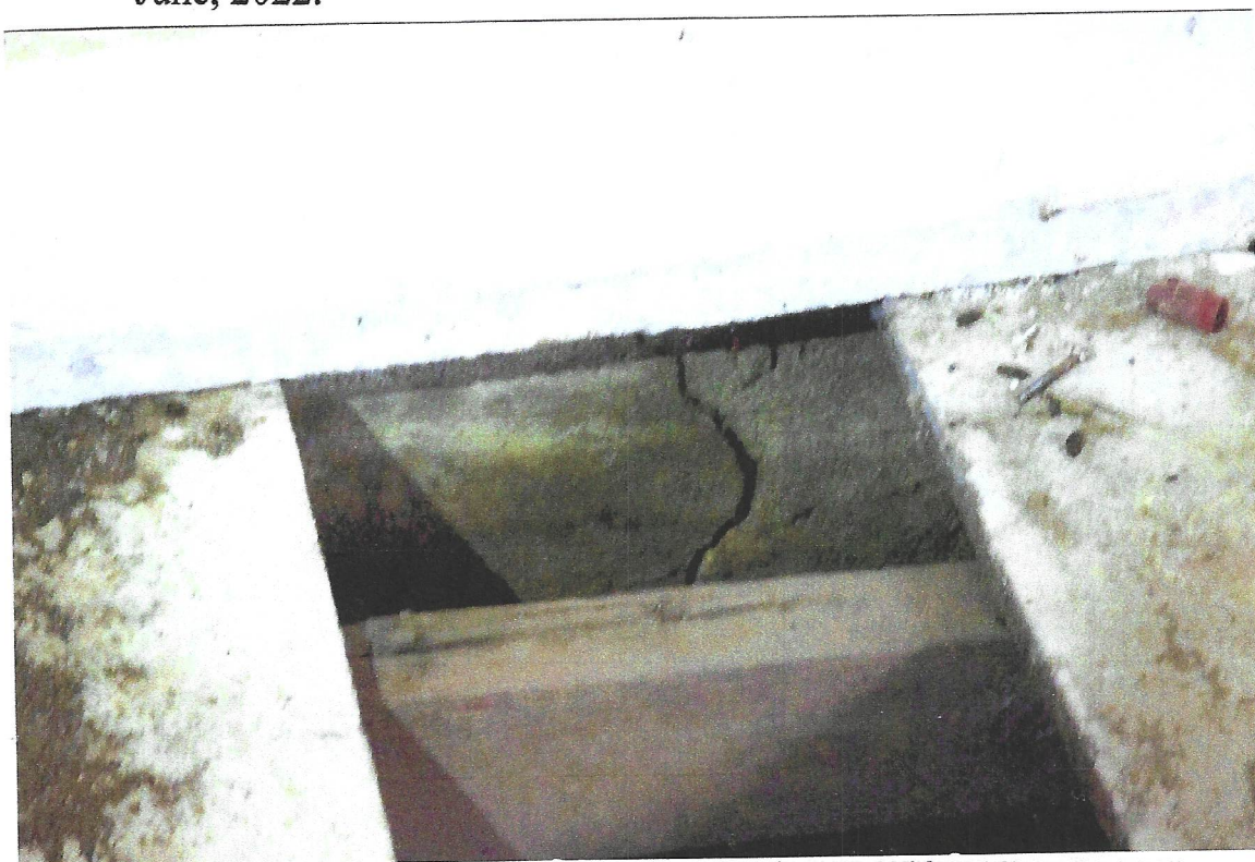
Photo #4. Looking at typical cement foundation failure in living room, Kent Seavey, June, 2022.
