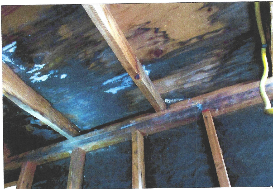
Photo #3. Looking at interior ceiling mold, found throughout bldg. Kent Seavey, June, 2022.
