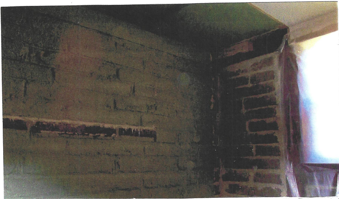
Photo #2. Looking NW at interior wall cladding, note single wythe adobe brick and use of cement mortar, Kent Seavey, June, 2022.
