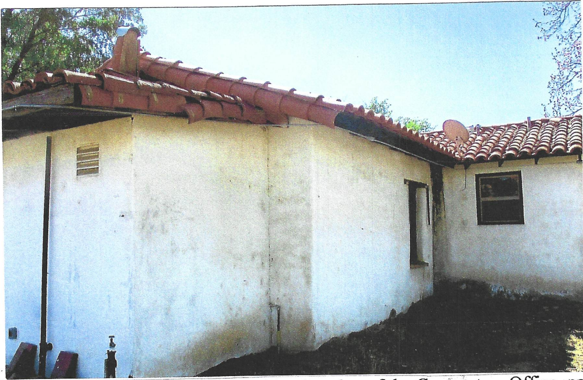
Photo #1. Looking East at the SW side-elevation of the Contractors Office, note mold, left & aluminum window, right, Kent Seavey, June, 2022. (Note: roof tile to be repurposed covering cemetery wall.)
