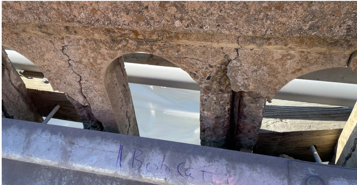
Figure 4: Photos of Bridge Rails dated December 13, 2022
