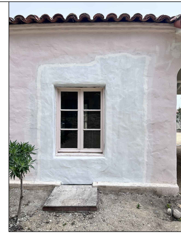
③ BATHROOM 1: STUCCO PATCH & REPAIR, FINISH TO MATCH (E). WINDOW TO REMAIN
