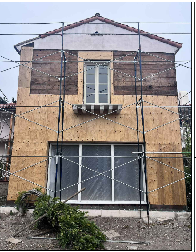
⑥ LIVING ROOM: ROT REPAIR AT PREVIOUSLY ALTERED WINDOW. STUCCO PATCH & REPAIR, FINISH & WINDOW TO MATCH (E).
