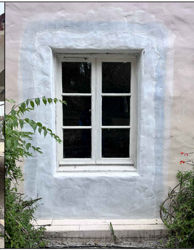
④ BATHROOM 2: STUCCO PATCH & REPAIR, FINISH TO MATCH (E). WINDOW TO REMAIN
