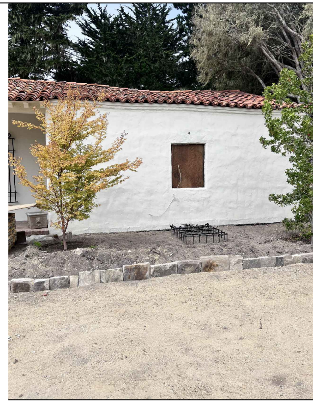
① GARAGE: (E) ROTTEN WINDOW TO BE REPLACED WITH TO MATCH EXISTING MATERIALS (N) WINDOW; PREVIOUSLY ALTERED
