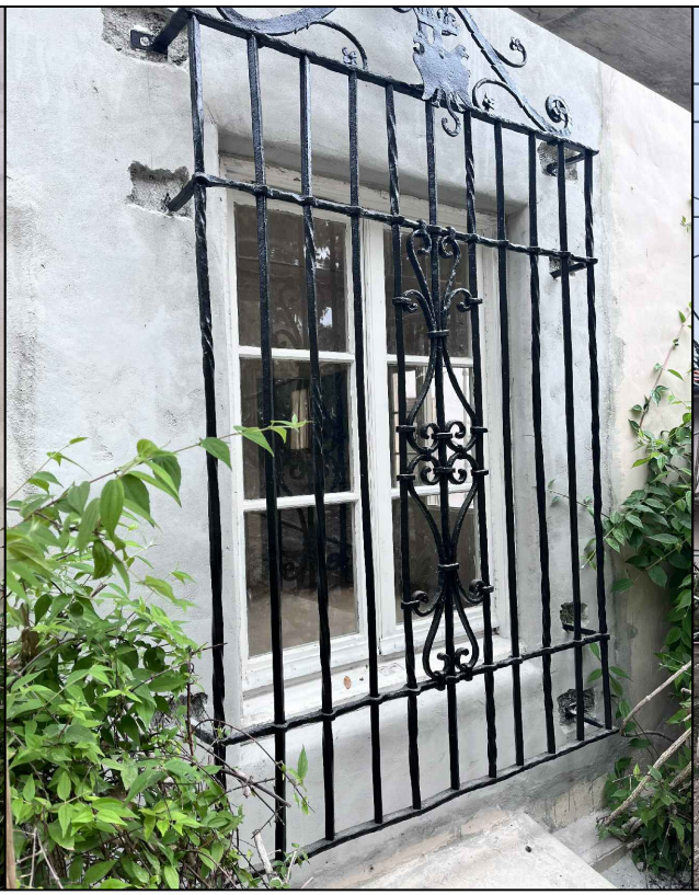
⑤ BATHROOM 2: STUCCO PATCH & REPAIR, FINISH TO MATCH (E). WINDOW TO REMAIN
