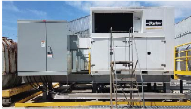
Power Conversion System
