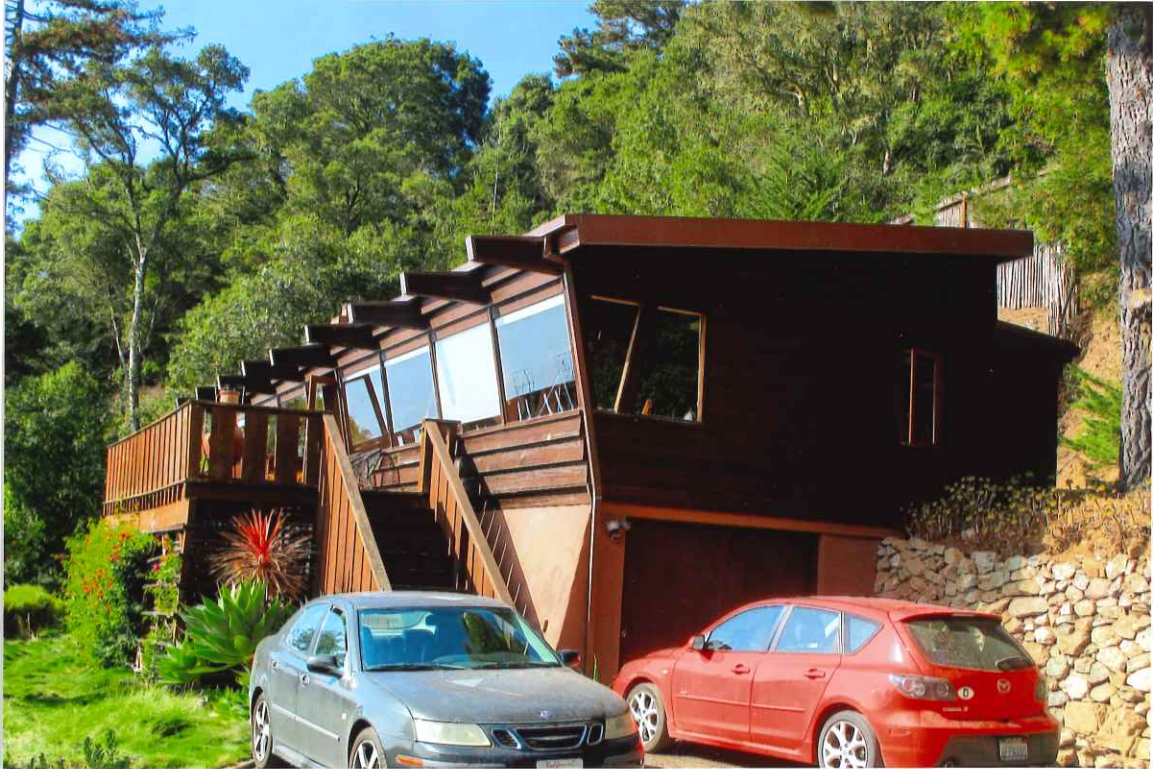
Photo #1. Looking NW at the SE facing entry deck, & access stairs proposed for relocation to the SE side of the deck, Kent Seavey, November, 2020
