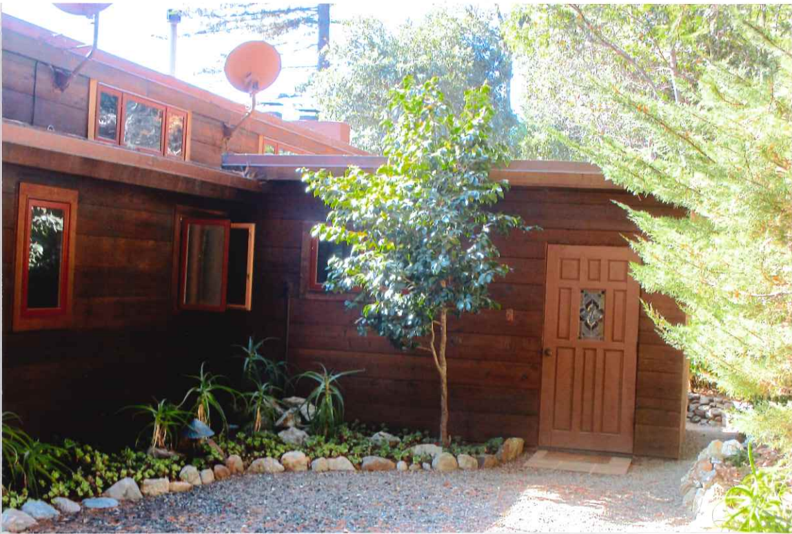
Photo #3. Looking SW at the c. 2008 laundry room addition projecting off the rear elevation, proposed for removal, Kent Seavey, November, 2020.
