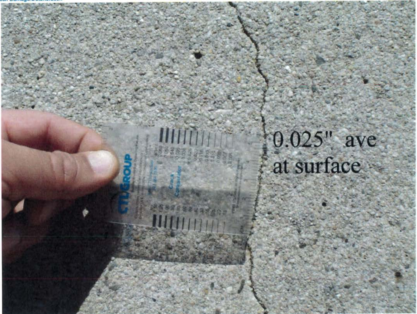
Photo #2 Typical deck crack size.
