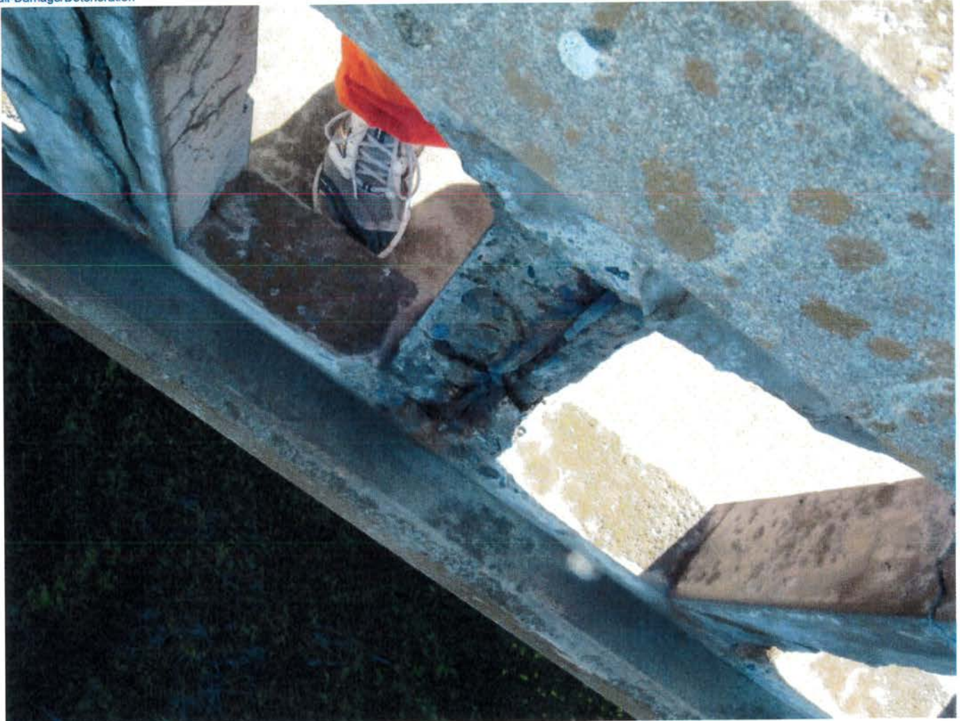
Photo #6 Gross deterioration of bridge railing.
