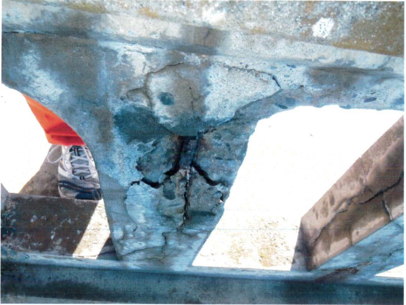
Photo #7 Gross deterioration of bridge railing.
