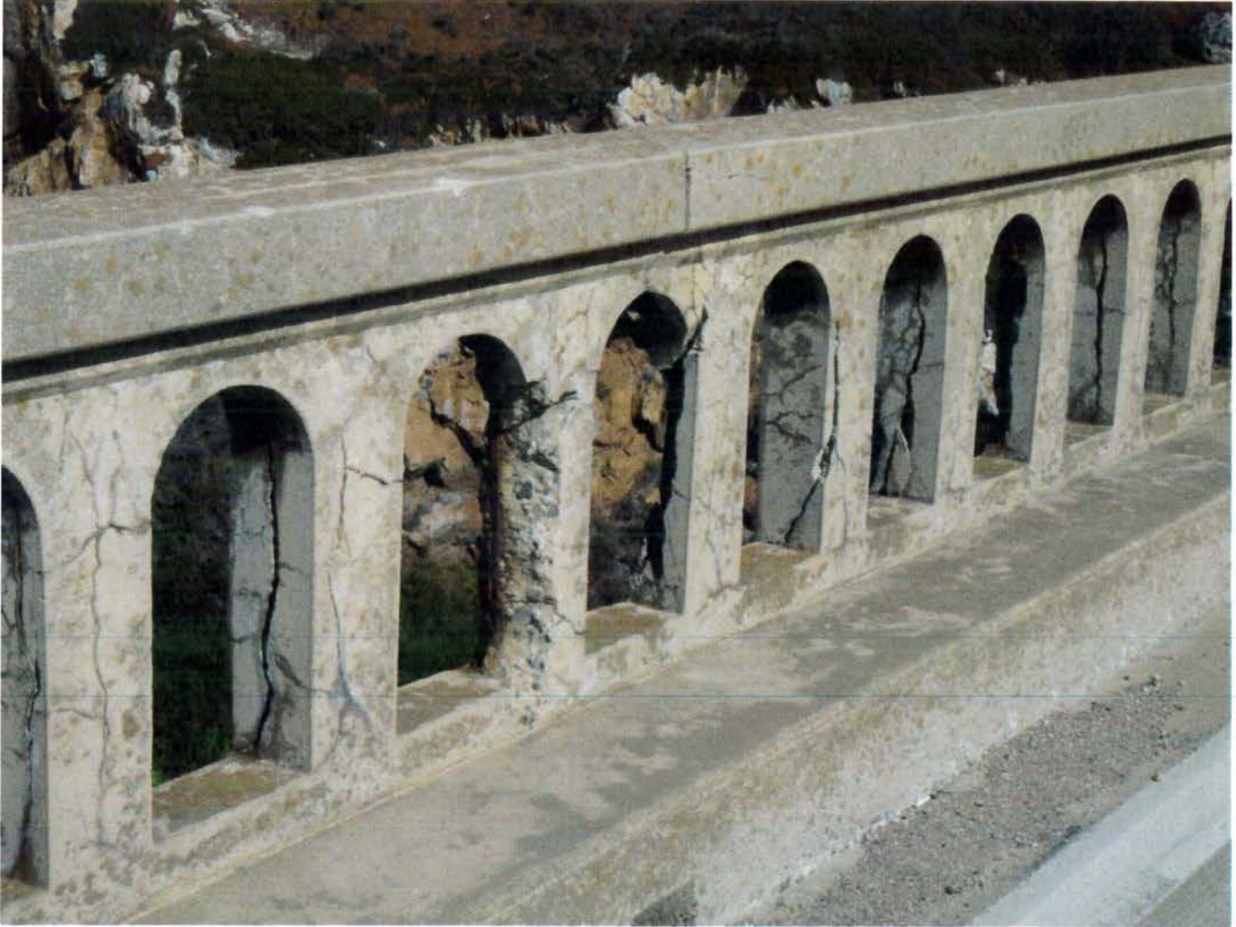
Photo #5 Gross deterioration of bridge railing.
