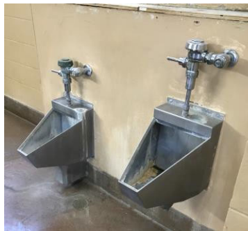
Figure 6. Typical Community Bathroom Water Closet
