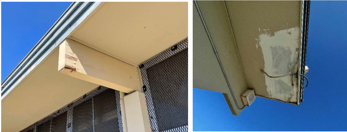
Figure 7 – Slight damage to beam overhang and soffit
