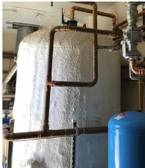
Figure 11. Existing Hot Water Storage
