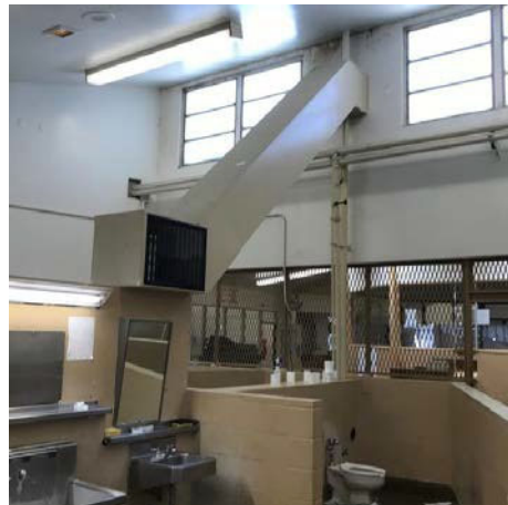
Figure 4. Typical Community Bathroom Exhaust Fan
