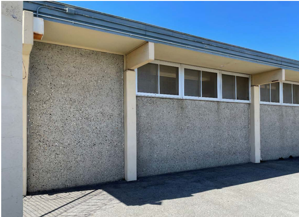
Figure 6 – Typical exterior wall of the wing section with windows full length of wall panel
