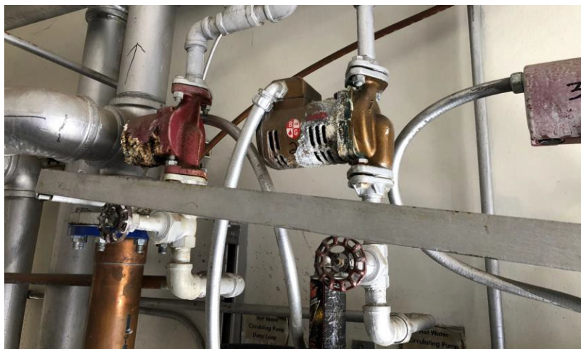
Figure 12. Existing Circulation Pumps
