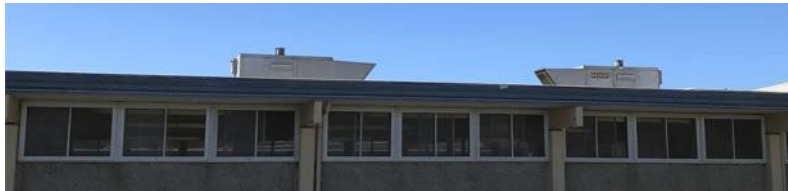
Figure 3. Typical Wing Rooftop Furnaces
