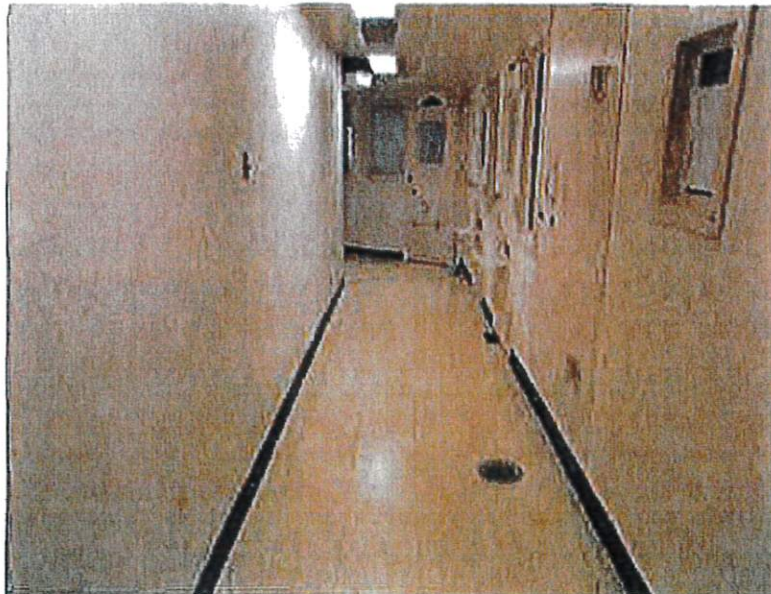
Women's Housing V Pod – Holding cells cannot be observed from a central location.
