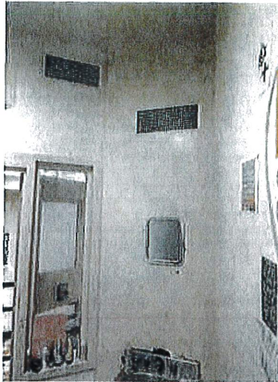
Women's Housing R and S Pod – Upper level cell mechanical grills in cells have excessive openings.
