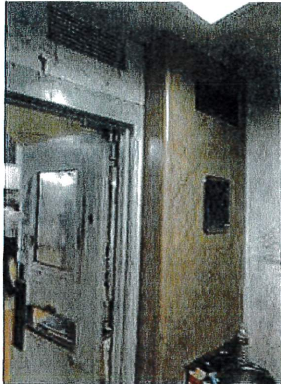
Men's Housing A and B Pod – Mechanical grills in cells have excessive openings. Return air grill is on the right in photograph.
