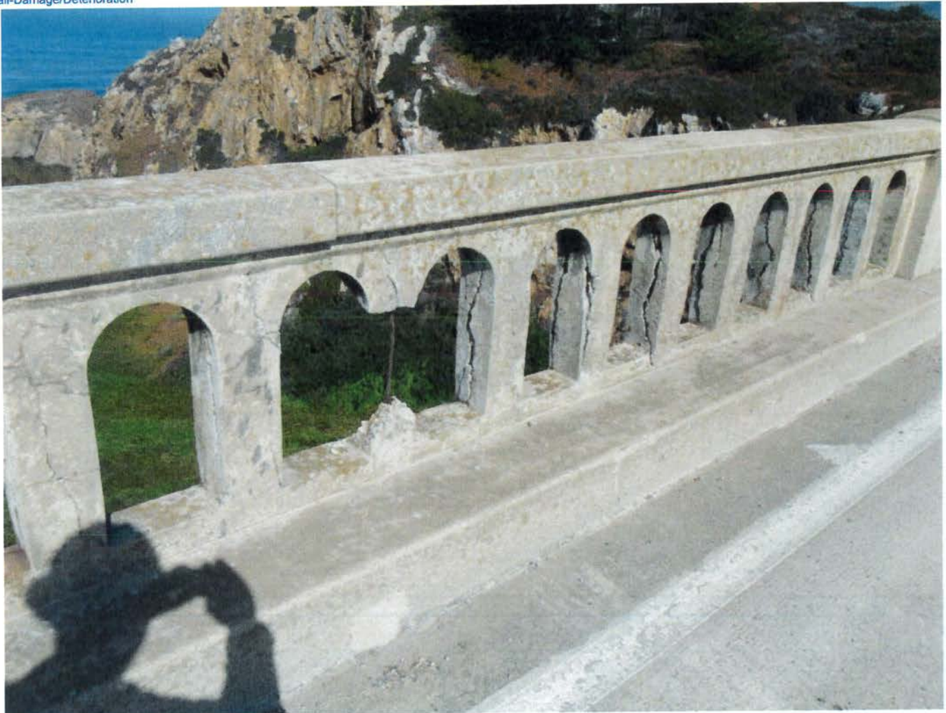
Photo #4 Gross deterioration of bridge railing.
