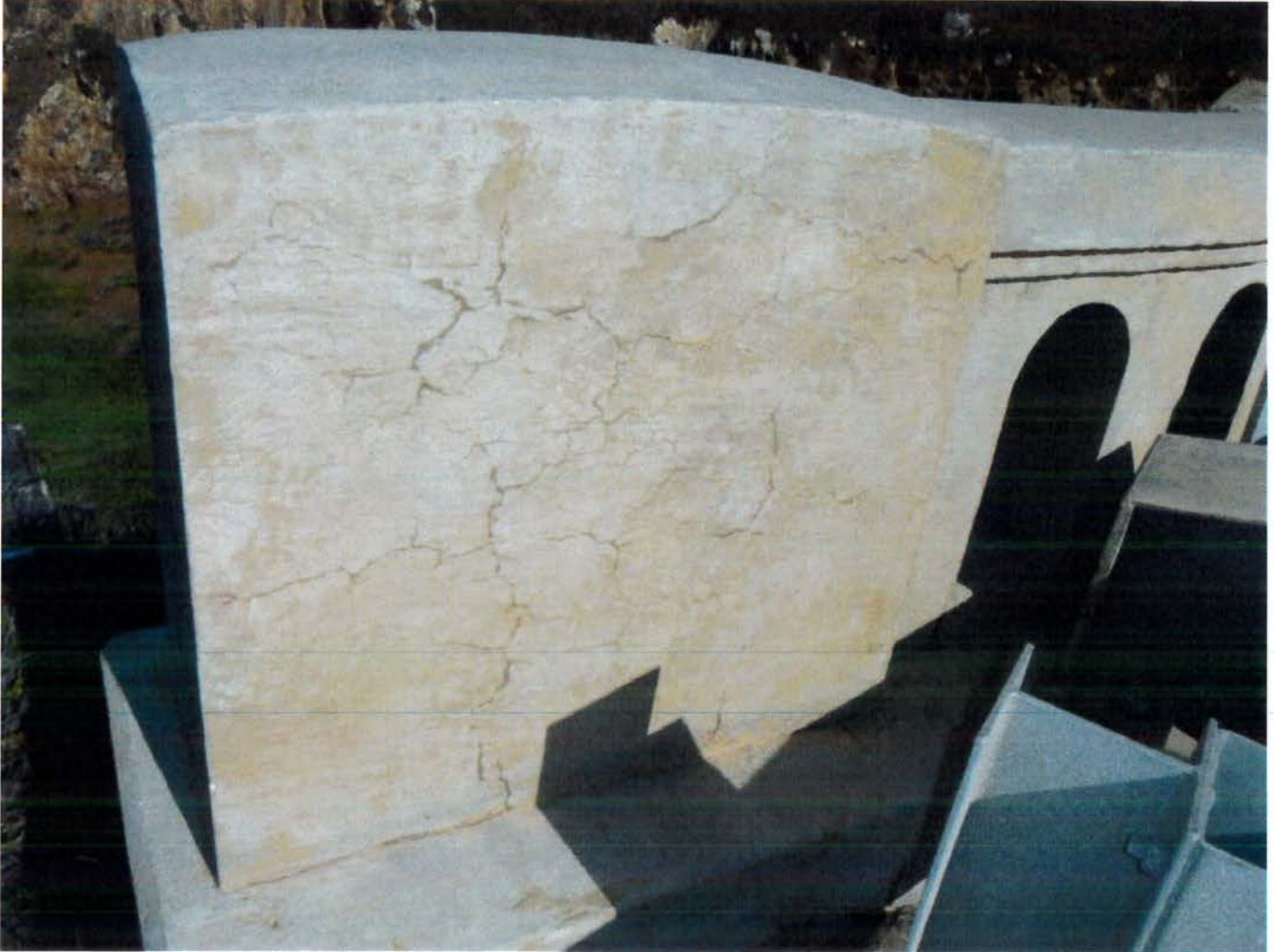
Photo #3 Pattern cracking on bridge rail end posts.
