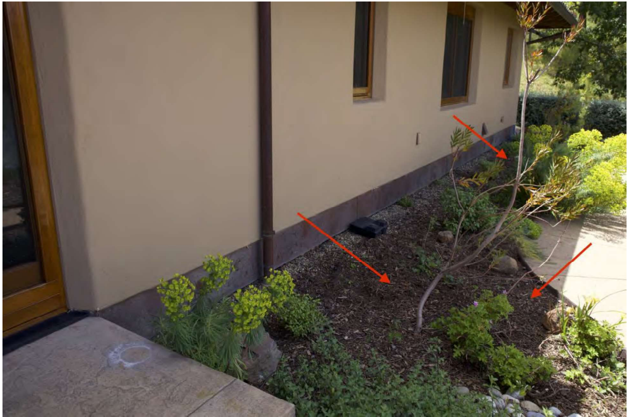
FIGURE 11. MAINTAIN SPACE BETWEEN PLANTINGS, AVOID USING WOOD CHIP MULCH AND REGULARLY REMOVE LEAF LITTER FROM THE LANDSCAPE ZONE (PHOTO NOT OF LOT 119).
