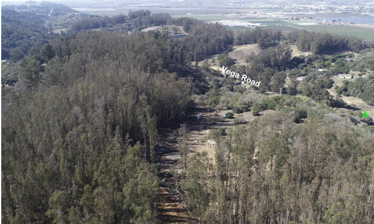
Figure 14: Westward-looking aerial oblique taken in October 2021 by R. Storesund showing site work consisting primarily of eucalyptus removal via pre-existing access roads.
