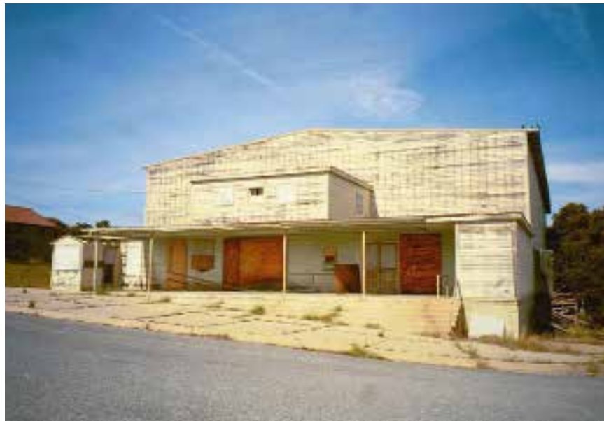
The simplicity of porches at the East Garrison is reflective of the utilitarian nature of the East Garrison buildings and should be maintained.
