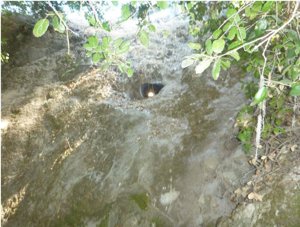
019 Photograph 20. Curb beneath lake Acirento. Note the curb appears partially collapsed but is open.
