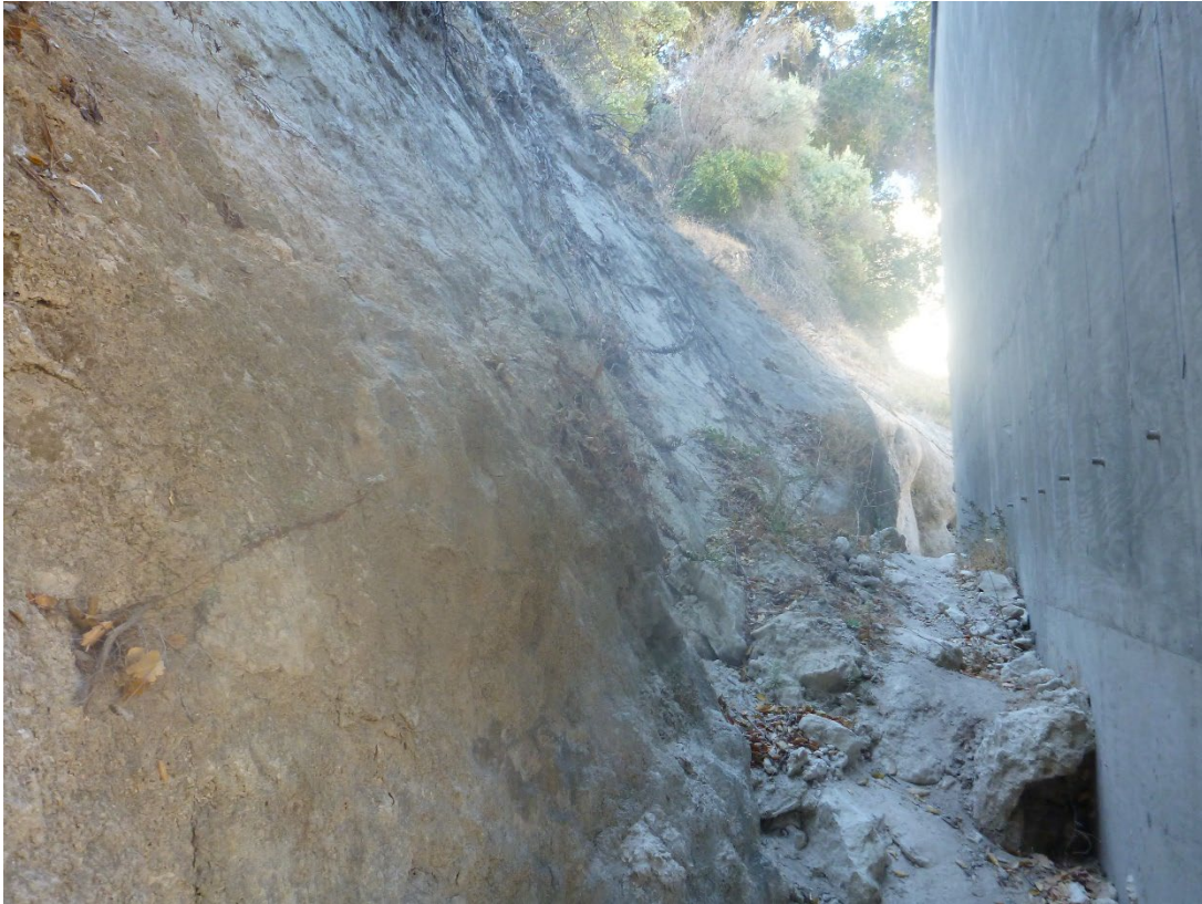
019 Photograph 019. Disformant type failure behind Powerhouse.
