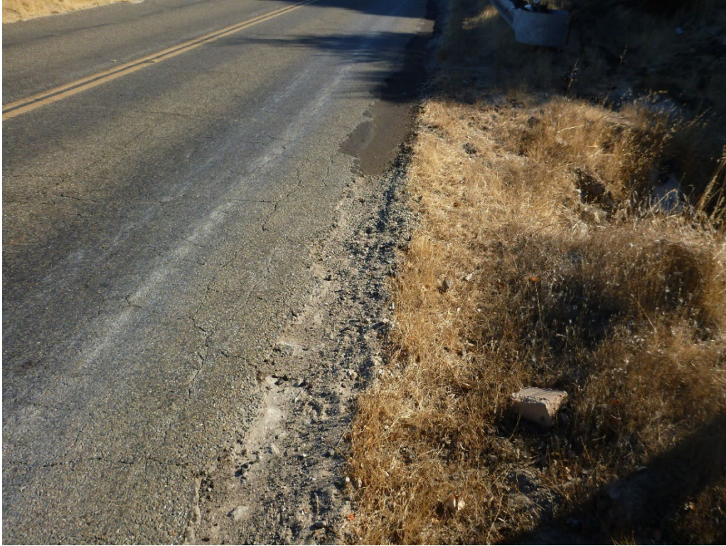
019 Photograph 1.5.19 along inside edge of roadway. Note minor cracks and asphalt patch in upper right.
