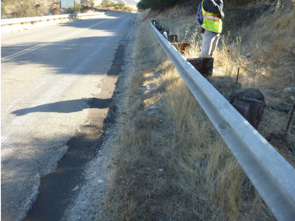
019 Photograph 14. What patch in area of erosion along inside edge of road.
