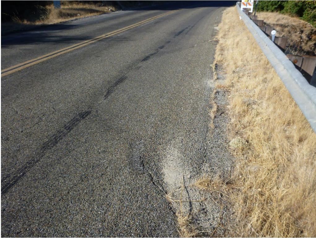
019 Photograph 15. Acuate crack in roadway is not attempt. New weeds growing in cracks
