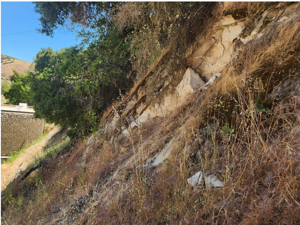
020 Photograph 020. Root in dimension back failure since 019. Failure occurred in planar bedding abng bedding. Trees appear to be leaning down slope slightly more than observed in 019
