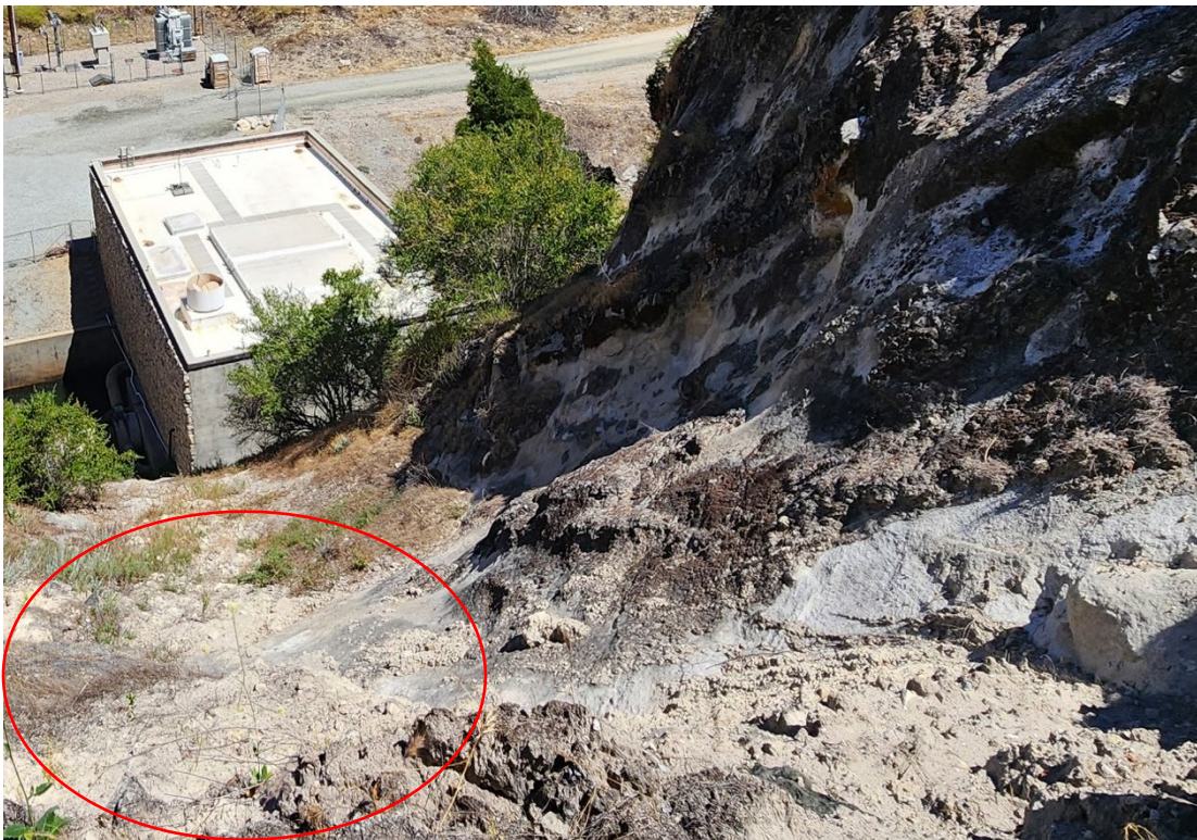
02 Photograph 21 March 2019. Shear of new wall debris bar at (circled)
