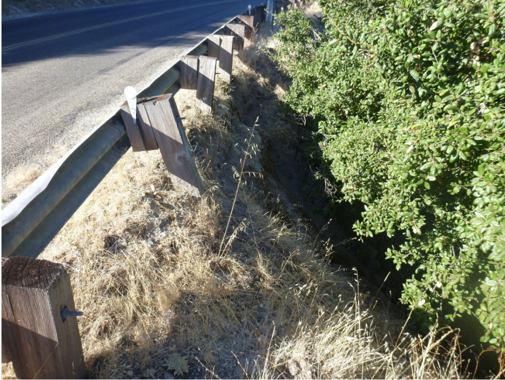
019 Photograph 21. Guardrail posts undermined at head of gulch cut at outfall.
