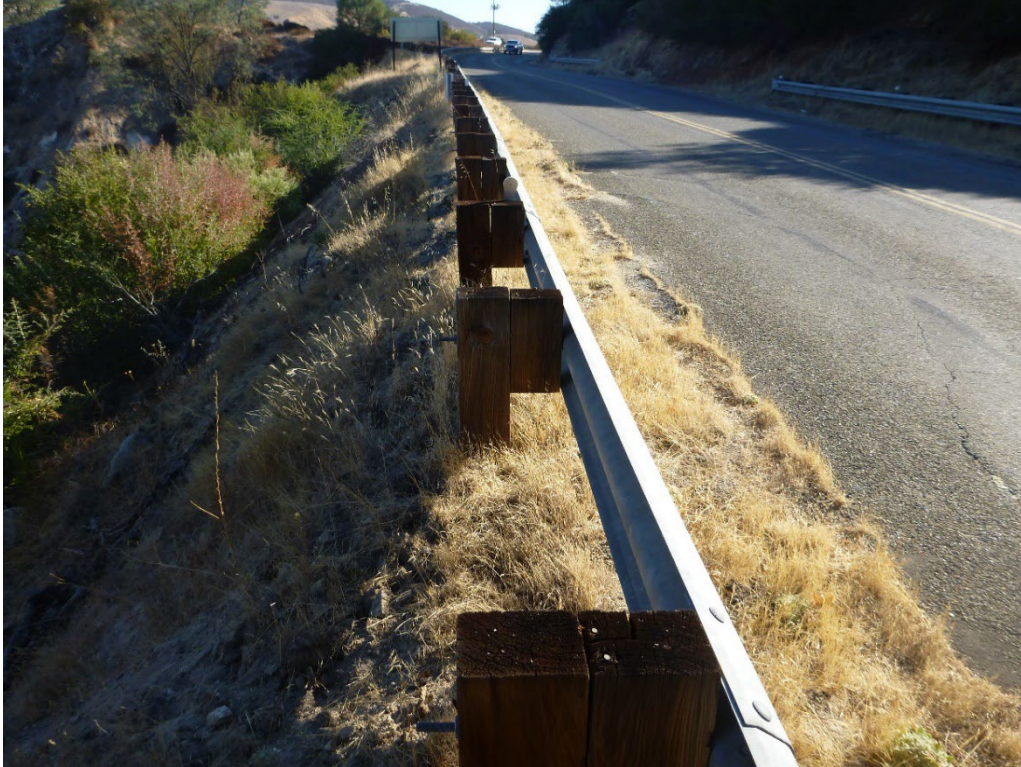
019 Photograph 16 Same area as in Photograph 15 but straight guardrail posts .
