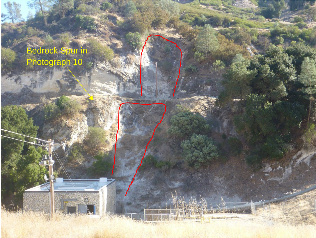
019 Photograph 1. Spesabito Powerhouse showing the abutment (red line) that failed in 19
