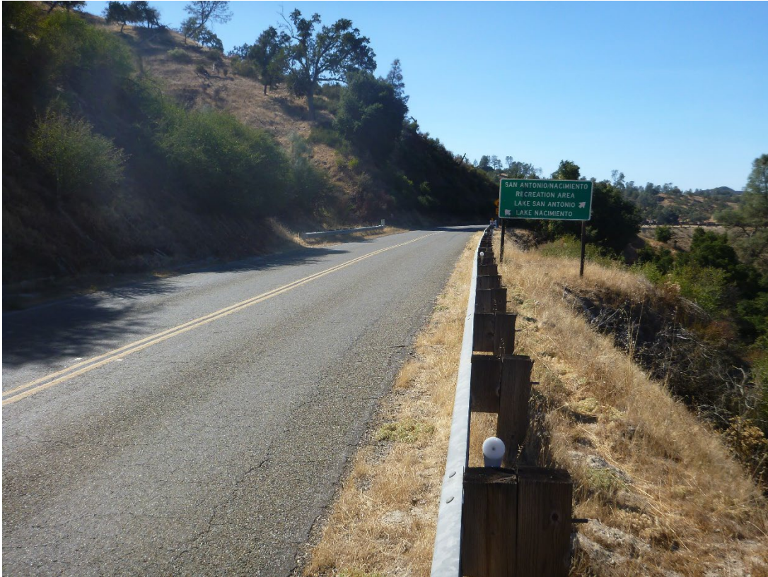
019 Photograph 120 General condition of road showing minor cracks.
