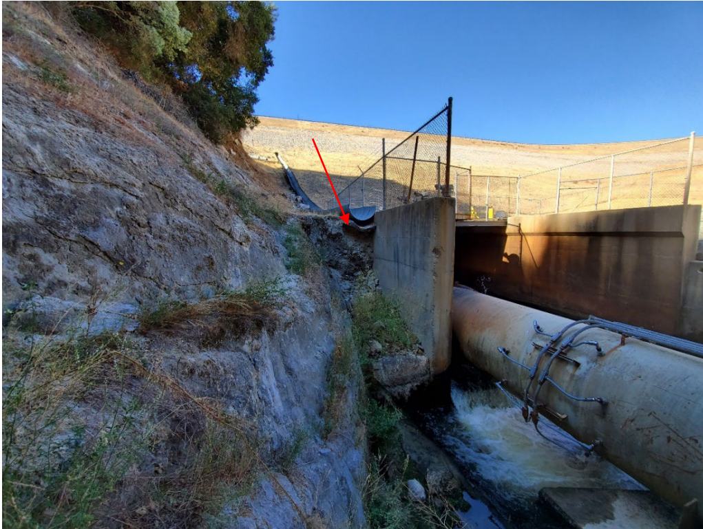
019 Photograph 3. A pipe at bottom of embankment and exposed penstock. The half-round pipe and erosion of the backfill
