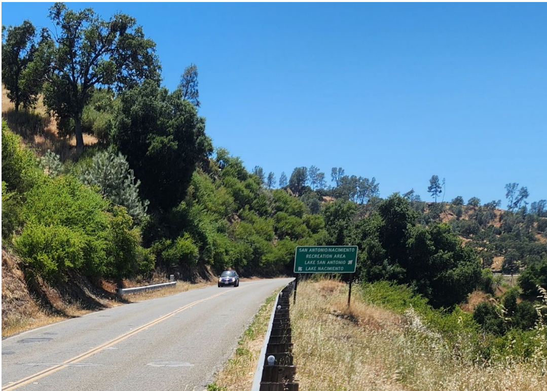
020 Photograph 121 Road patch repairs since 019. Marginal difference in overall road condition.
