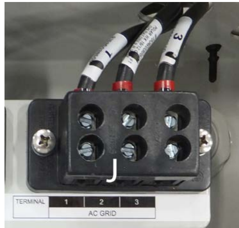
Figure 3-18: Bottom switch AC grid terminal
