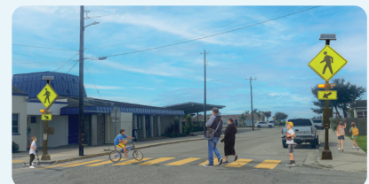
Rectangular Rapid Flashing Beacons at crosswalk across Union Street at McDougall Street
