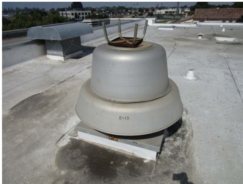
Rooftop exhaust fan to be removed and/or abandoned.
