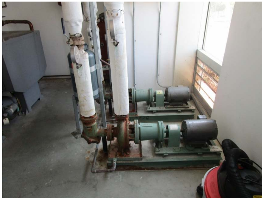
Recirculation pumps are at the end of their expected useful lives.
