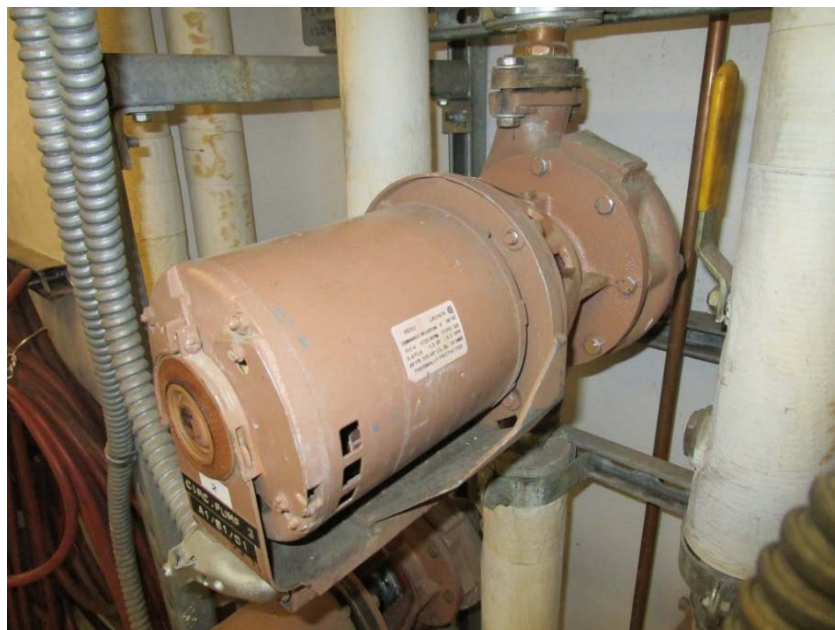
Circulating pumps are at the end of their expected useful lives.
