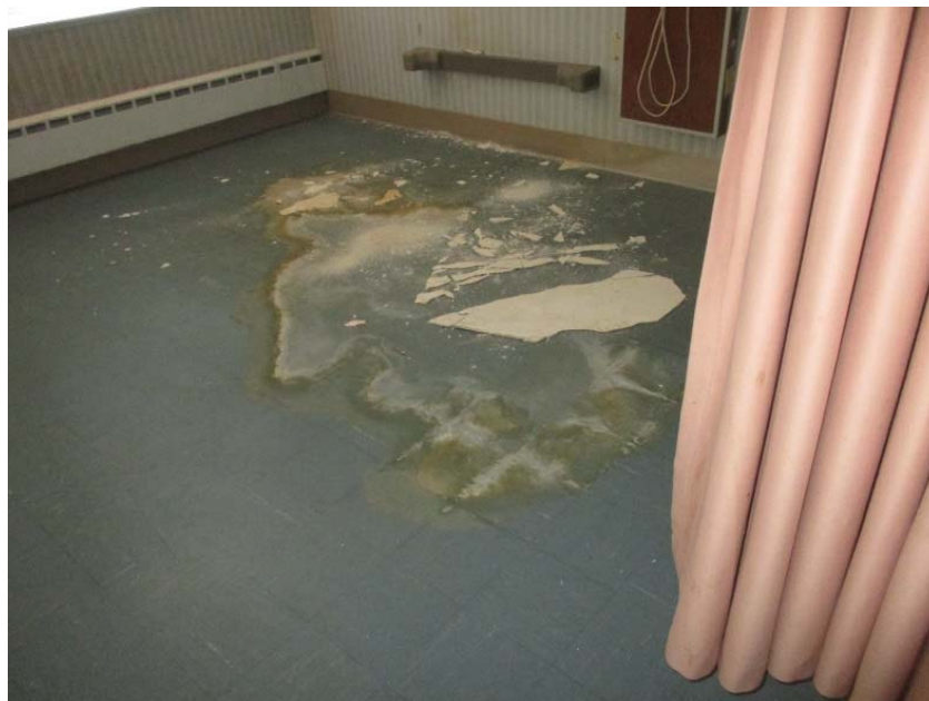
Typical floor damage at patient rooms
