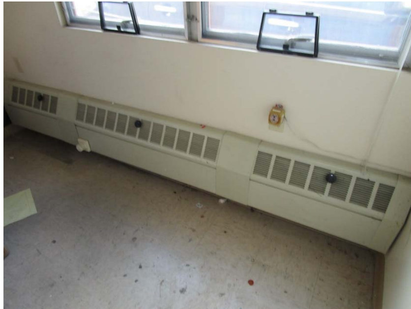
Baseboard heater is at the end of its expected useful life.
