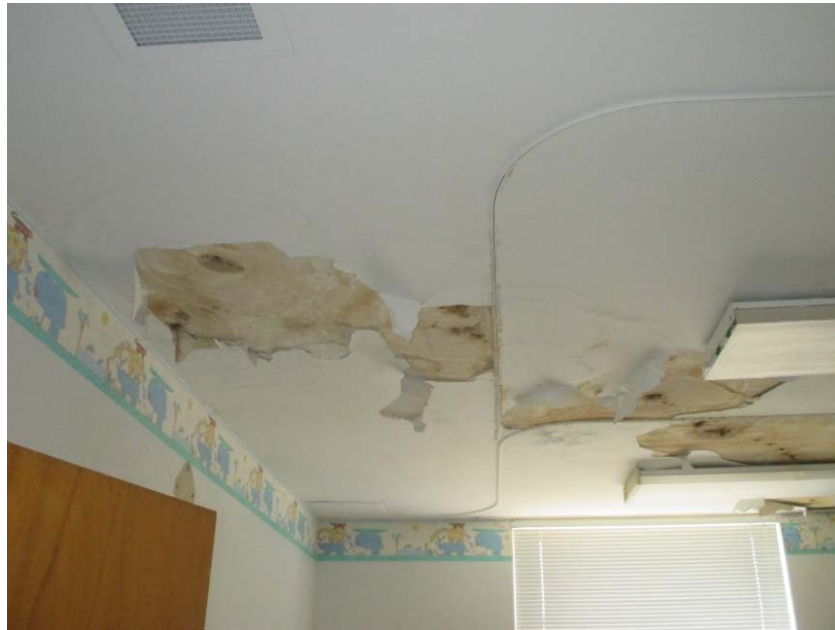
Typical ceiling damage at gypsum ceiling in patient rooms
