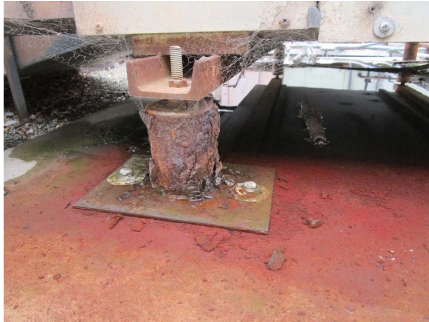
Standing water on the roof is causing the mounts to rot away. Suggest installing a 4" curb for both HVAC units to mitigate this.
