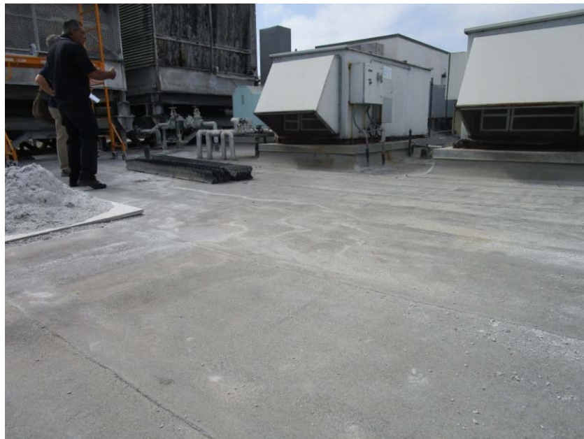
Make-up air handling units pulls in calcium deposits from the cooling towers and contaminates the air and food in the kitchen.
