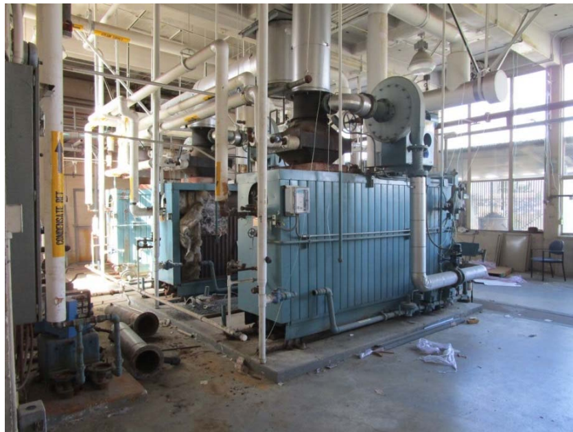
Heating hot water boilers are in poor condition and will need to be replaced.
