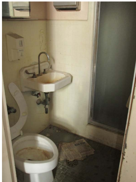
Plumbing system and plumbing fixtures are at the end of their expected useful lives.
