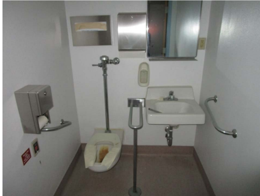
Plumbing system and plumbing fixtures are at the end of their expected useful life.
