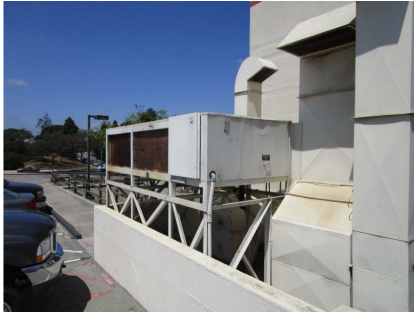
Packaged DX cooling with gas heating air conditioning unit is at the end of its expected useful life.
