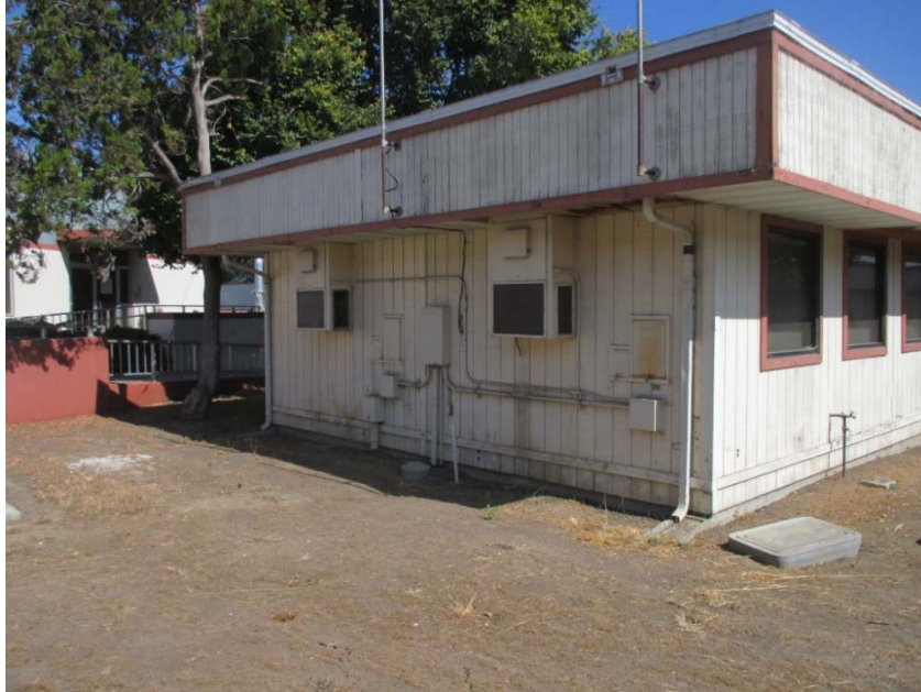
Typical deteriorated plywood siding.
