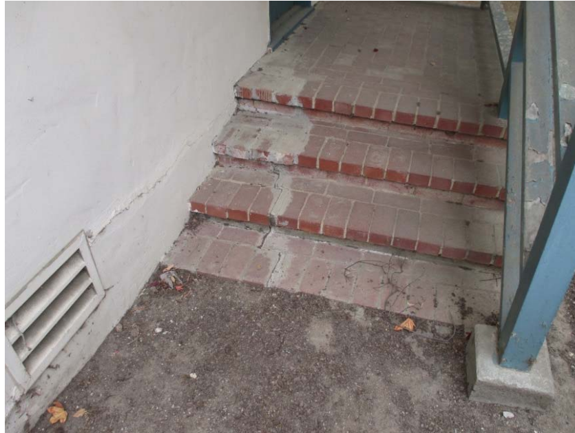
Exterior steps require correction
