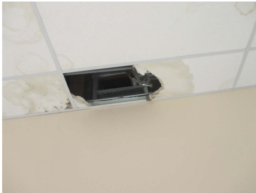
Damaged ceiling tiles
