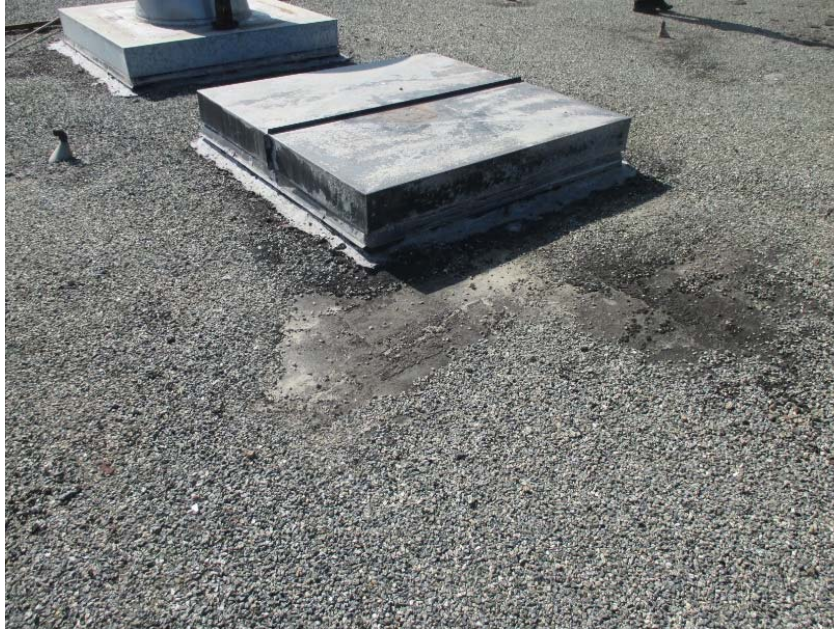
Worn gravel roof
