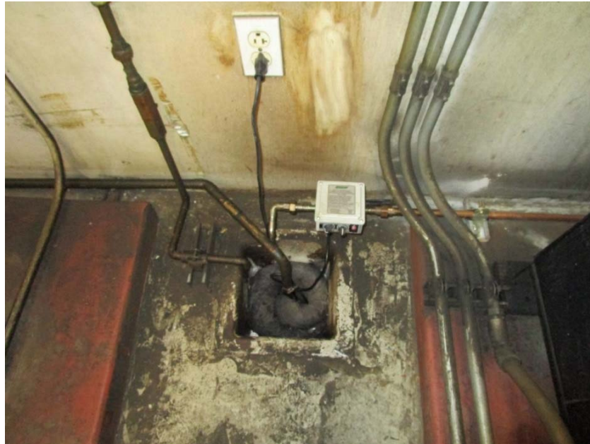
Condensate pump is at the end of its expected useful life.
