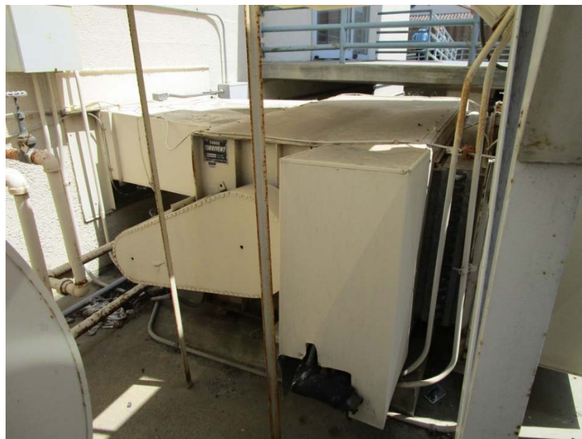
Heating and ventilation unit is at the end of its expected useful life.
