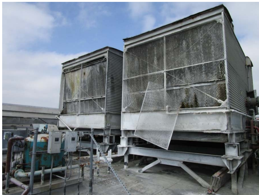
Cooling towers are in poor condition and will need to be replaced.
