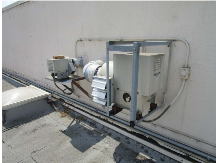
Utility exhaust fan is at the end of its expected useful life.
