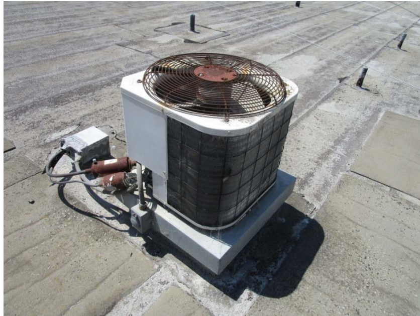
Split air conditioning systems with outdoor condensing units and indoor fan coil units are at the end of their expected useful lives.
