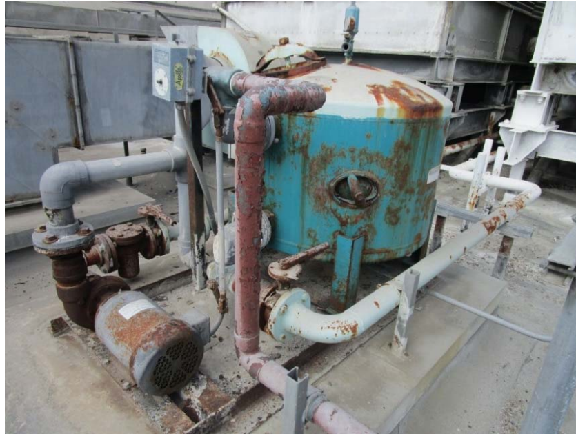
Rooftop sand filter is no longer working and will need to be replaced.
