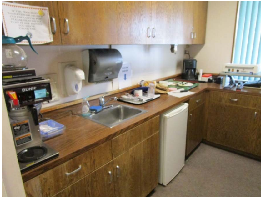
Plumbing system and plumbing fixtures are the end of their expected useful lives.
