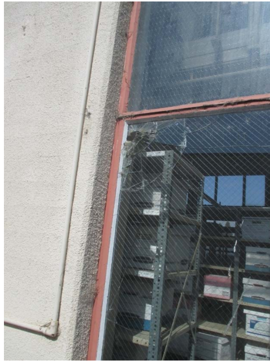
Damaged window frame / glazing
