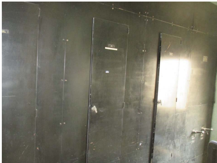
The panelboards are past their expected useful lives.
