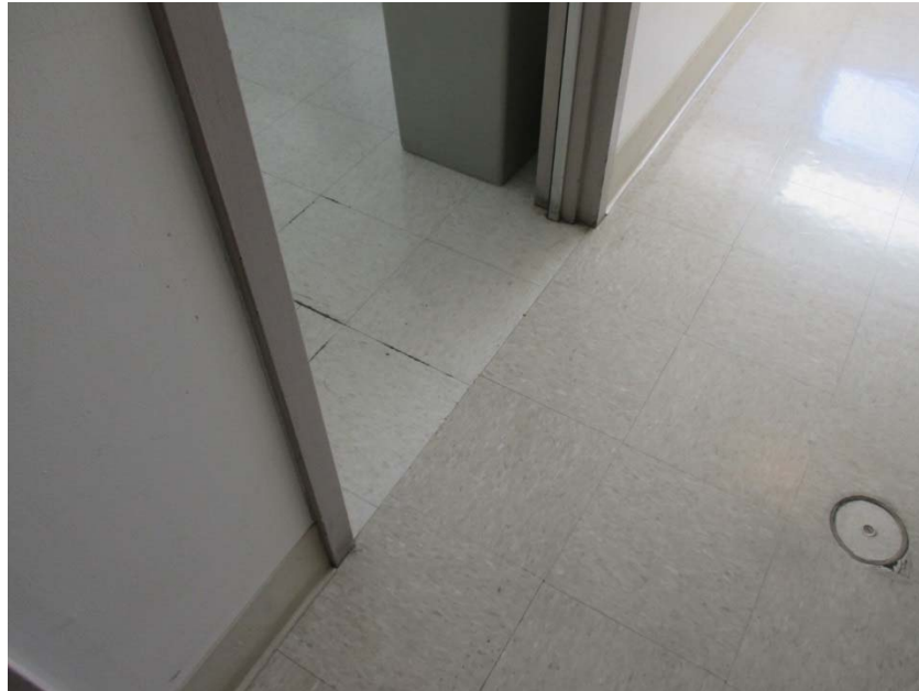
VCT flooring is failing
