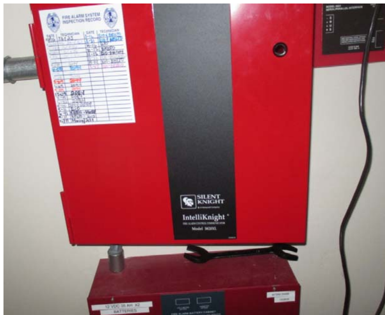
The fire alarm is past its expected useful life.
