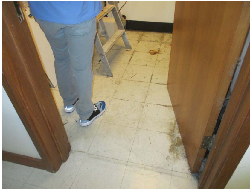
Failing VCT flooring
