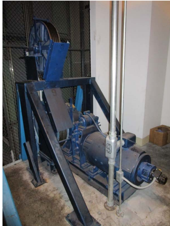
Elevator motors frequently go down and will eventually need to be replaced.
