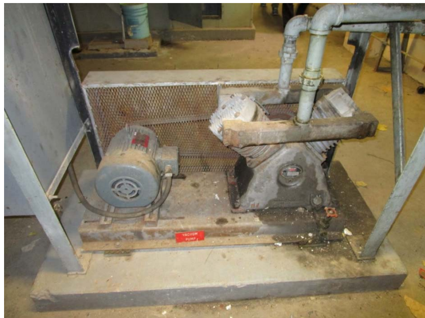
Vacuum pump system is at the end of its expected useful life.
