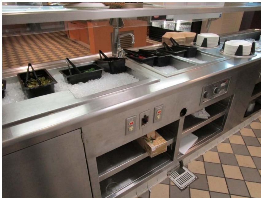
The food service equipment located in the kitchen are at the end of their expected useful lives.
