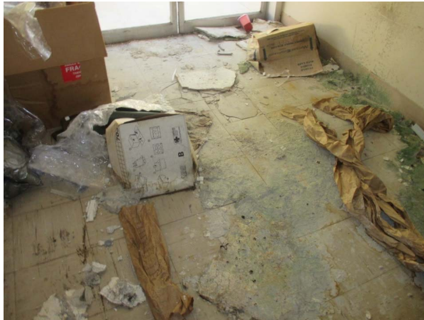
Floor tile is damaged, debris present.
