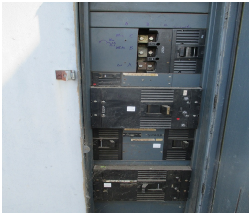
The main switchboard is past its expected useful life.
