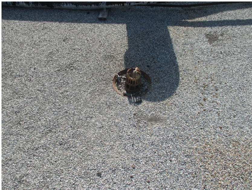
Damaged roof drain
