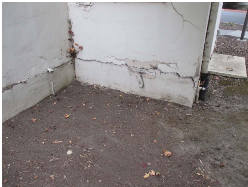
Failing cement plaster
