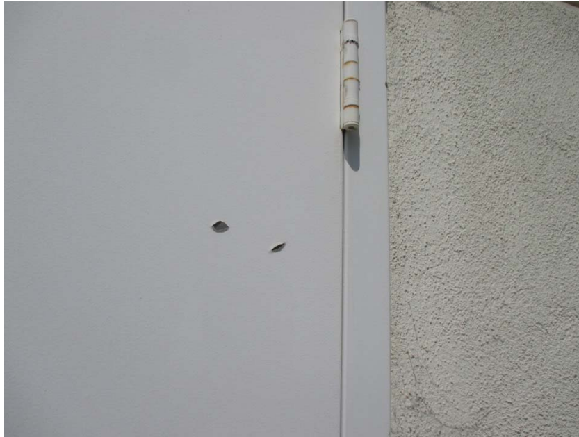
Exterior door needs paint
