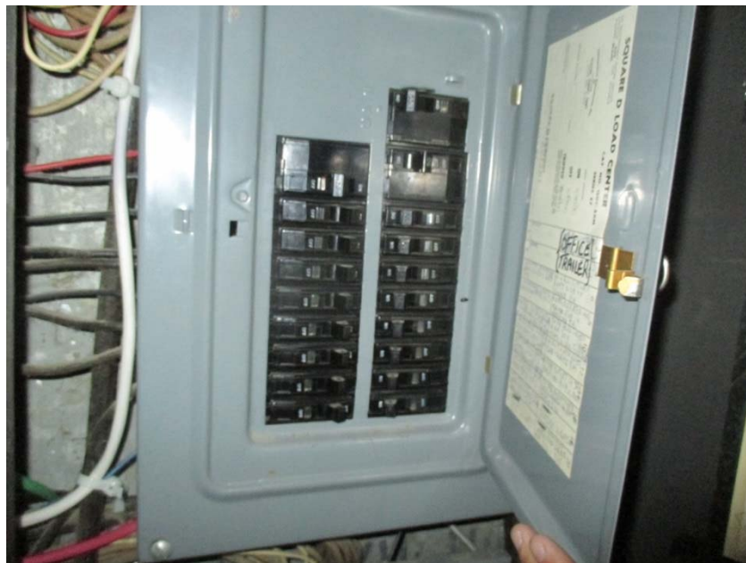
All panels are past their expected useful lives.
