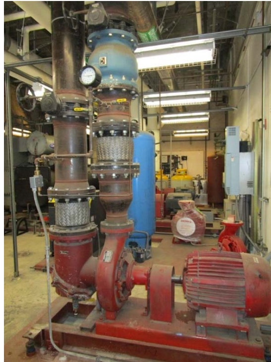
Condenser water pumps are at the end of their expected useful lives.
