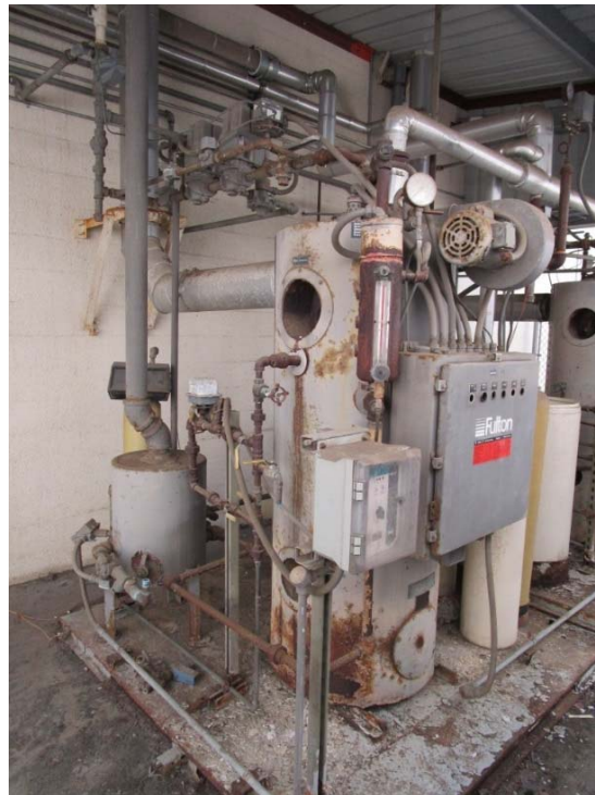
Heating hot water boilers are at the end of their expected useful lives.
