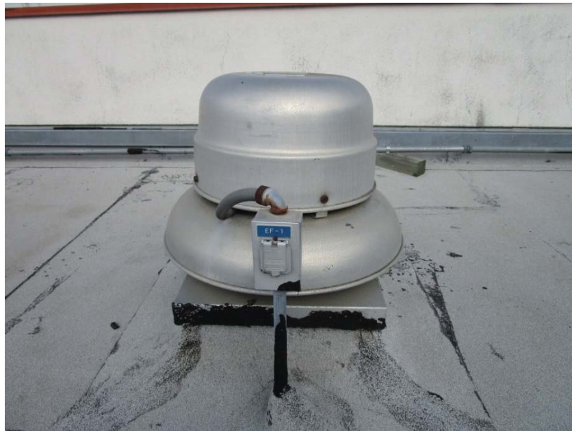
Rooftop exhaust fan is at the end of its expected useful life.
