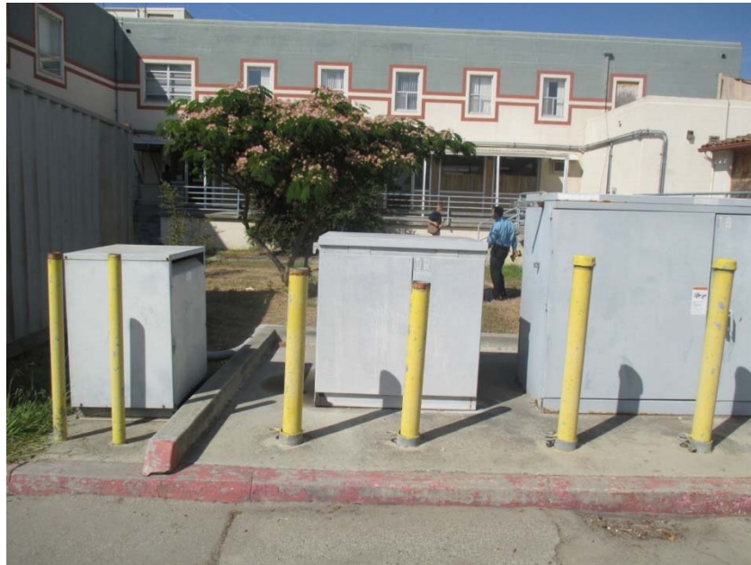
Two transformers are past their expected useful lives.
