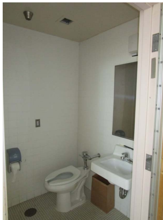
The plumbing system and plumbing fixtures are at the end of their expected useful lives.
