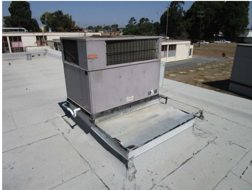
Building 840 packaged rooftop DX cooling with gas heating air conditioning units are at the end of their expected useful lives.
