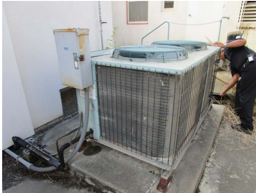
Ground mounted heat pump unit is at the end of its expected useful life.
