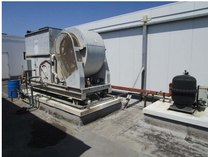
Cooling tower and sand filter are not working and will need to be replaced.
