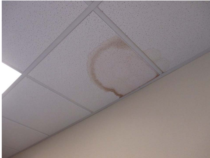
Stained ceiling tiles
