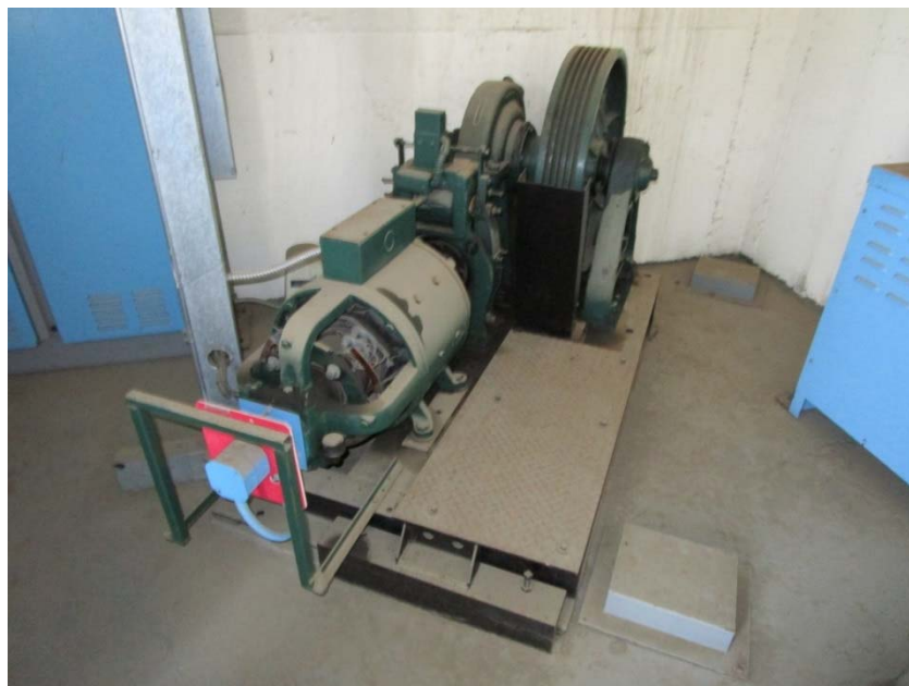
Elevator motor is at the end of its expected useful life.
