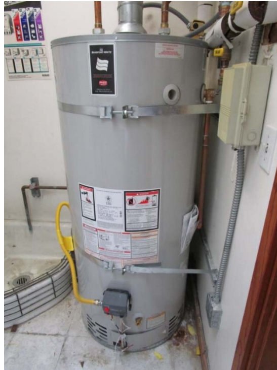
Gas water heater is at the end of its expected useful life.
