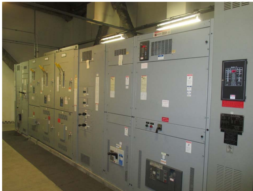
The main switchboards have reached the end of their expected useful lives.
