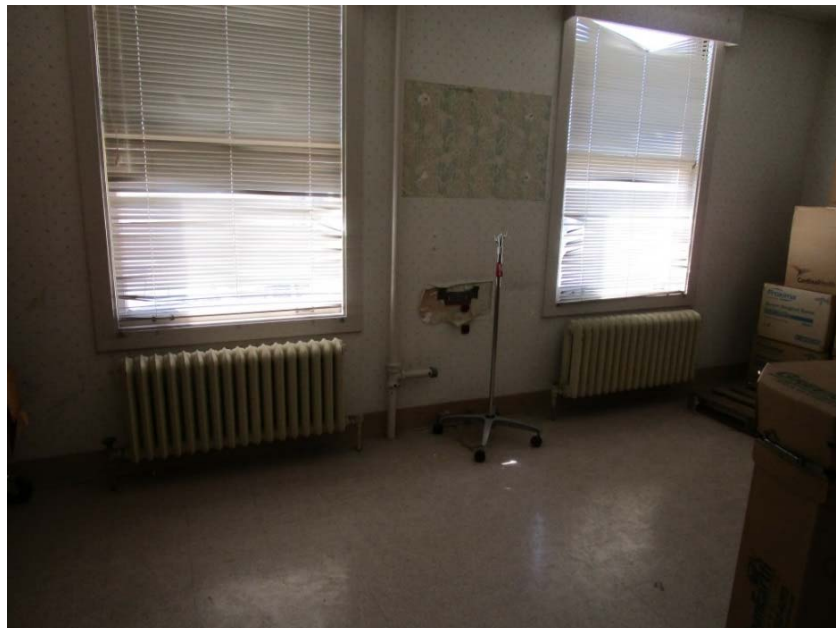
Radiant wall heaters are at the end of their expected useful lives.
