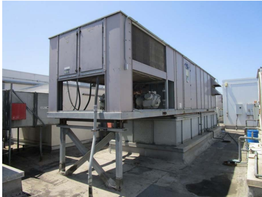
Rooftop AHUs are at the end of their expected useful lives.
