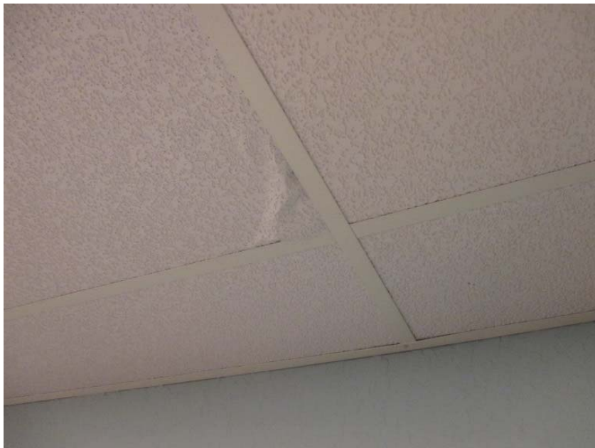
Typical ceiling tile needing replacement
