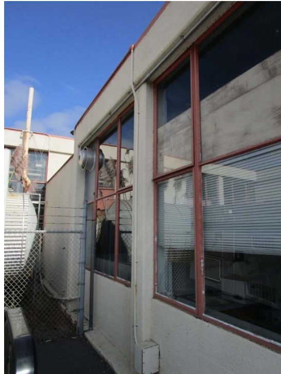
Sidewall exhaust fan is at the end of its expected useful life.
