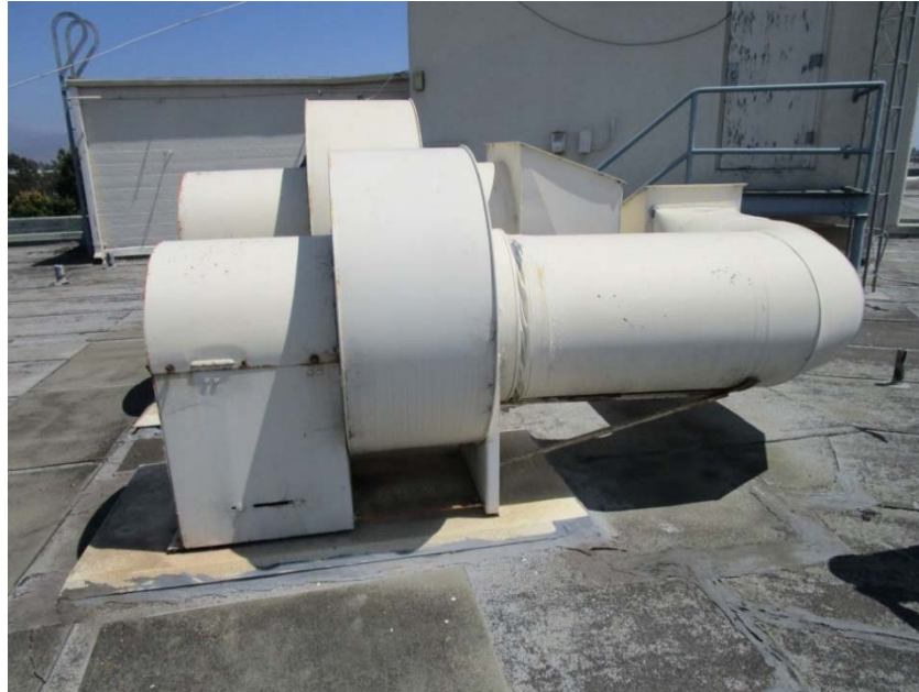
Utility exhaust fan is at the end of its expected useful life.
