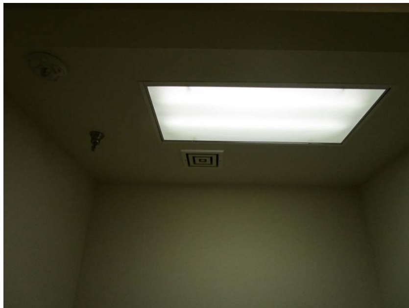
Buildings 840 and 870 ceiling exhaust fans are at the end of their expected useful lives.
