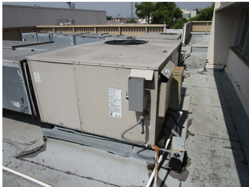
Packaged rooftop DX cooling with gas heating air conditioning unit is at the end of its expected useful life.
