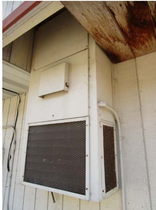
Buildings 820 and 870 Bard wall mounted AC units are at the end of their expected useful lives.
