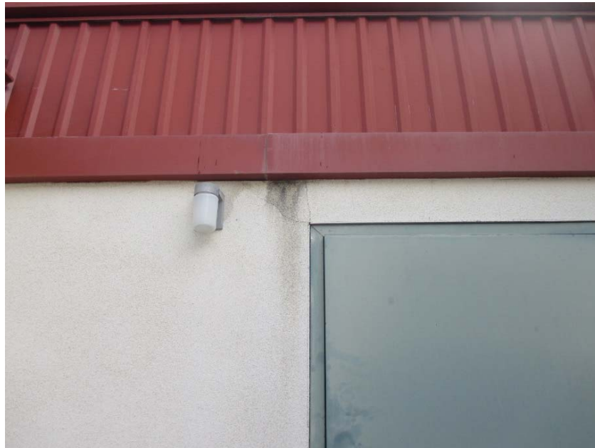
Cement plaster cracking
