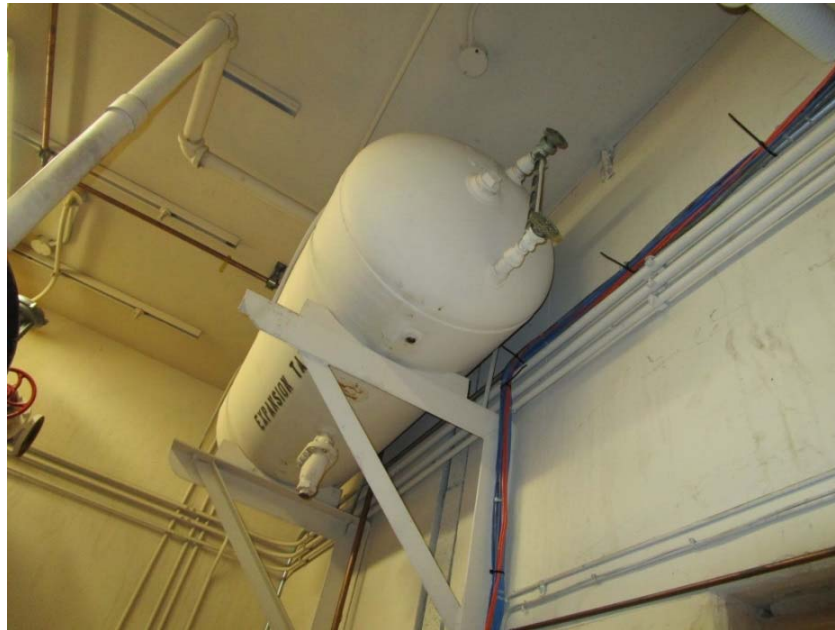
Expansion tank is at the end of its expected useful life.
