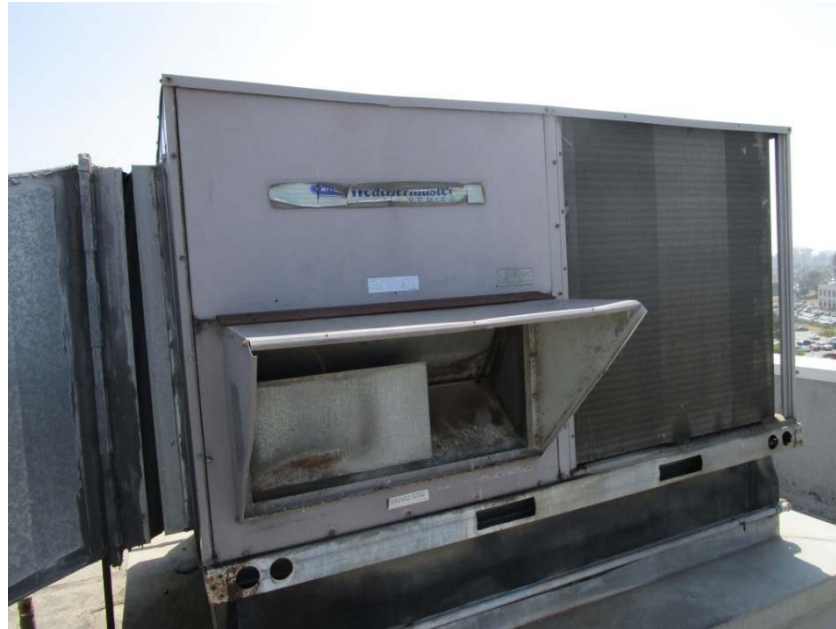
Packaged rooftop DX cooling with gas heating air conditioning unit is at the end of its expected useful life.
