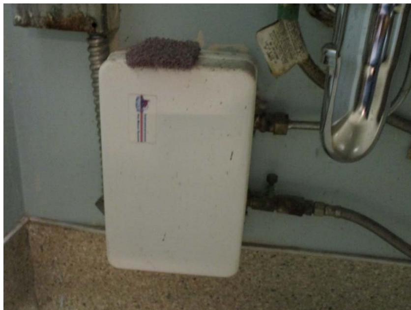
Electric instantaneous water heater is at the end of its expected useful life.
