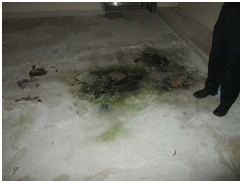
Exposed slab showing water damage / staining
