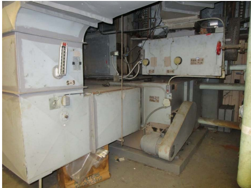
Heating hot water fan coil unit is at the end of its expected useful life.
