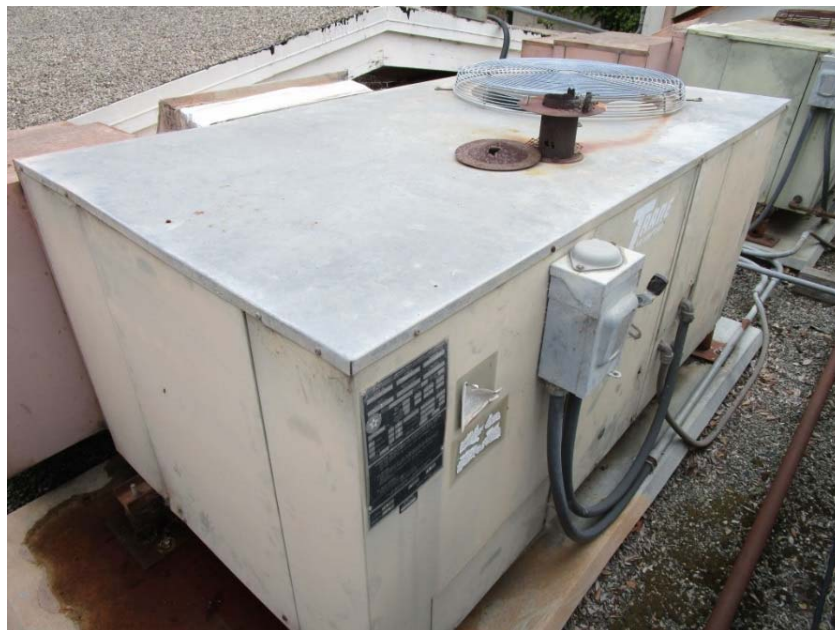
Packaged rooftop DX cooling with gas heating air conditioning unit is at the end of its expected useful life.
