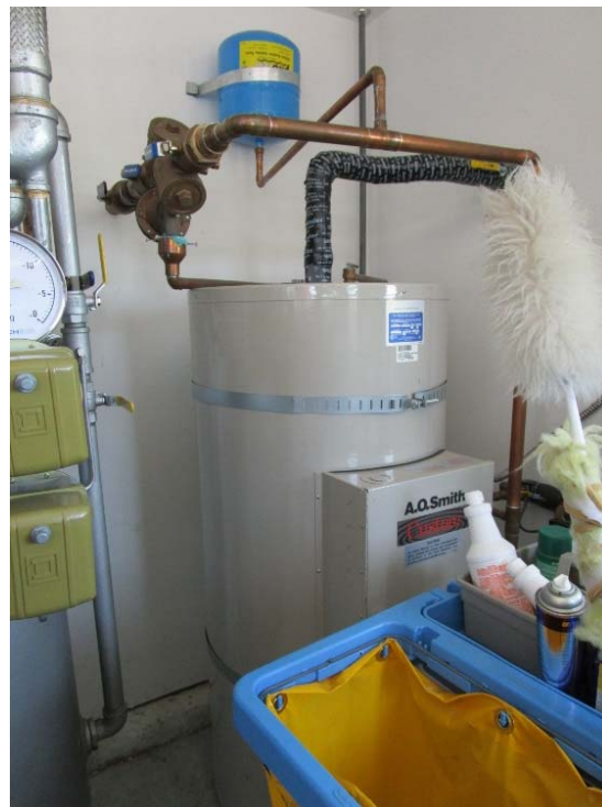
Electric water heater is at the end of its expected useful life.
