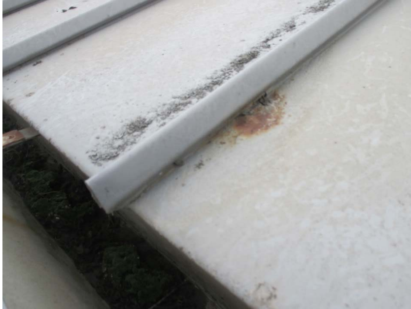
Metal roofing is rusting and starting to fail
