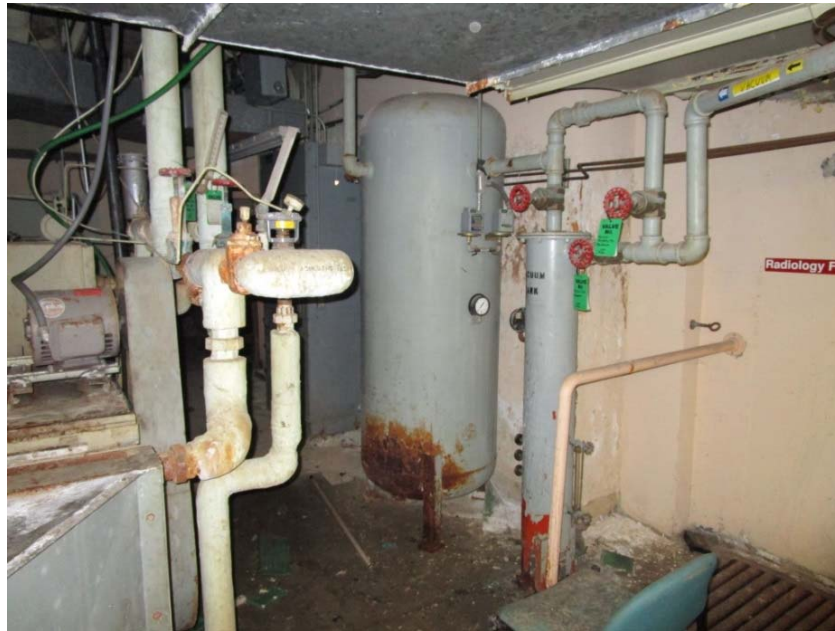
Expansion tank is in poor condition and needs to be replaced.
