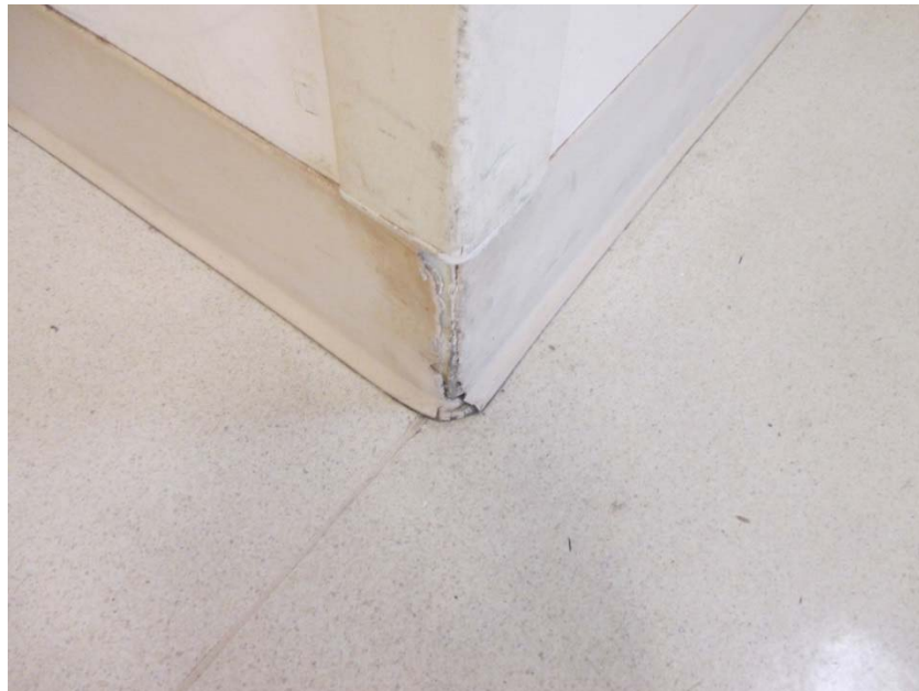
Damaged wall base.
