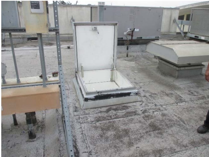
Roof hatch with no fall protection
