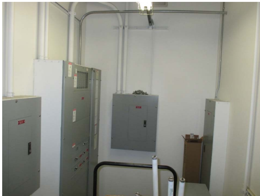
The main switchboard is approaching its expected useful life.
