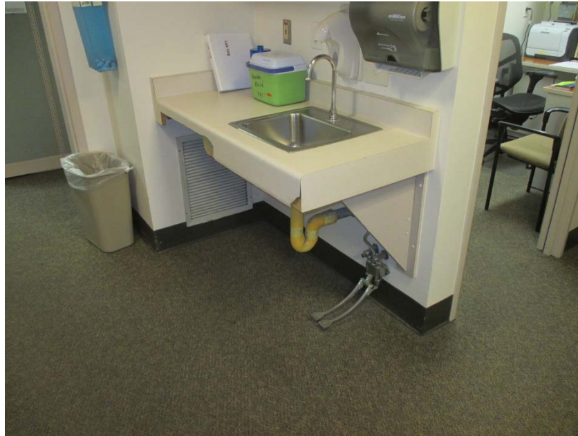
Damaged handwash station
