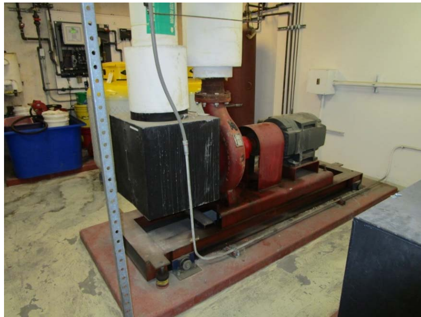
Chilled water pumps are at the end of their expected useful lives.
