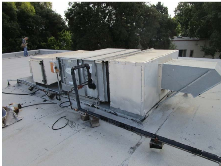
Rooftop packaged DX cooling with gas heating air conditioning unit is at the end of its expected useful life.
