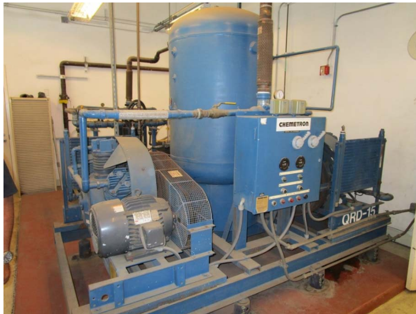
Medical air compressor system is at the end of its expected useful life.
