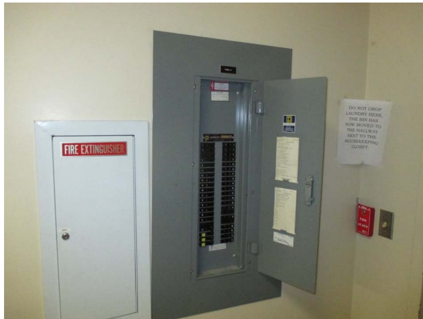
All panels are past their expected useful life.
