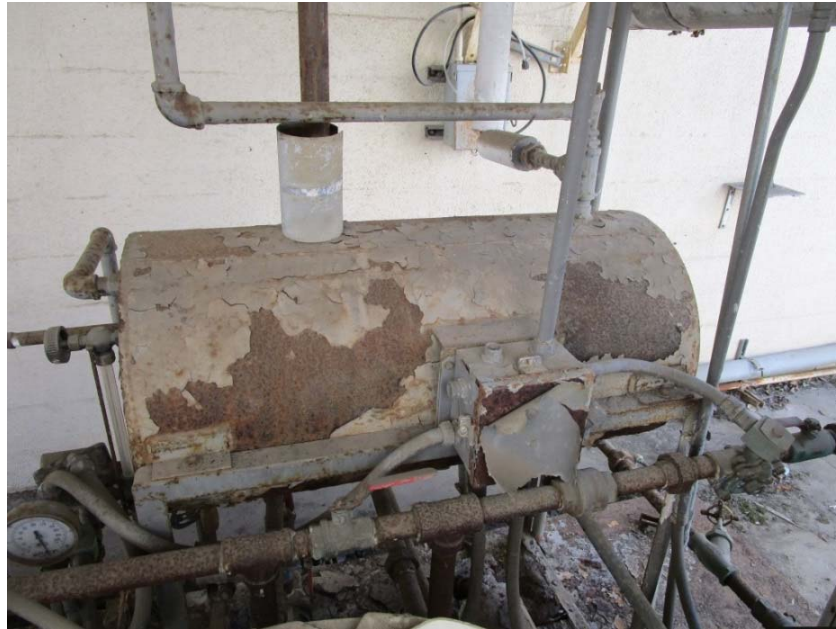
Expansion tank is in poor condition and will need to be replaced.
