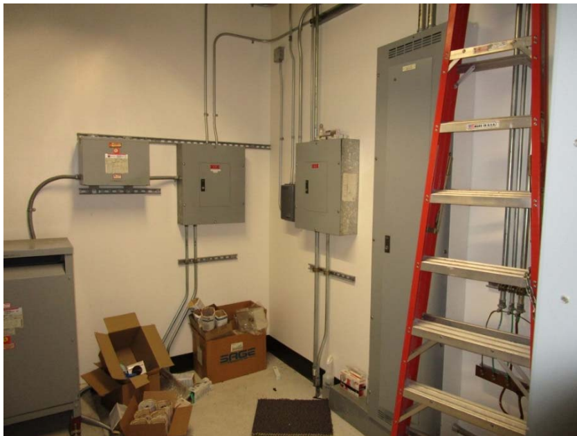
Recommend installing a new split ductless HVAC system in Electrical Room to maintain proper room temperature.
