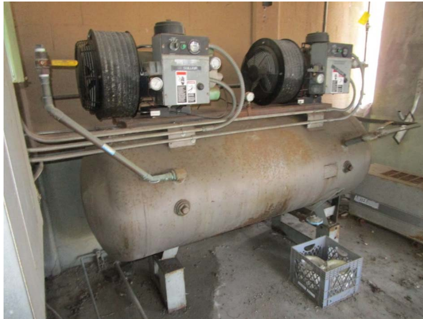
Air compressor is at the end of its expected useful life.
