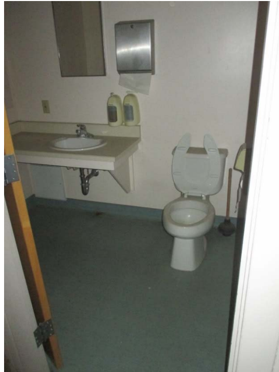
Plumbing system and plumbing fixtures are at the end of their expected useful lives.
