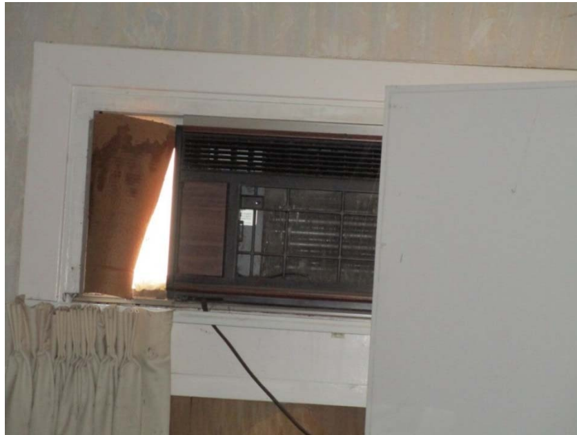
Window mounted AC unit is at the end of its expected useful life.
