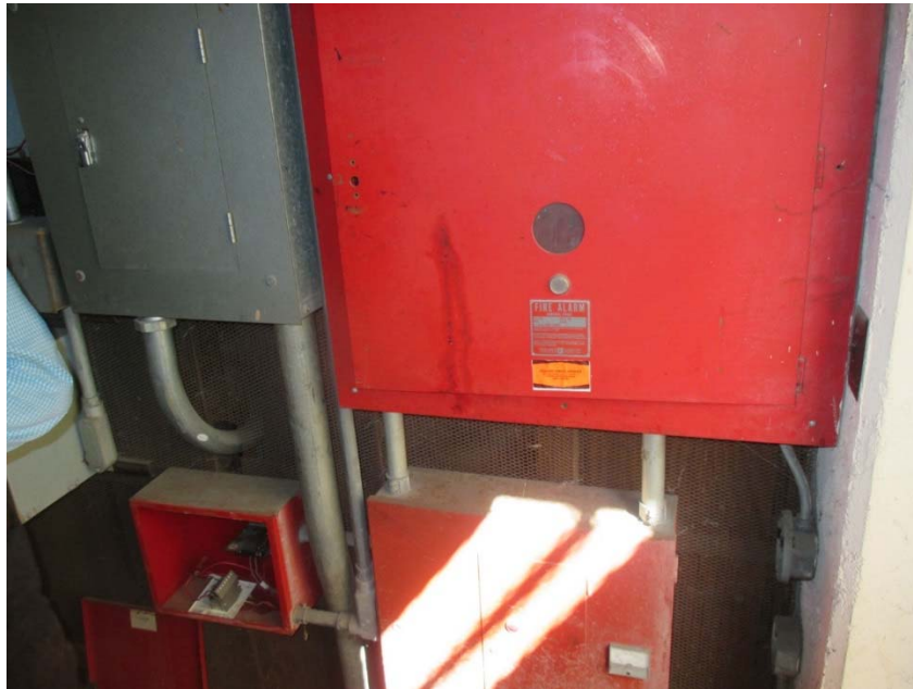
The fire alarm panel is past its expected useful life.
