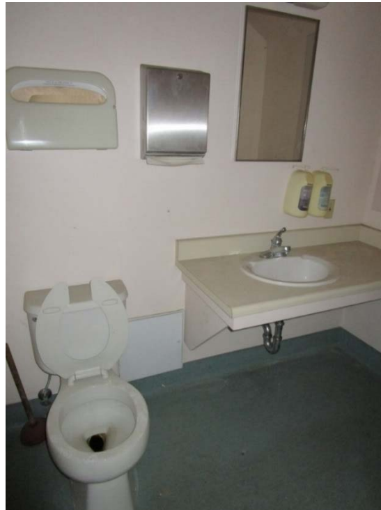
Plumbing system and plumbing fixtures are at the end of their expected useful lives.
