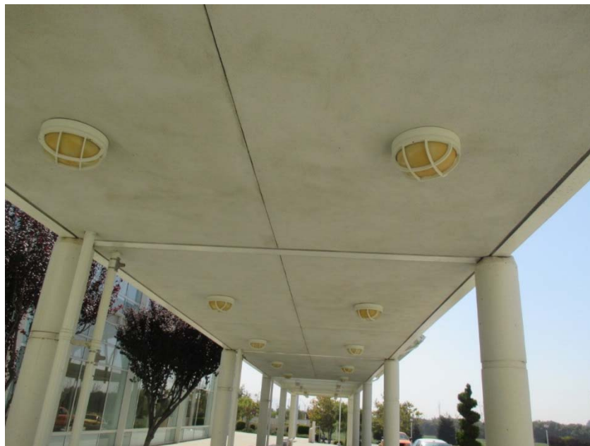
Exterior lighting fixtures are yellowing and should be replaced.
