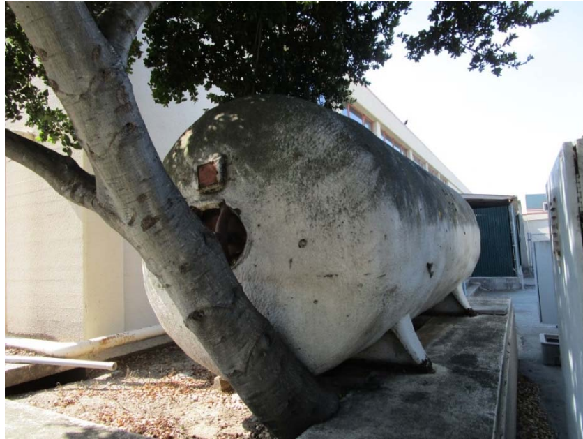
Hot water storage tank is at the end of its expected useful life.
