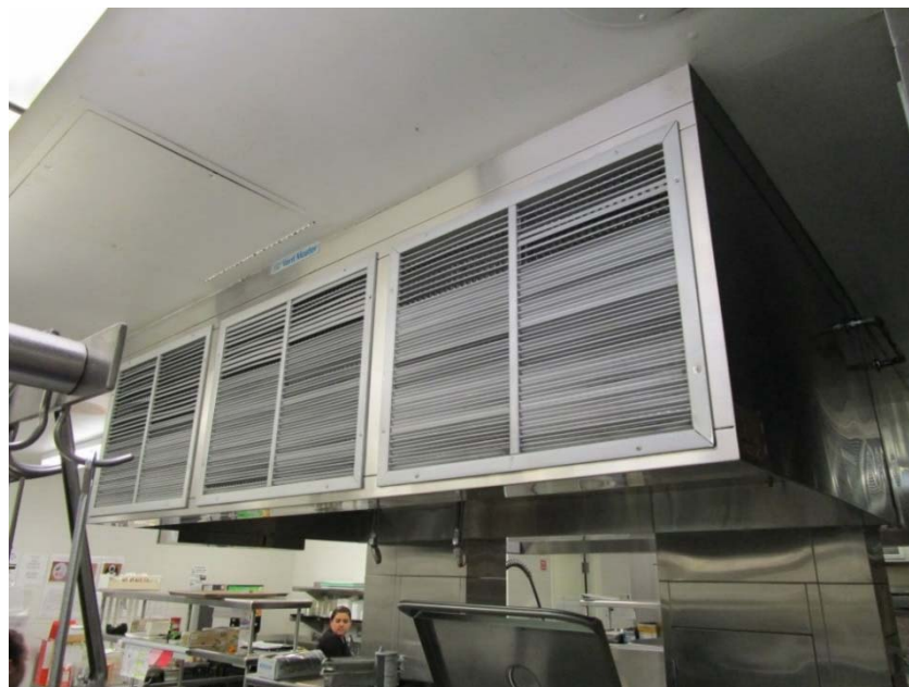
Kitchen exhaust hood with fire suppression systems are at the end of their expected useful lives.
