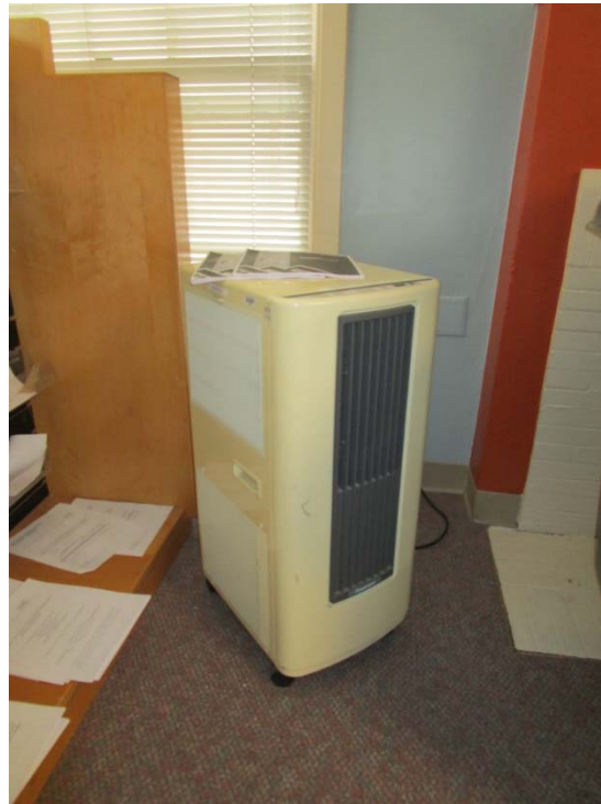
Portable air conditioning unit is at the end of its expected useful life.
