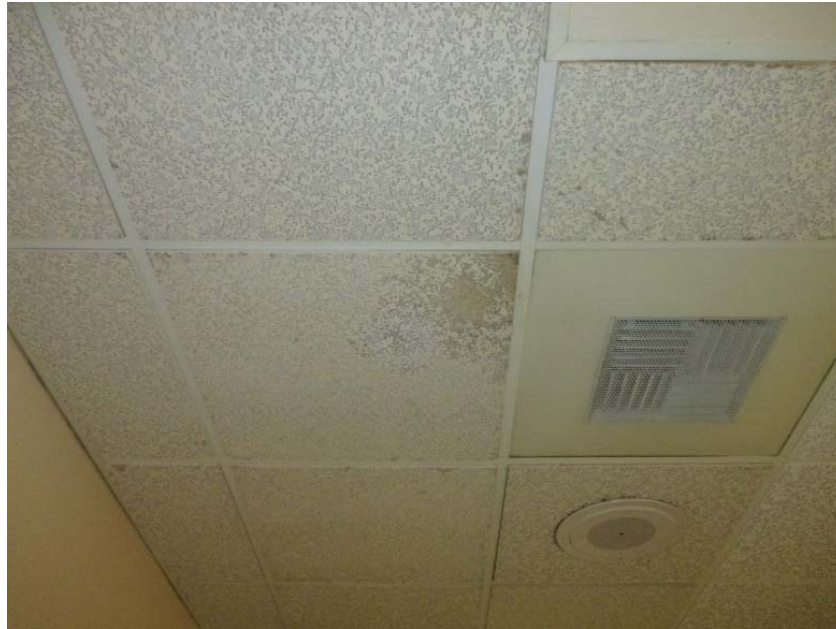
Worn ceiling tiles
