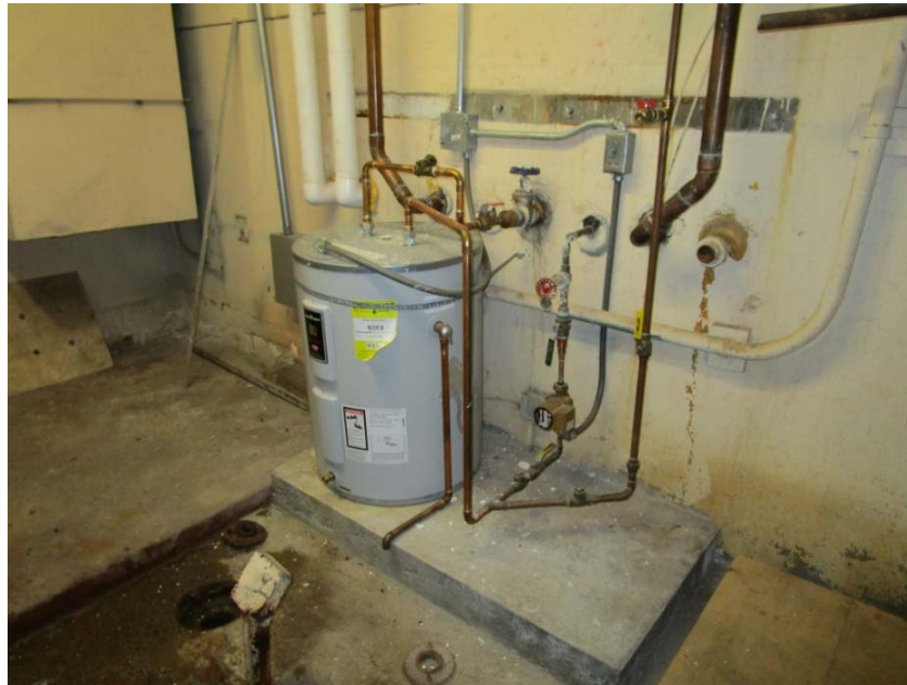
Electric water heater is at the end of its expected useful life.
