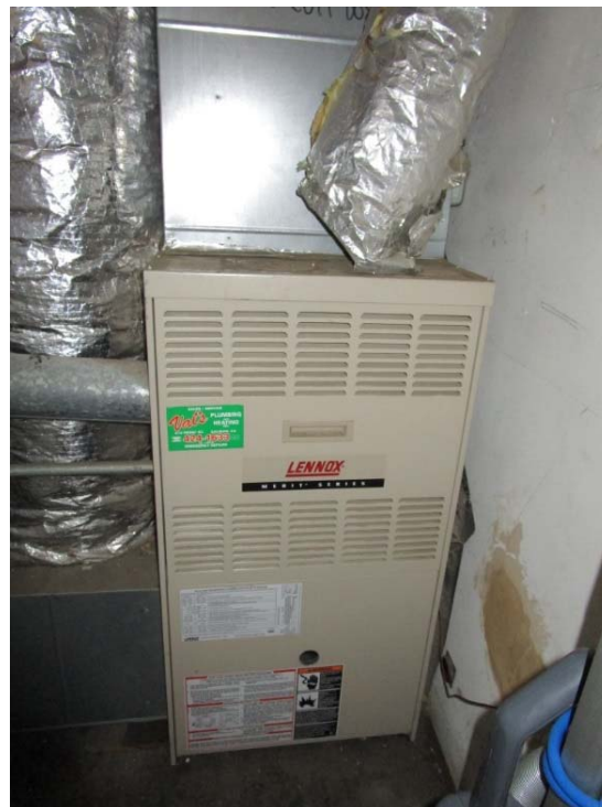
Indoor gas furnace unit is at the end of its expected useful life.
