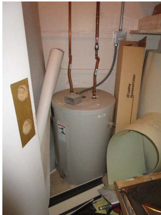
Electric water heater is at the end of its expected useful life.
