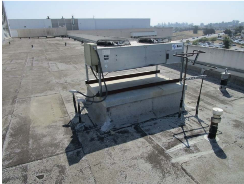
Rooftop refrigeration condensing unit and indoor evaporator for the walk-in refrigeration system is at the end of its expected useful life.
