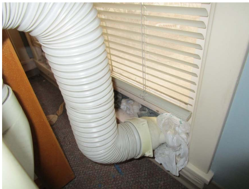
Exhaust duct for portable air conditioning unit is improperly installed.
