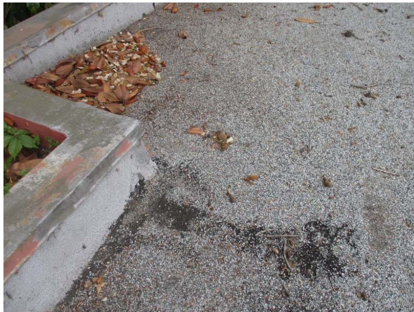
Gravel roof and parapet caps are beyond useful life
