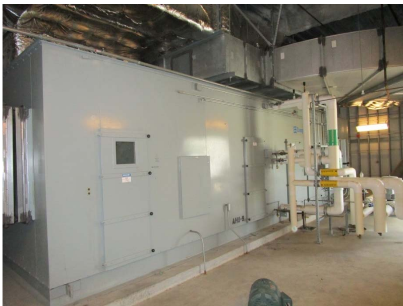
Buildings 100, 200, 300, 500 and 580 built-up AHUs are at the end of their expected useful lives.
