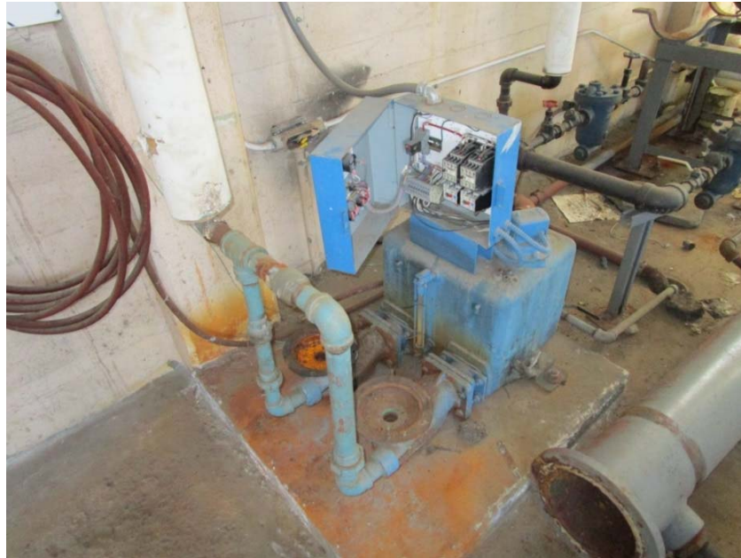
Steam condensate vacuum pump unit is in poor condition and will need to be replaced.
