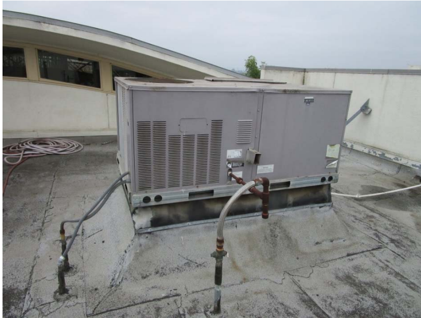
Packaged rooftop AC unit is at the end of its expected useful life.
