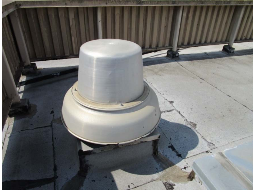
Rooftop exhaust fan is at the end of its expected useful life.
