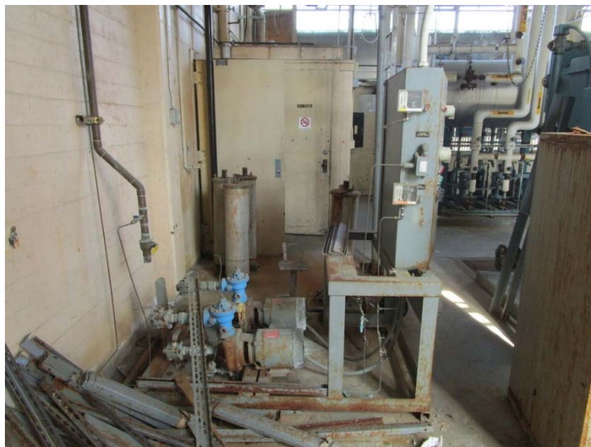
Recirculating pumps are in poor condition and will need to be replaced.
