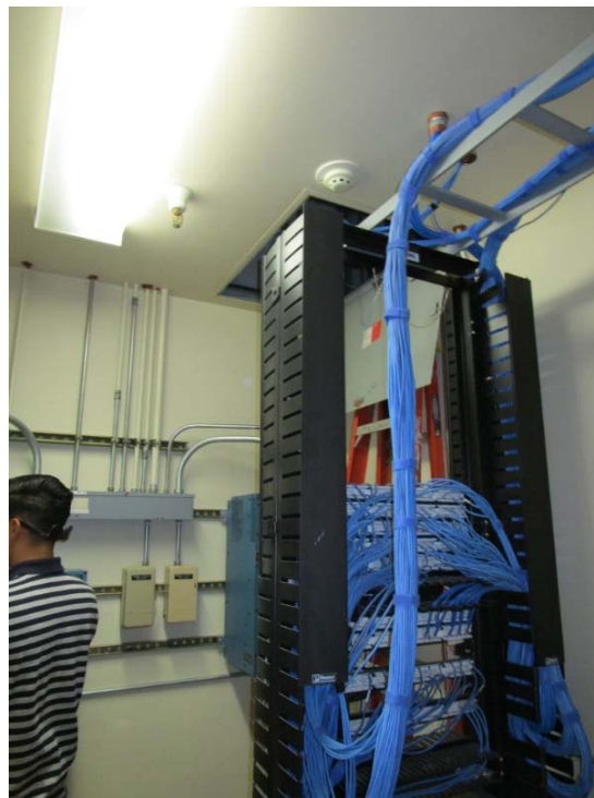
The Data Room contains data equipment and gets very warm. Recommend installing a new split ductless HVAC system in this room to maintain proper room temperature.
