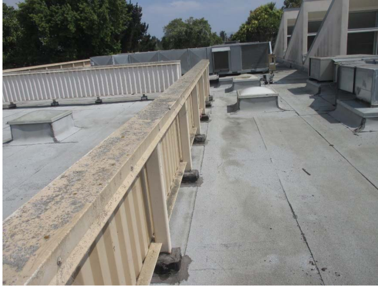
Rooftop mechanical screen is worn
