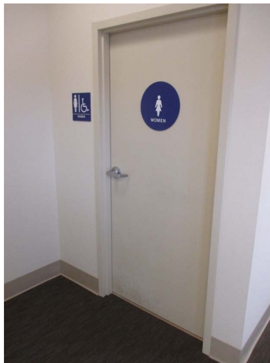
Restroom doors need paint
