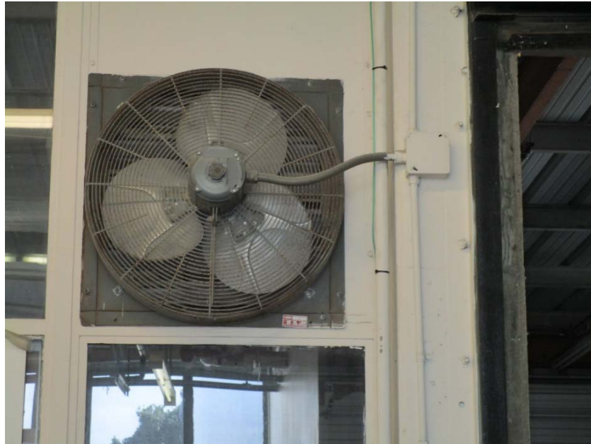
Circulating fan is at the end of its expected useful life.
