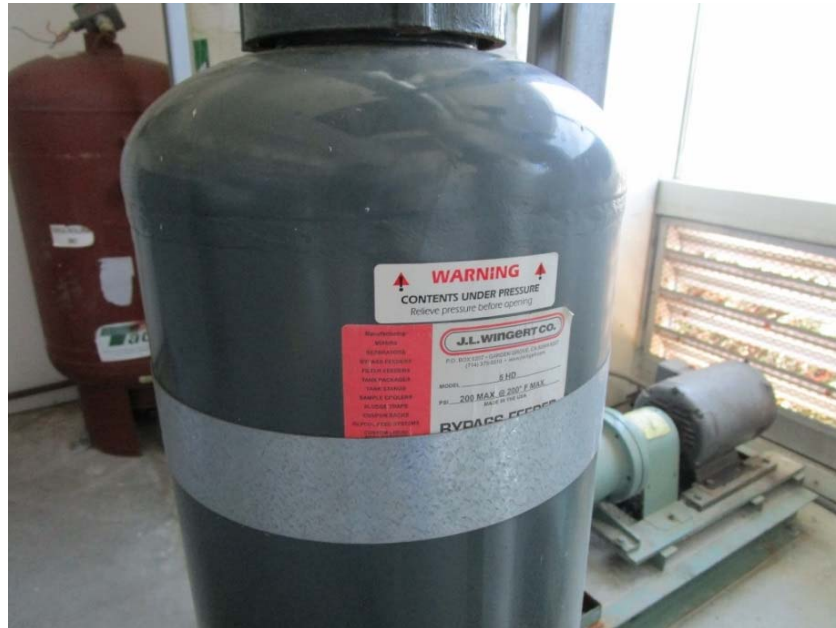
Chemical feeder is at the end of its expected useful life.
