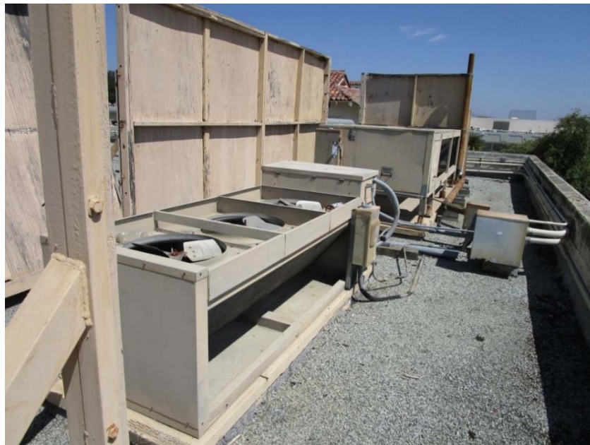
Rooftop air cooled chillers are at the end of their expected useful lives.
