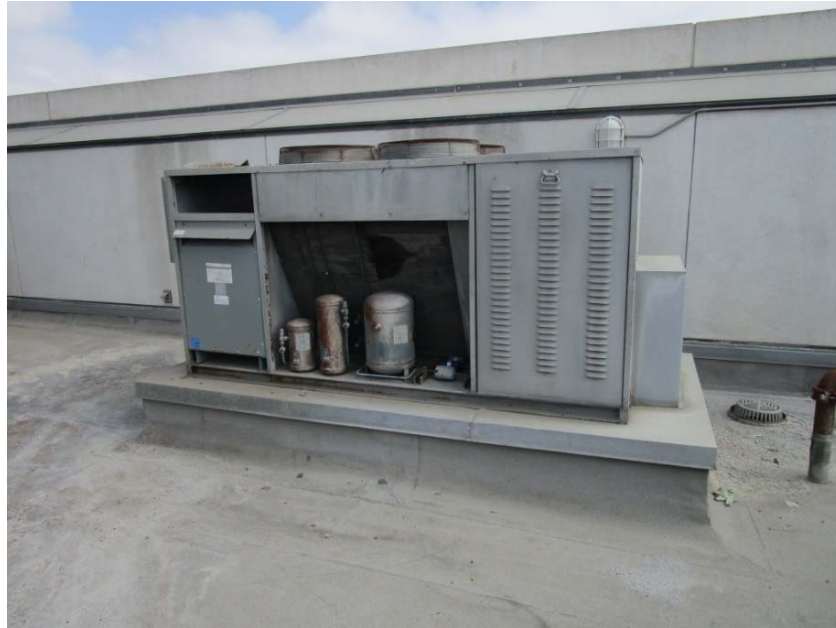
Rooftop refrigeration condensing unit and indoor evaporators for the walk-in refrigeration system are at the end of their expected useful lives.
