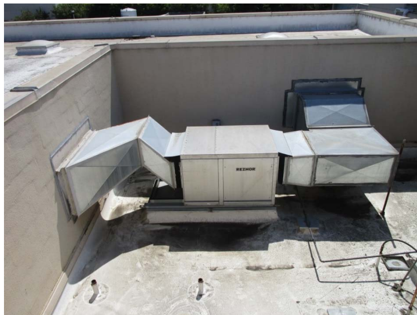
Rooftop heating and ventilation unit is at the end of its expected useful life.
