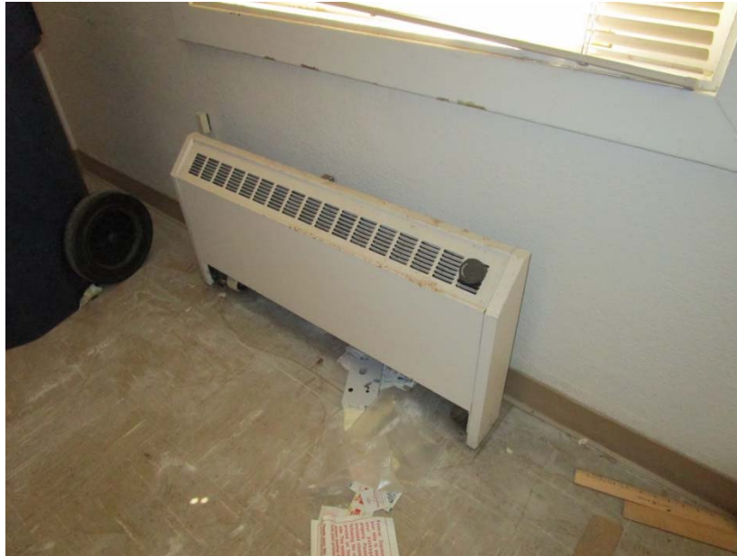
Radiant wall heater is at the end of its expected useful life.
