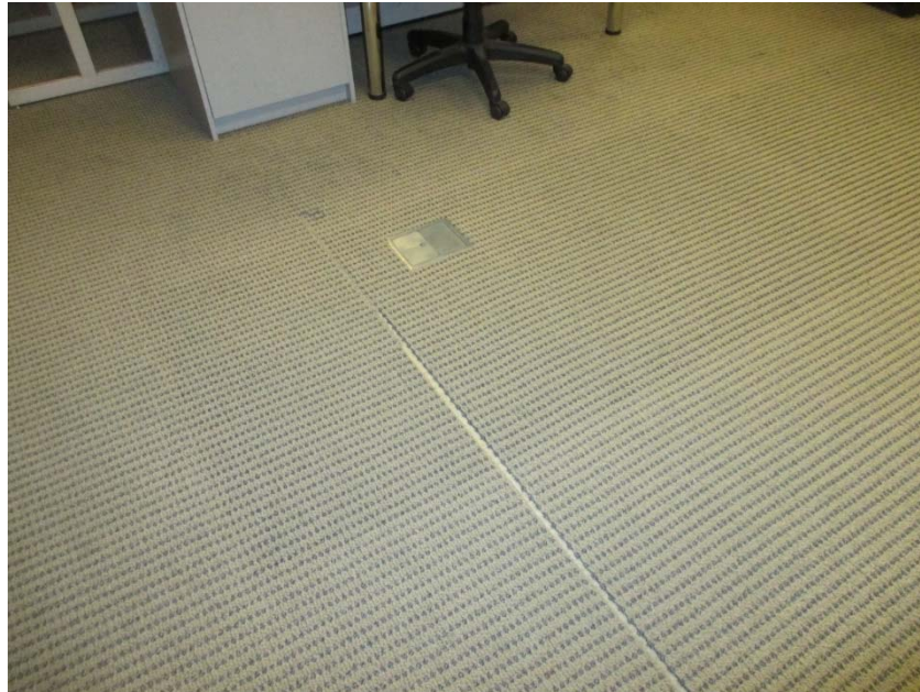
Carpet requiring replacement.
