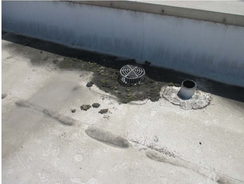
Roof drain with sediment and vegetation
