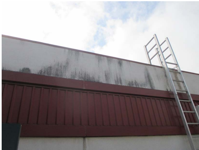
Exterior finish has staining
