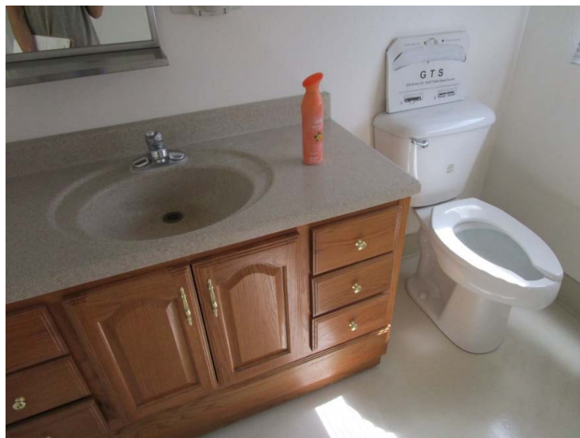
Building 820 currently no means of ventilation in the restroom. A ceiling exhaust fan will need to be installed to maintain proper ventilation.
