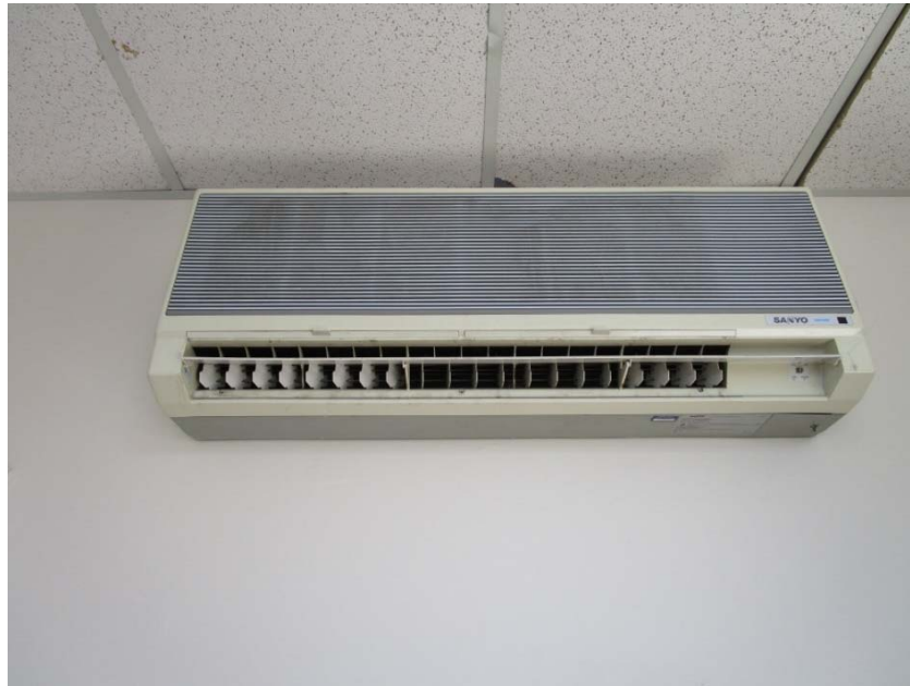
Split ductless air conditioning system is at the end of its expected useful life.
