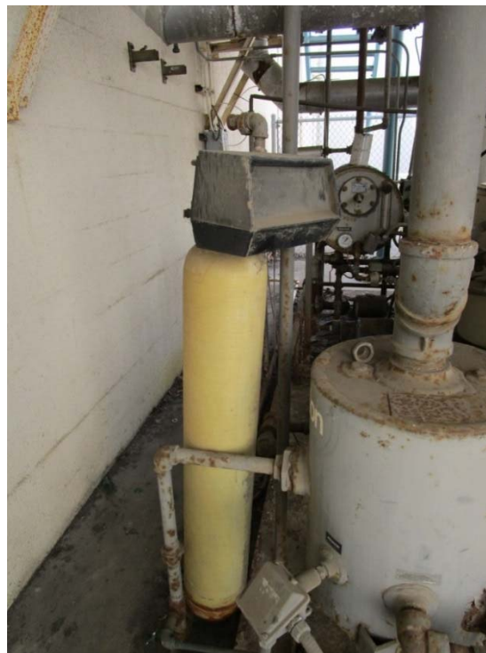
Water softener system is in poor condition and will need to be replaced.
