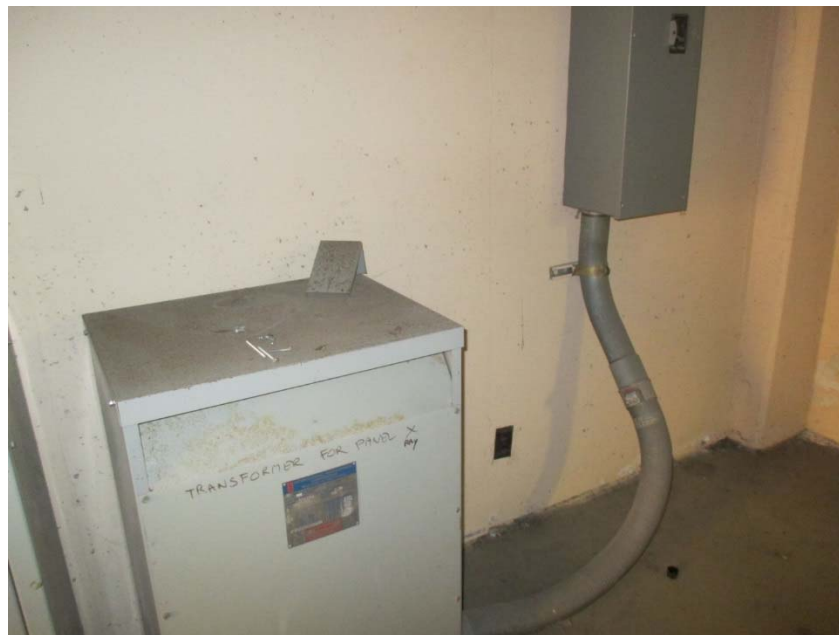
All transformers are past their expected useful lives.
