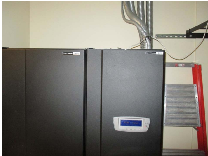
Uninterruptible Power Supply (UPS) is due for a battery replacement.
