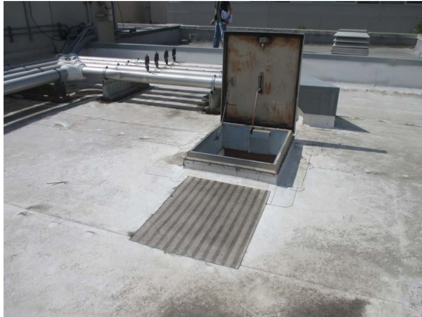
Roof hatch requiring fall protection
