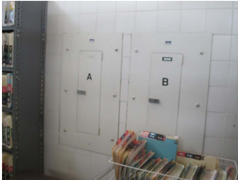
All wall recessed panels are approaching the end of their expected useful lives.
