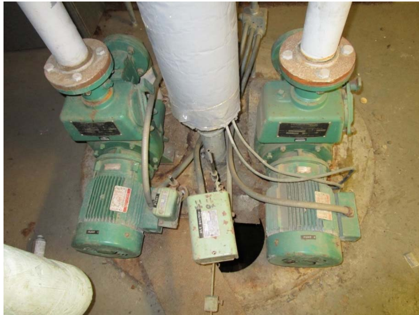
Recirculating pumps are at the end of their expected useful lives.
