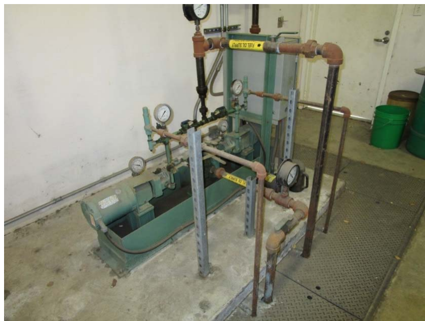
Booster pump controller system for the diesel fuel daytank is at the end of its expected useful life.
