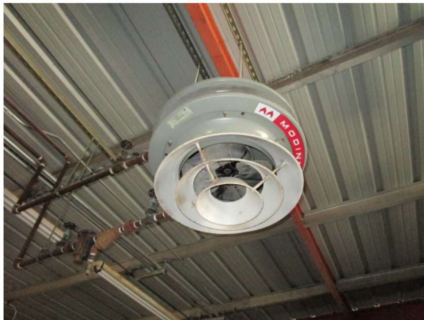
Gas unit heater is at the end of its expected useful life.
