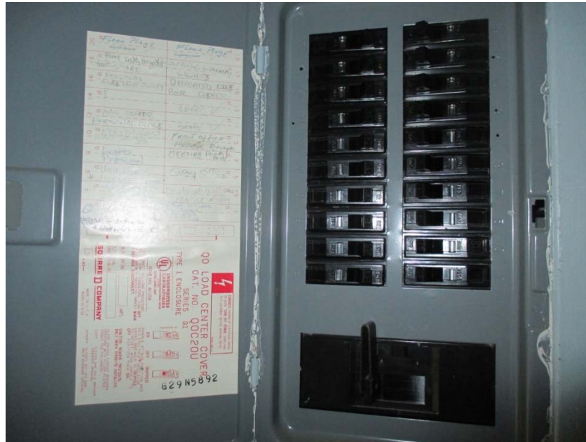
Two panels are past their rated usable lifetime and should be replaced.
