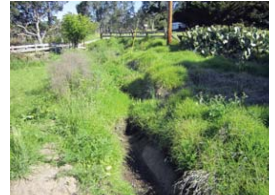
④ View of drainage channel facing Hall Road, which drains to Carneros Creek
