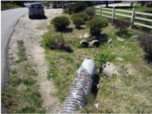
② Outlets from culverts under driveways and under Las Lomas Drive to drainage ditch
