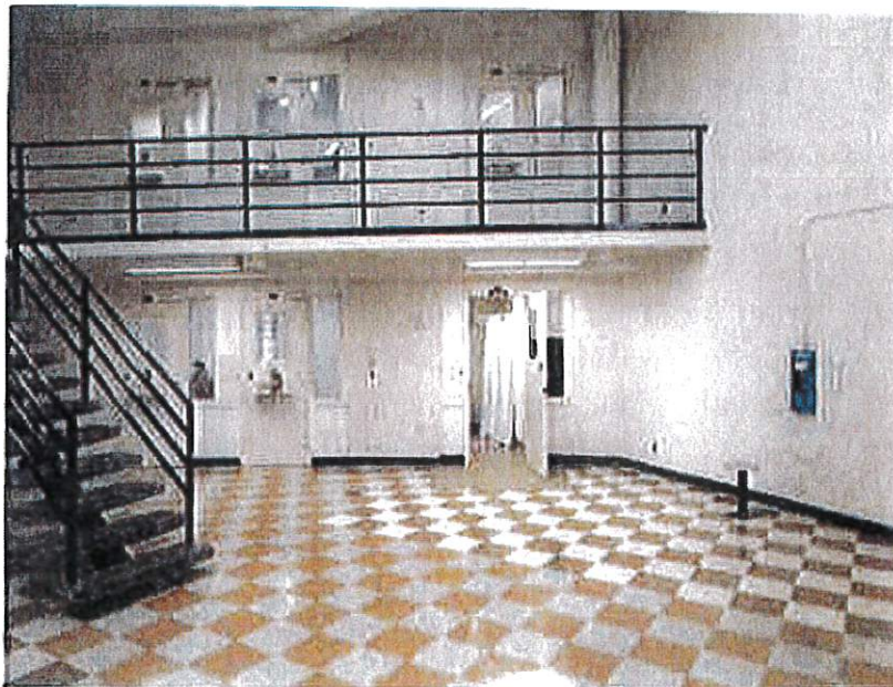
Women's Housing R and S Pod - Railing on upper level can be scaled or tied off.
