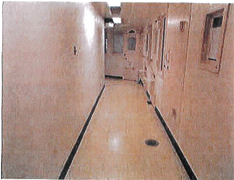
Women's Housing V Pod – Holding cells cannot be observed from a central location.
