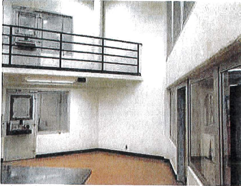
Men's Housing A and B Pod – Railing on upper level can be scaled or tied off.
