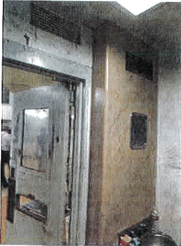
Men's Housing A and B Pod – Mechanical grills in cells have excessive openings. Return air grill is on the right in photograph.
