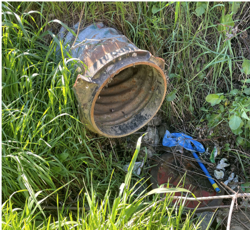
Photo 5. Area B-3 Outfall (15" CMP with broken flap gate)
