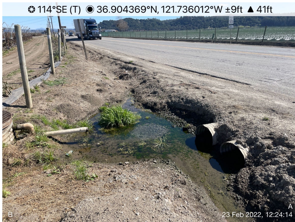
Photo 6. Inlet side of double 22"x12" CMP culvert crossing San Juan Road at Allison Street. These CMP pipes have a capacity of approximately 12 cfs prior to road overtopping.
