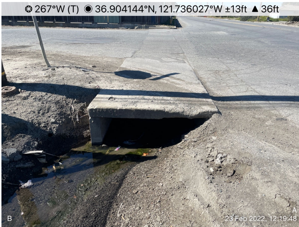
Photo 7. Inlet side of 4.5'W x 1.5'H box culvert crossing Allison Street at San Juan Road. Culvert has a capacity of approximately 22 cfs prior to road overtopping.
