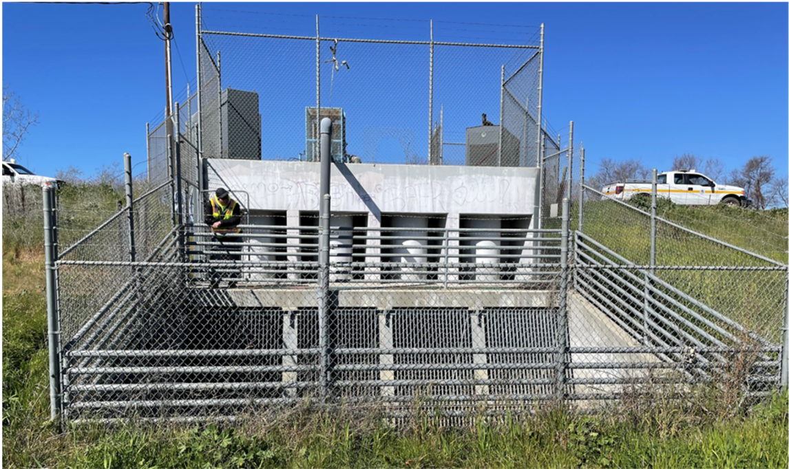
Photo 1. Susan Street Storm Drain Pump Station
