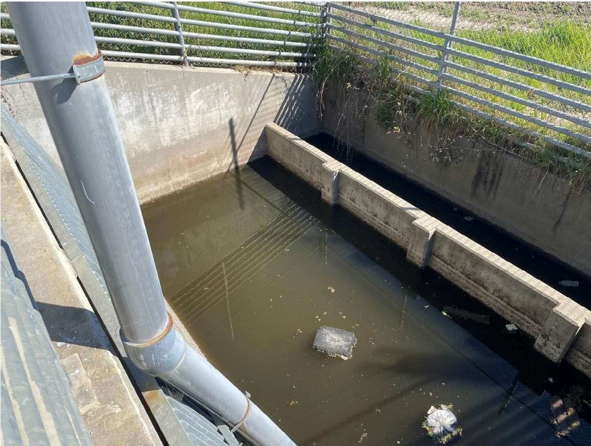
Photo 2. Pump station inlet bay with trash pump suction pipe in foreground
