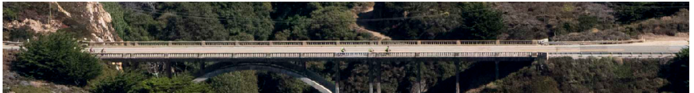
Garrapata Creek Bridge Railings and Balusters. Photo date: October 2, 2019; excerpt from CCRP Image 201900706
