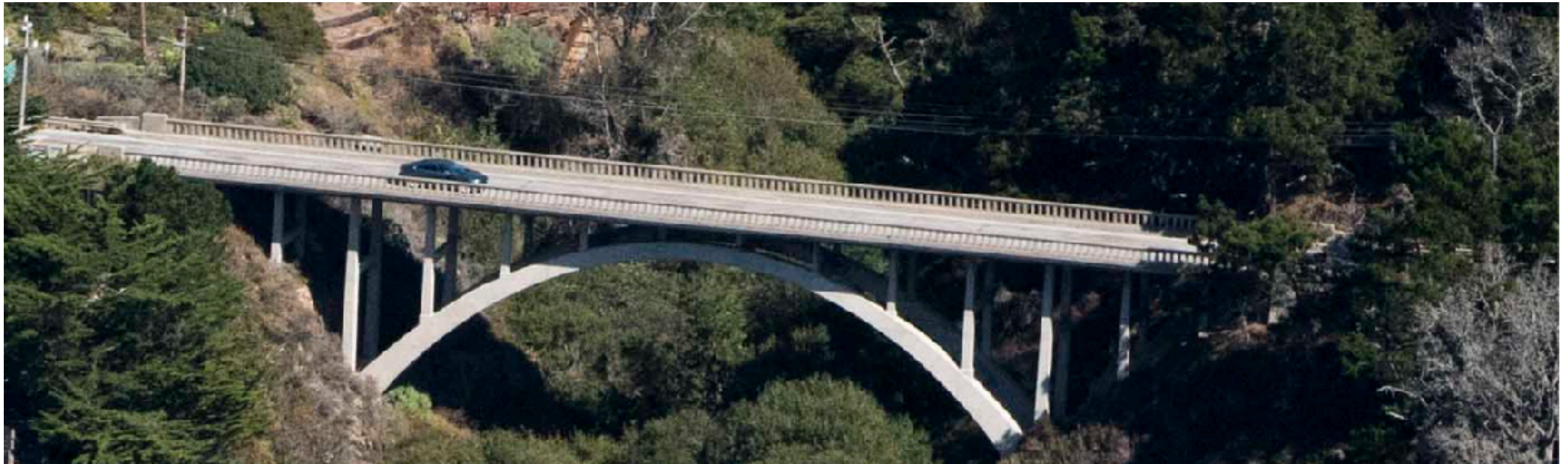
Malpaso Creek Bridge Railings and Balusters. Photo date: October 2, 2019; excerpt from CCRP Image 201900658
