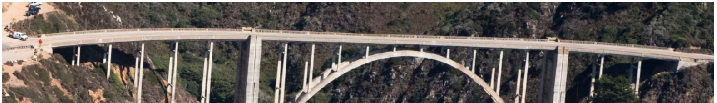
Bixby Creek Bridge Railings and Balusters. Photo date: October 2, 2019; excerpt from CCRP Image 201900745.
