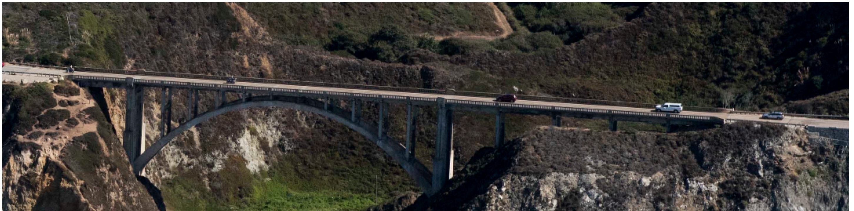
Rocky Creek Bridge Railings and Balusters. Photo date: October 2, 2019; excerpt from CCRP Image 201900737.
