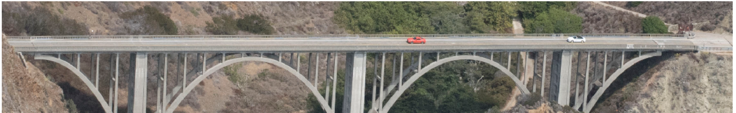
Big Creek Bridge Railings and Balusters. Photo date: September 11, 2015; excerpt from CCRP Image 201501549.
