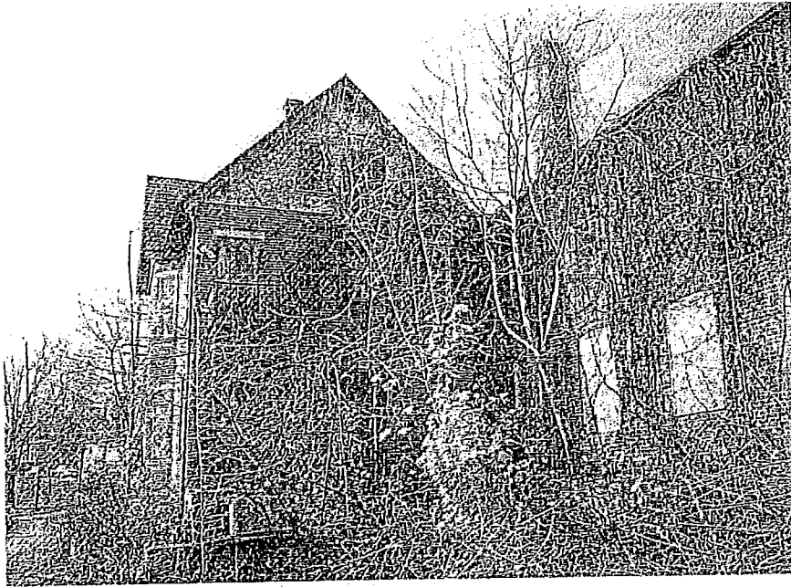
Figure 2. Improper treatment: Boarding up without adequate ventilation, lack of maintenance, and neglect of this property have accelerated deterioration. Photo; NPS file.
