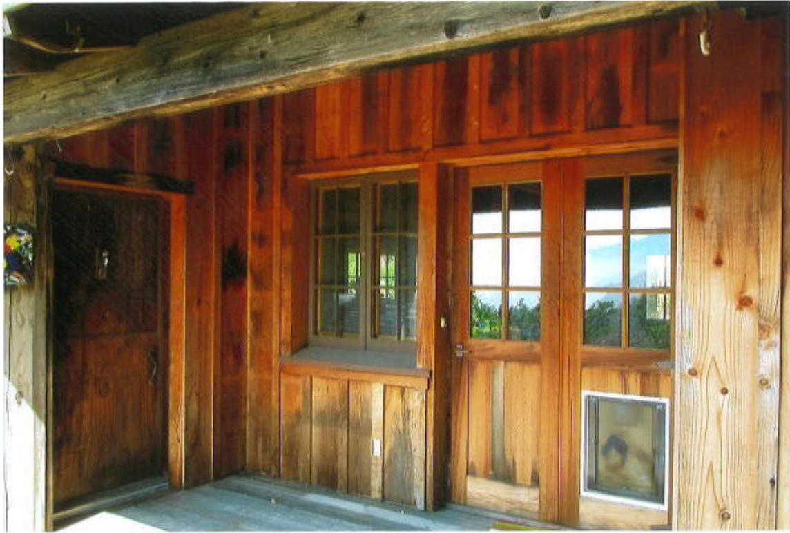
Photo #5. Looking at recessed entry on South elevation proposed for in fill to beam under existing roof overhang. Doors & windows proposed for repurposing on project, Kent Seavey, October 2020.
