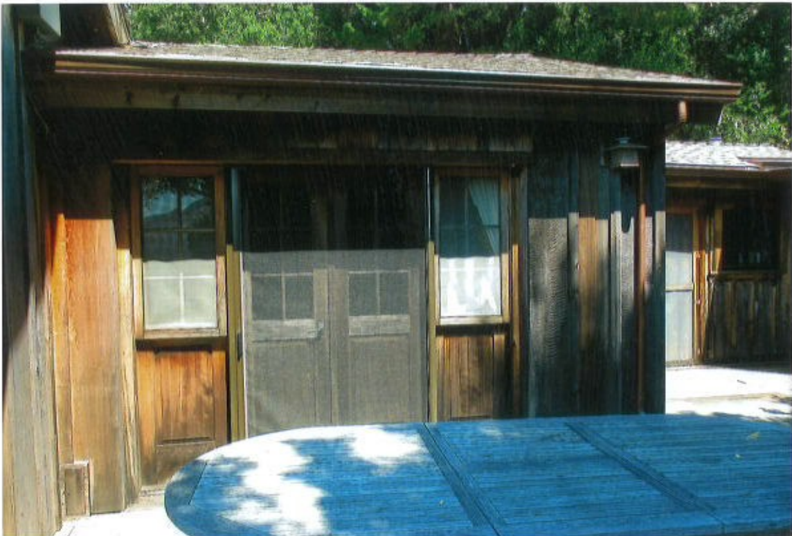
Photo #6. Looking North at bedroom double-doors proposed for single light reglazing & window/door far right for minor reconfiguration, Kent Seavey, October, 2020.
