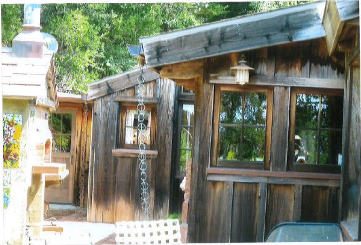
Photo #3. Looking East at the North side additions, entry door to laundry room at left, bathroom window, center & wide fascia boards, Kent Seavey, October, 2020.
