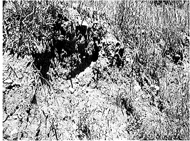
Photo 2. Burrow located in the bank of Pancho Rico Creek on the northeast side of the upstream end of Bridge 412.
