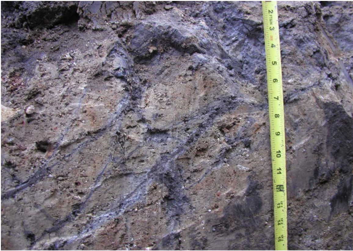
Photograph No. 14: Clay shear surfaces exposed in TP-5, Lot 3.
