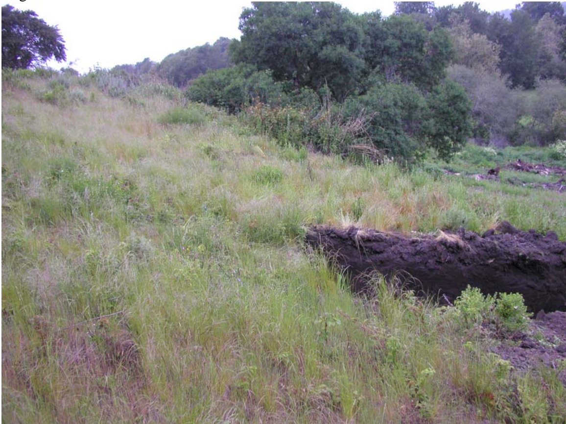
Photograph No. 13: Surface condition near headscarp of small slide Lot 3.
