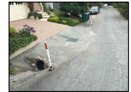
APPROX. LOCATION OF STORM DRAIN COLLECTING STORM WATER RUNOFF FROM LINCOLN ST, 1ST AVE AND BEYOND - UPSLOPE FROM THE KOSTIGEN RESIDENCE
