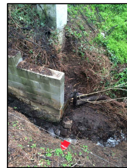
EXISTING MONTEREY COUNTY MAINTAINED STORM WATER DRAINAGE CHANNEL CAUSING SEVERE EROSION AND DAMAGE TO BUILDING FOUNDATIONS.
