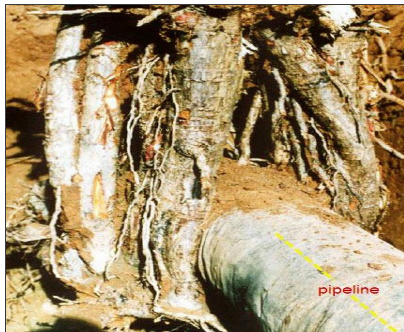
Example of the impact tree roots can have on a gas pipeline.
