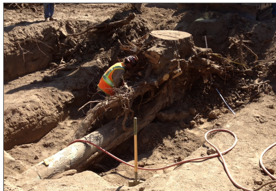
Example of the impact tree roots can have on a gas pipeline.
