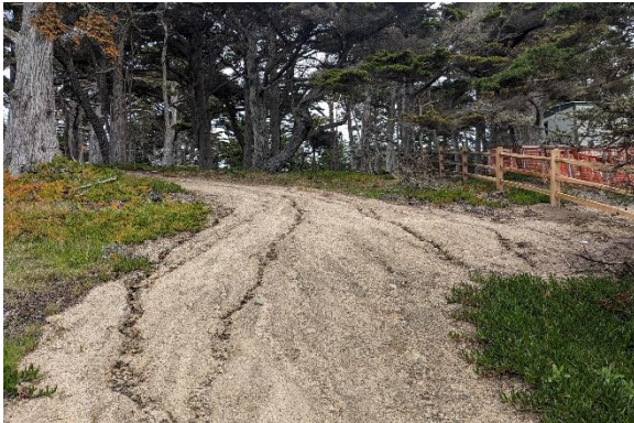
Photo 3. Looking northeast from the western end of the roadcut. Bare ground and erosion gullies present on disturbed slope.
