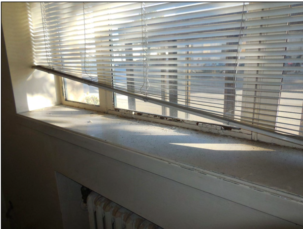
East Wing window visibly in moderate-poor condition
