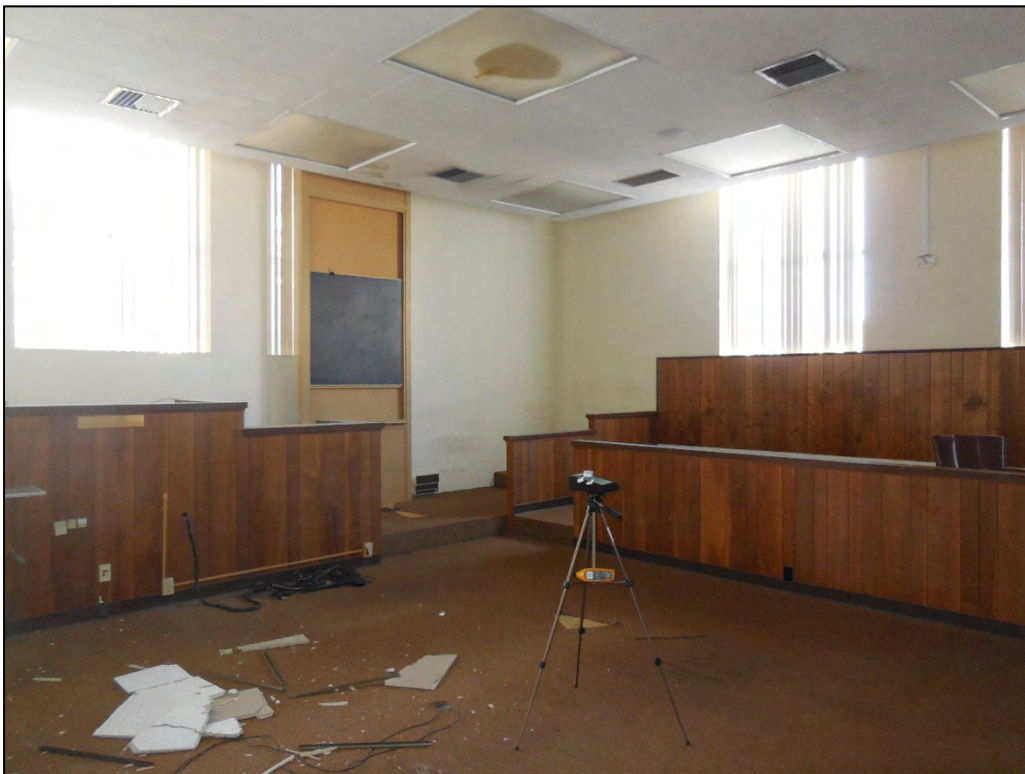
Air sampling in the East Wing courtroom 2-4; Water damage visible on ceiling in background
