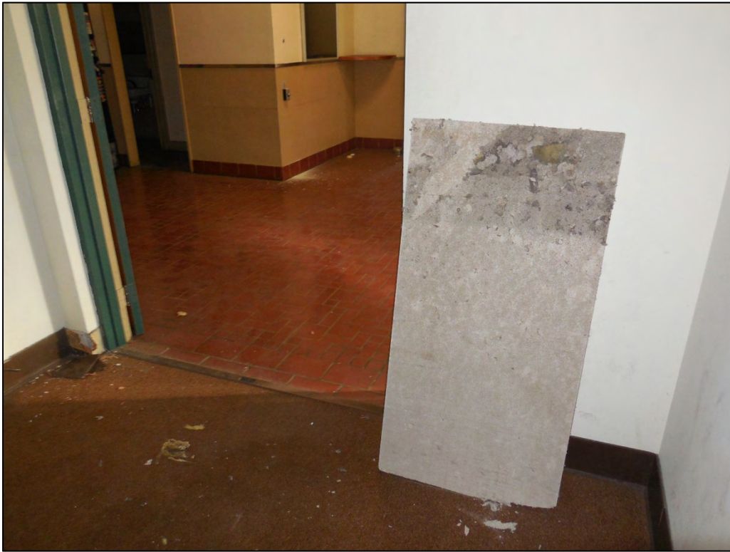
Suspect mold growth visible on lay-in ACP in East Wing
