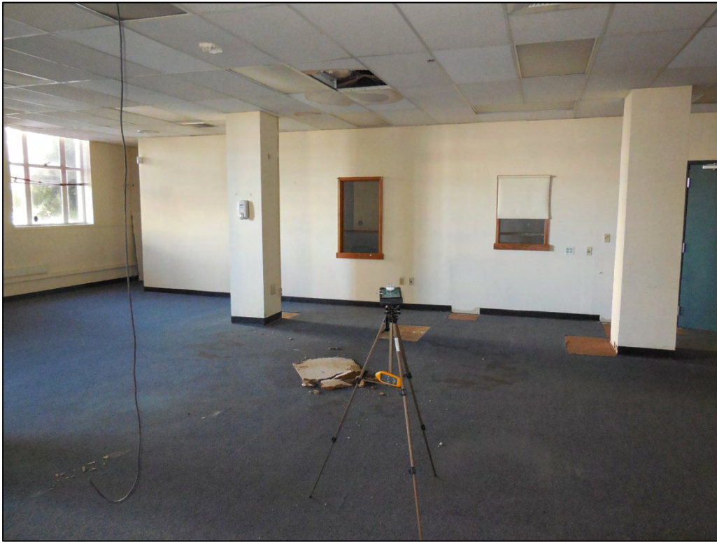
Air sampling in the East Wing cubicle area 1-22; Site of active leak visible in background
