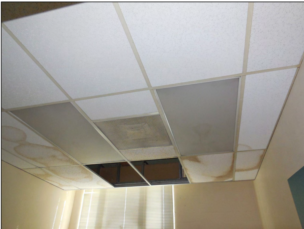
Visible water damage on lay-in ACP in West Wing
