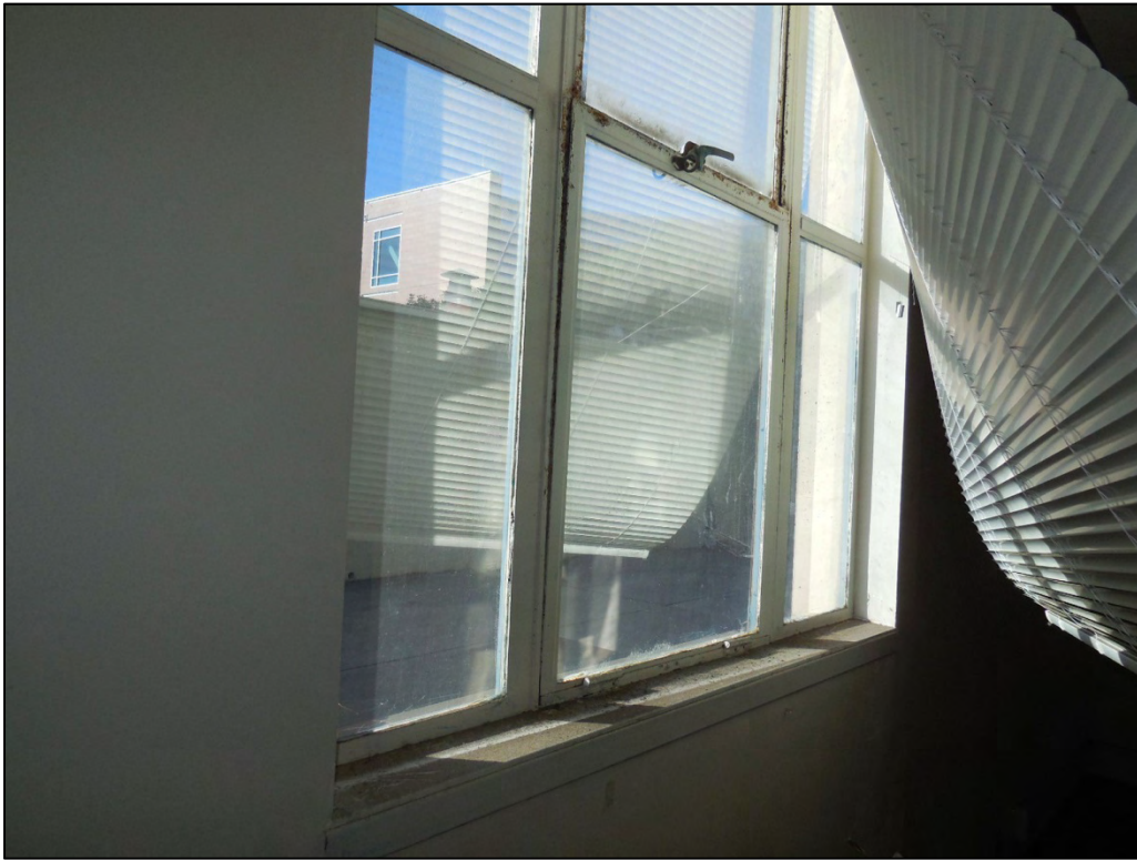
West Wing window visibly in moderate-poor condition
