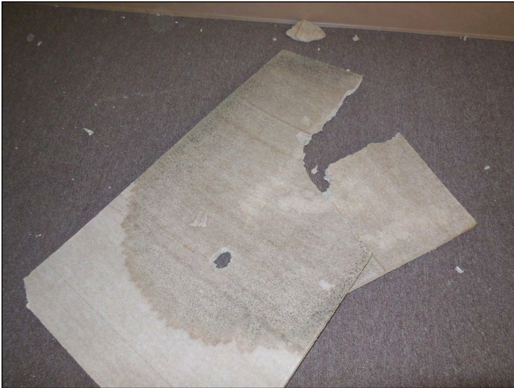
Visible suspect mold growth on lay-in ACP in West Wing
