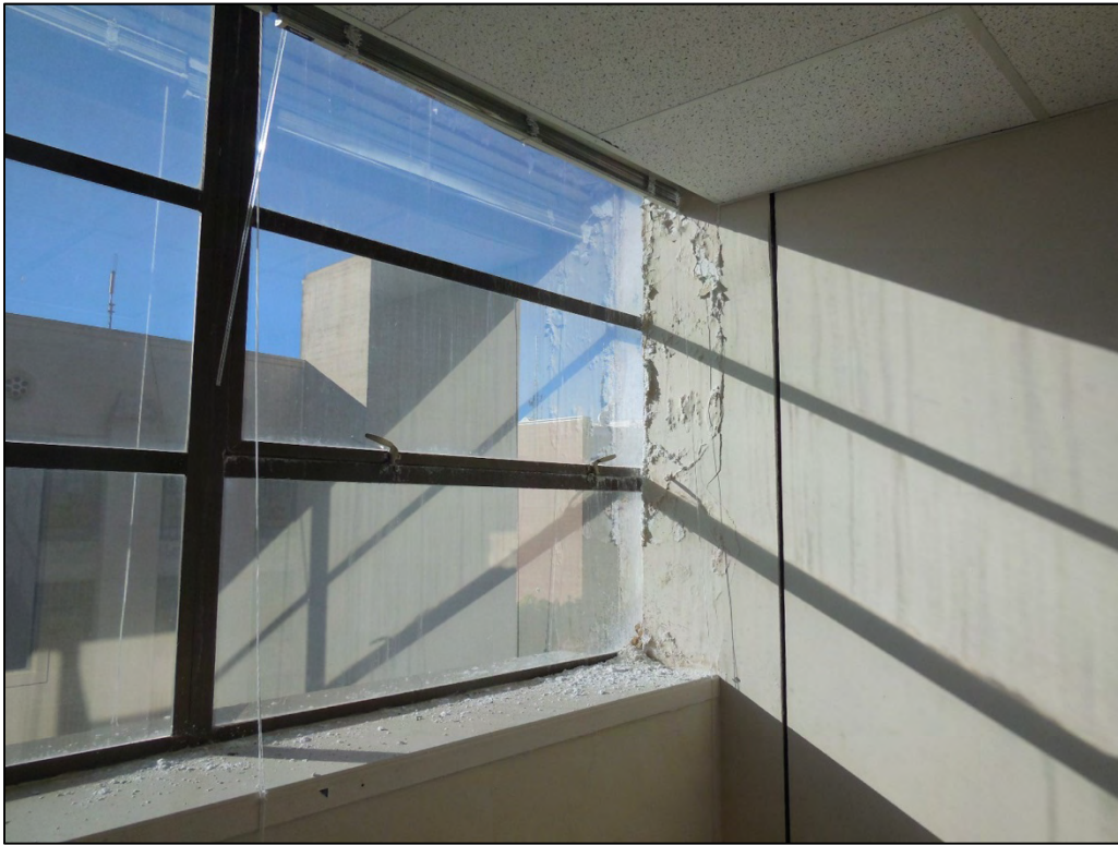
Heavy efflorescence visible on exterior wall in West Wing
