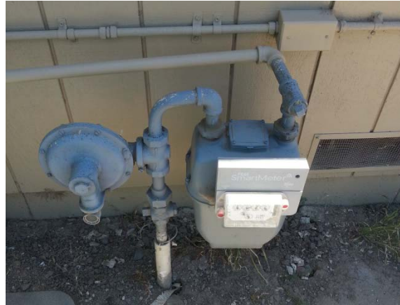
Gas connection and meter
