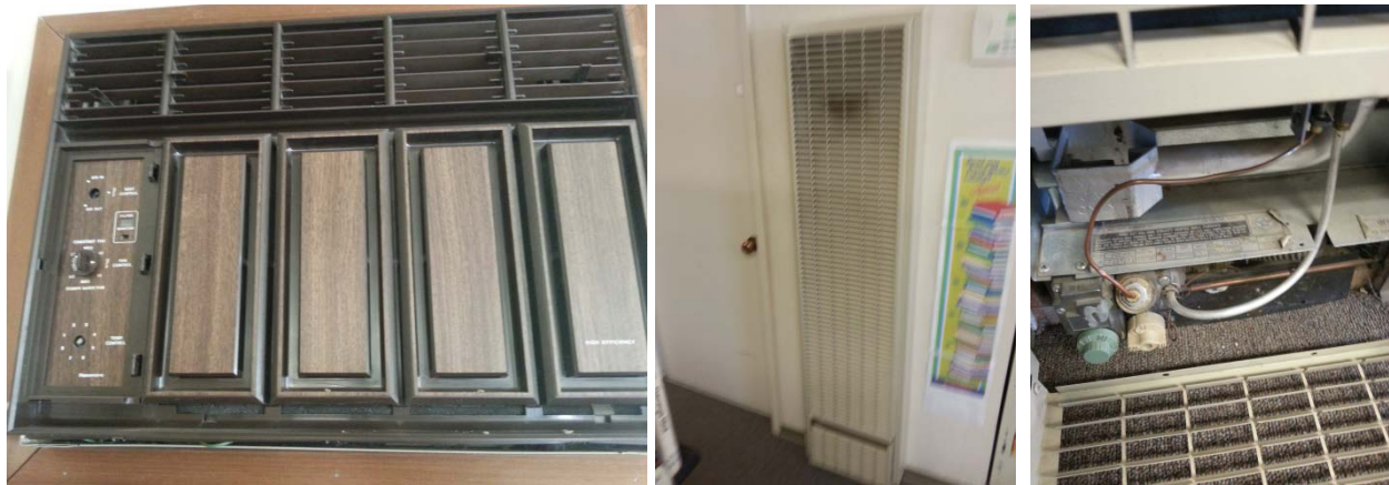
(L to R) Room air conditioner, Wall Heater unit, Wall Heater Unit connection and control panel
