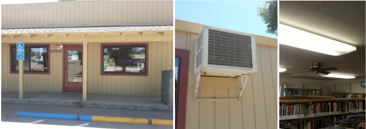
(L to R) Ventilation items: Operable windows, Room AC with fresh air intake, Ceiling fan
