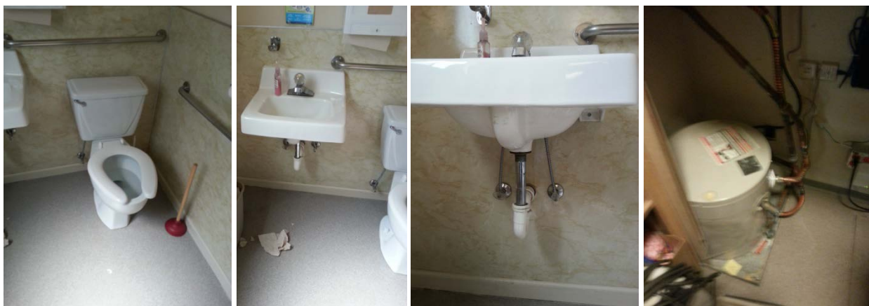
(L to R) General Plumbing items, Water Closet, Hand Wash Sink, Hand Wash Sink connections, Hot Water Unit.
