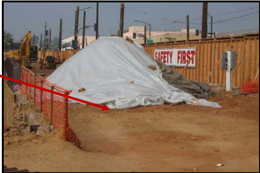
Stockpile covered with plastic and secured with large rocks. Where more than one sheet of covering is required, overlap sheets and secure at seam.
