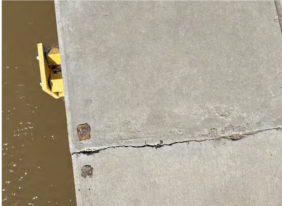
Figure 2: Missing Crack Meter
