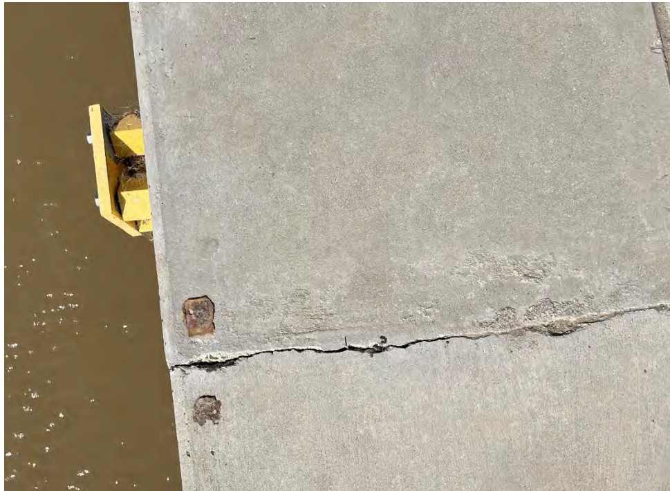
Figure 2: Missing Crack Meter
