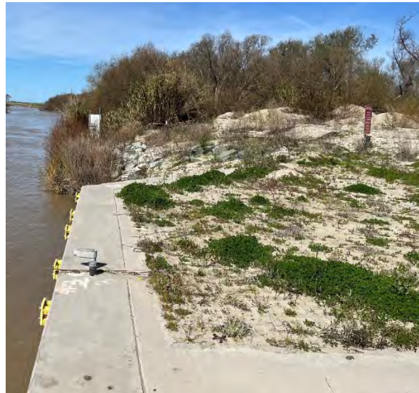
Area 2 RB wing walls: remove silt and replace riprap. Area 14,000 sq ft, volume est. 500 yards (ave depth 1 foot)
