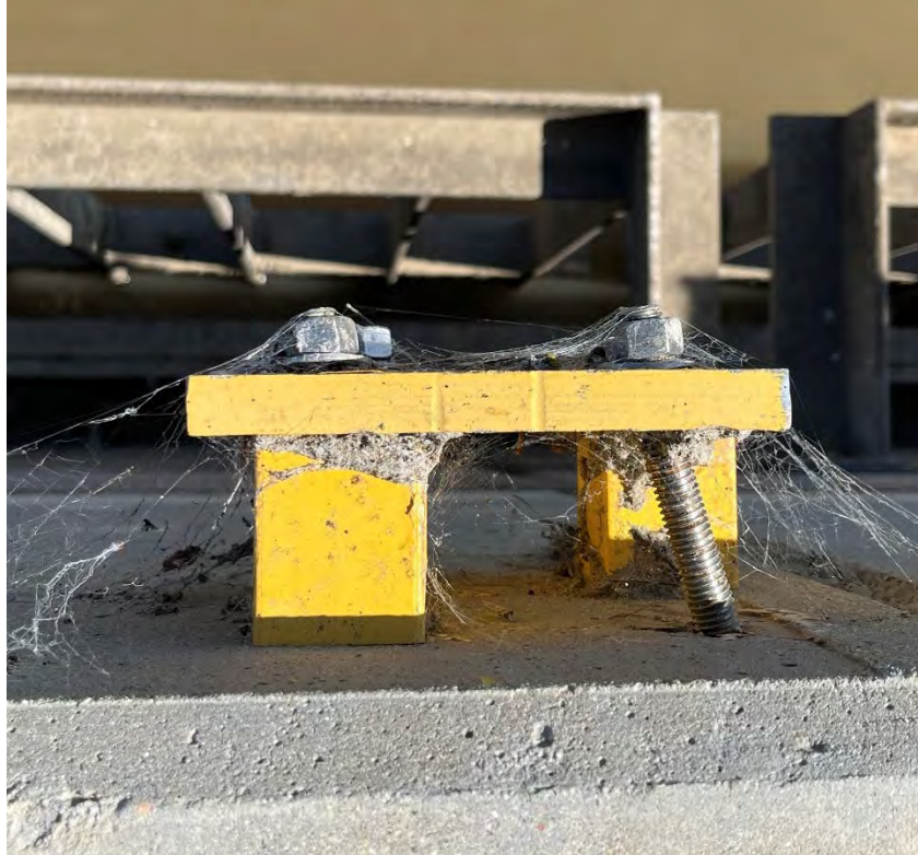
Figure 4: Damaged Rail Support
