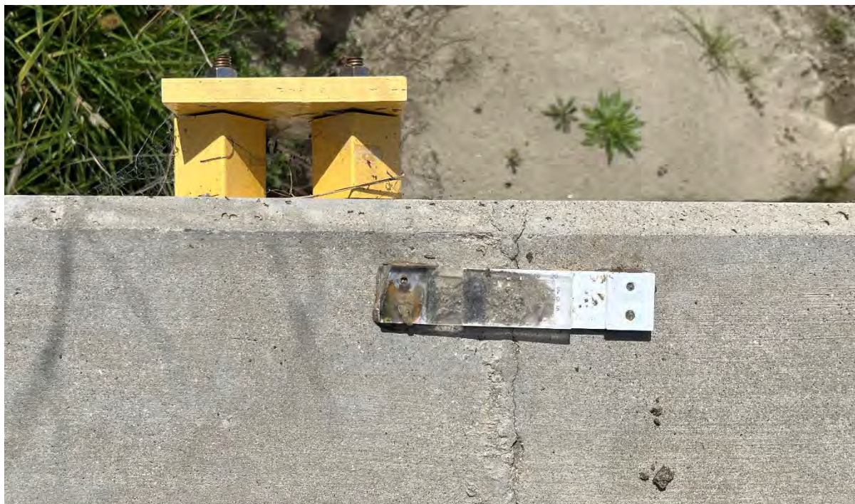
Figure 3: Crack Meter needs cleaning.
