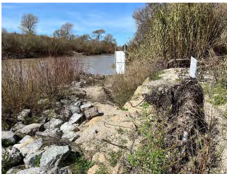
Figure 6: Downstream signage, vegetation removal needed. Repair & remove debris from foreground sign
