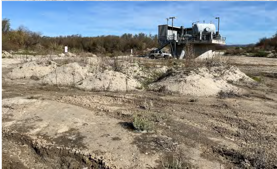
Area 1 LB Silt Removal: Further sediment removal is required to return site to original condition. Estimated area: 15,500 sq feet with an estimated silt volume of 860 yards
