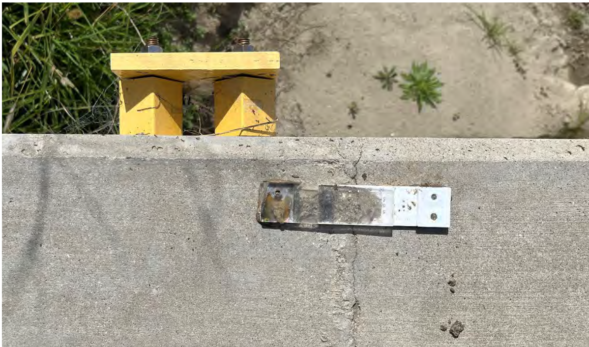
Figure 3: Crack Meter needs cleaning.
