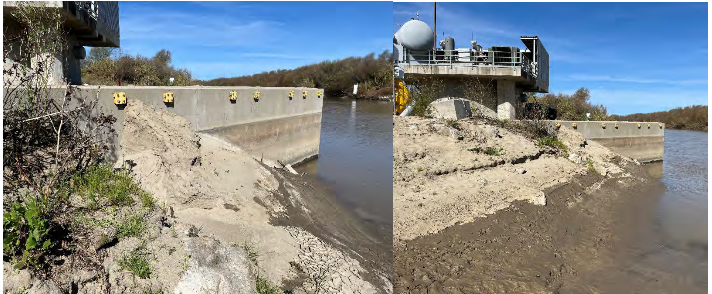
Area 3 Upstream boat ramp: Remove Sediment and debris, restore boat ramp to original condition. Area: 1300sq ft, sediment varies in depth estimated at 80 yards (average 1.5 feet fill)
