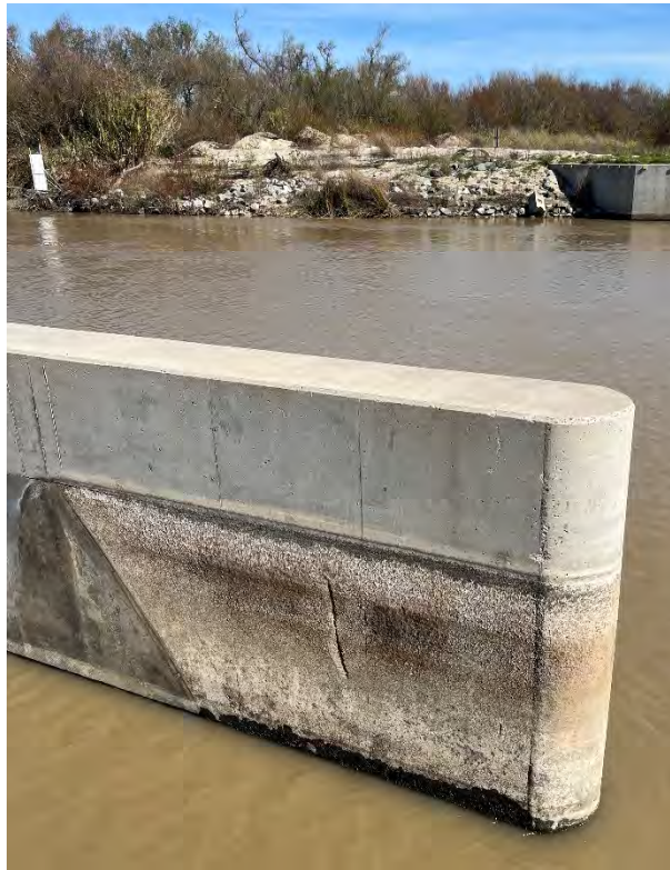
Figure 1: Gash in abutment
