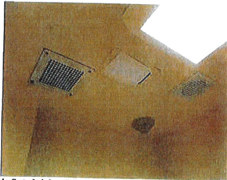
Intake Center Isolation - Cell ceilings have fixtures that have means of attachment.
