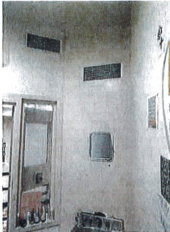
Women's Housing R and S Pod – Upper level cell mechanical grills in cells have excessive openings.
