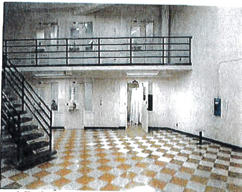
Women's Housing R and S Pod - Railing on upper level can be scaled or tied off.
