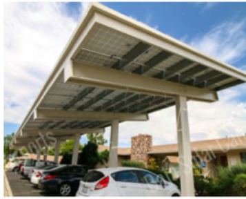
Carport with solar array on roof:
