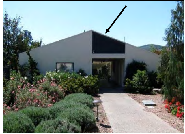
Figure 26. Rear (north) elevation of the West Parlor. Connection of two shed roofs shown with an arrow.
