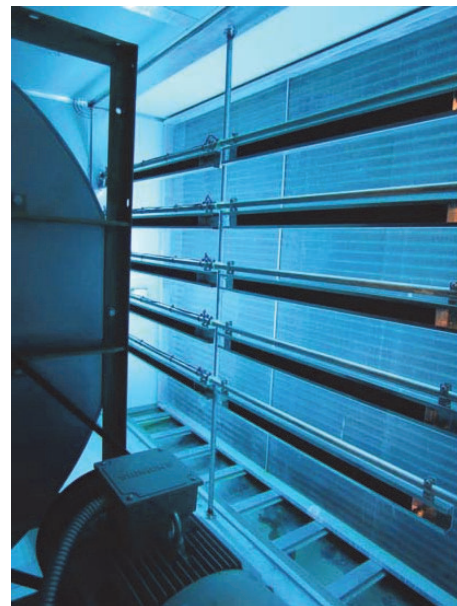
DISINFECTING WITH UVC: The APCO disinfection-odor control installed in the AHU disinfects and reduces odors with proprietary UVC and carbon ceramic lifetime tiles. Courtesy Fresh-Aire UV
