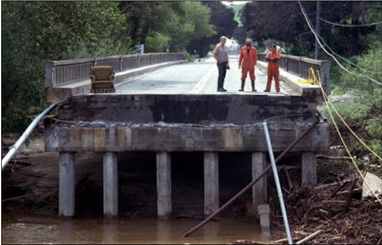
Figure 4: State Route 1 bridge over the Carmel River collapsed during March 1995 flood event.
