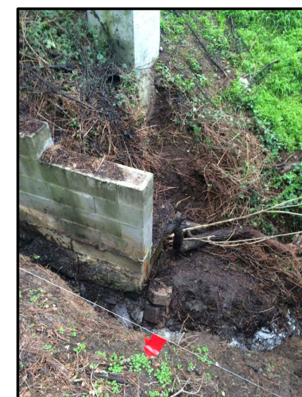
EXISTING MONTEREY COUNTY MAINTAINED STORM WATER DRAINAGE CHANNEL CAUSING SEVERE EROSION AND DAMAGE TO BUILDING FOUNDATIONS.
