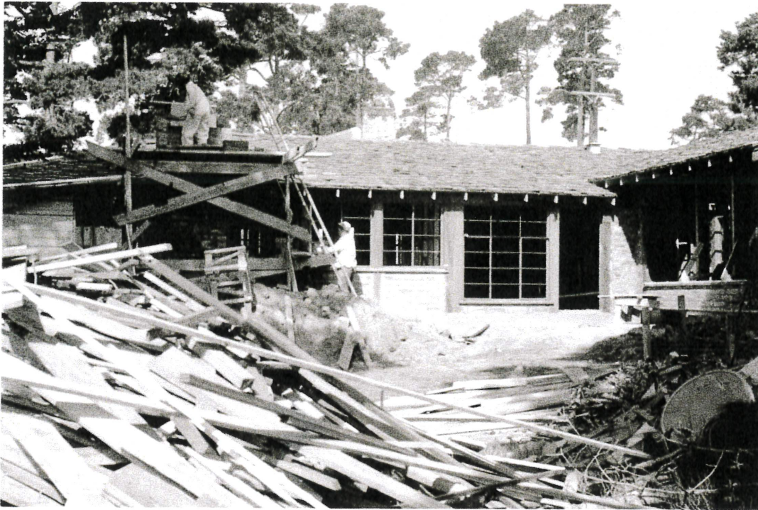
Photo #3. Looking North at the South side-elevation, note original door at right, chimney at left being built, Donald Teague photo, 1951.
