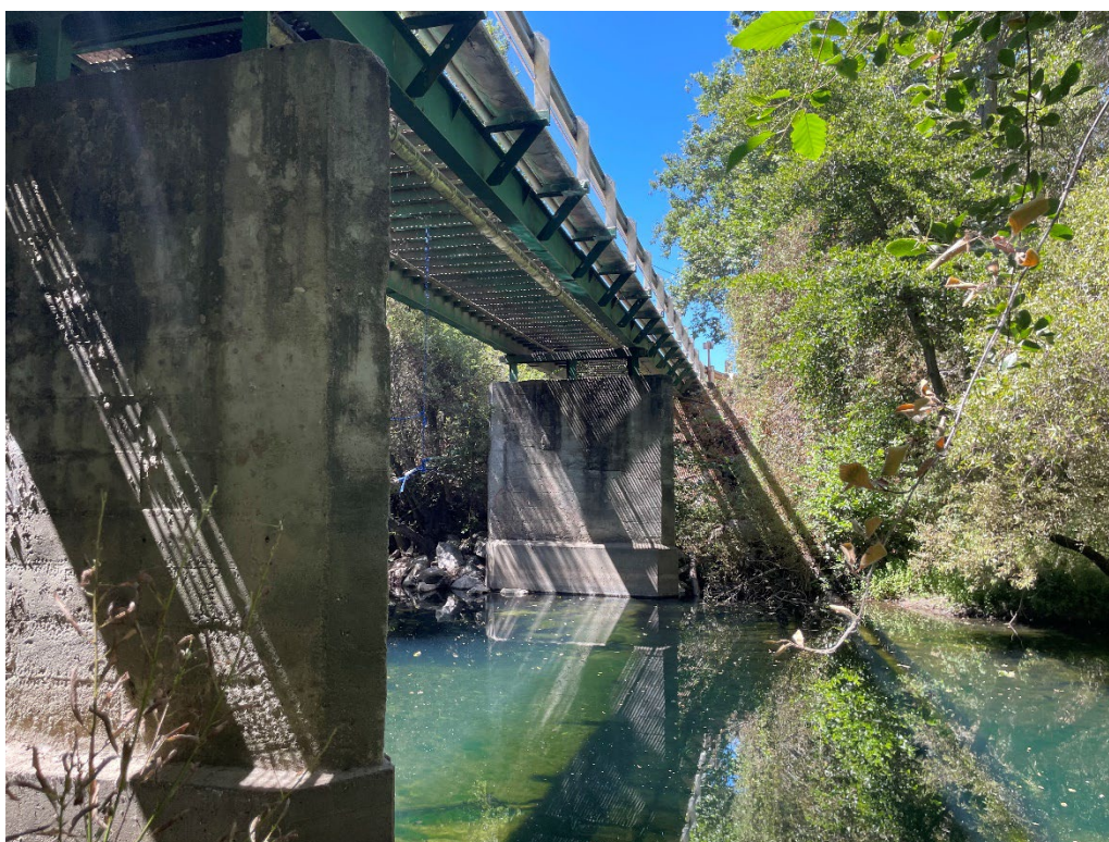
Photo 6: Looking east. Note skirt around bottom of pier from previous scour mitigation project.
