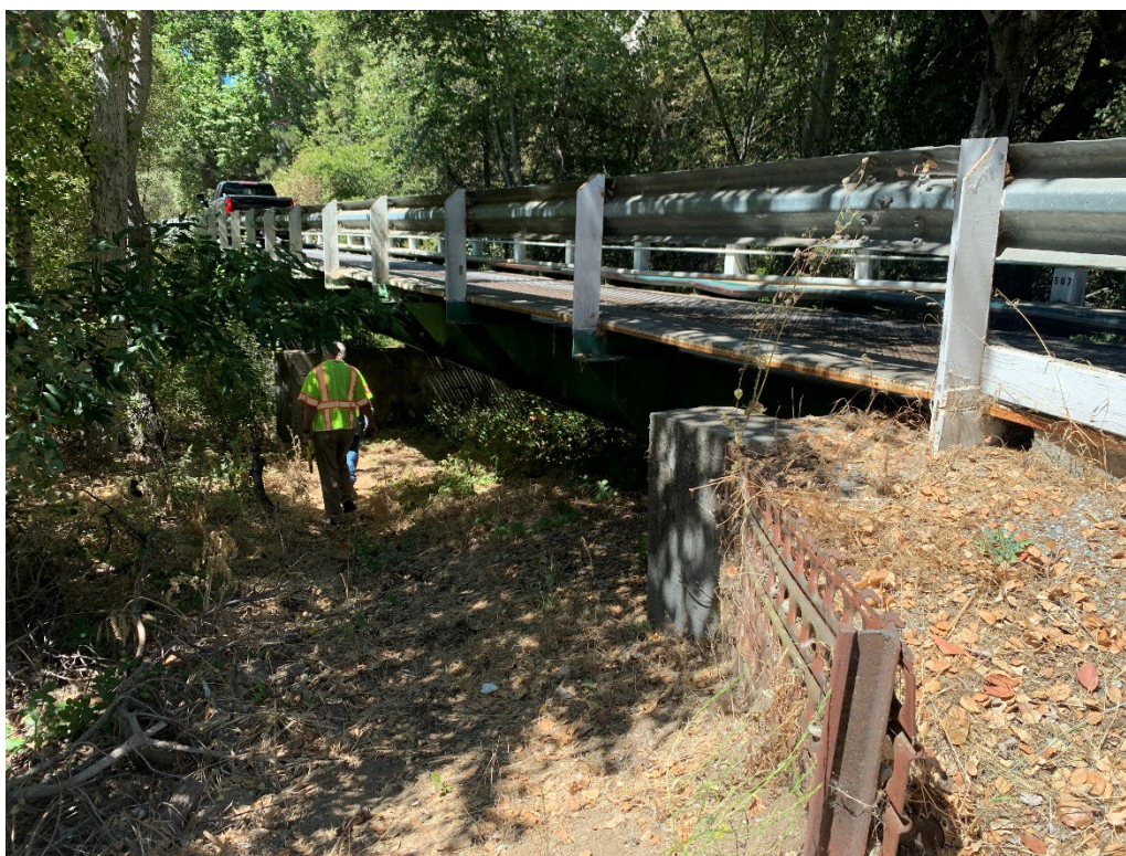
Photo 5: Low clearance under east abutment
