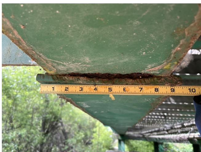
Photo 3 Typical pack rust at the end of cover plate
