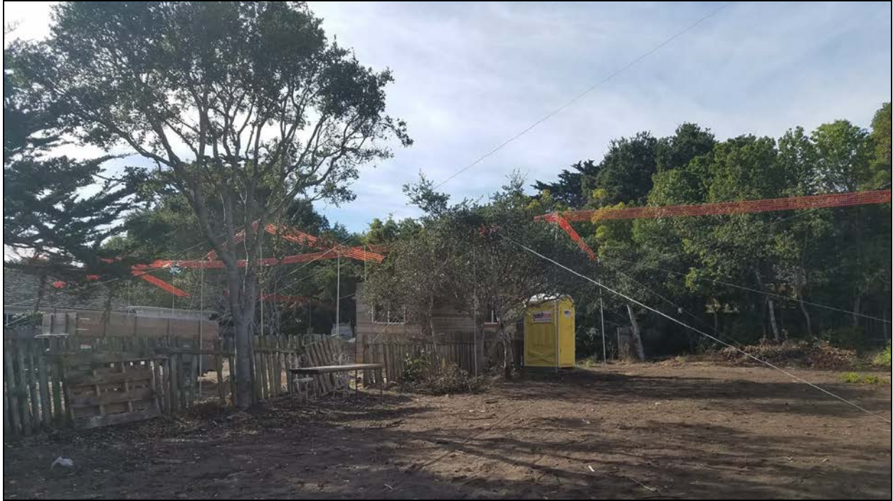
Figure 13a – Site Visit Photos: Staking and Flagging (west) at 26338 Valley View Avenue
