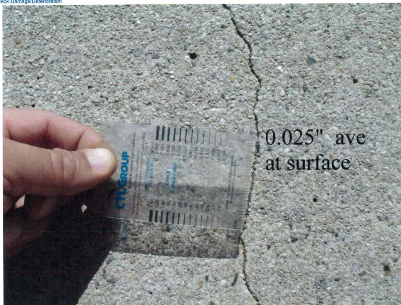
Photo #2 Typical deck crack size.
