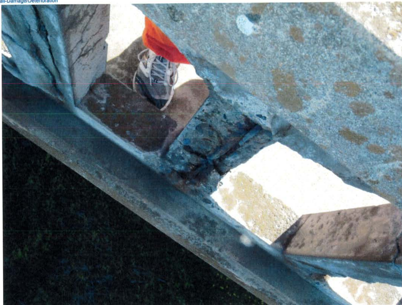
Photo #6 Gross deterioration of bridge railing.
