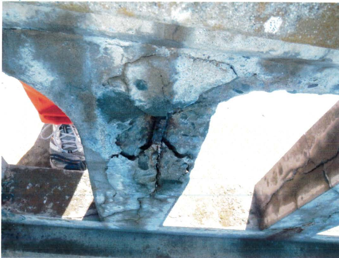
Photo #7 Gross deterioration of bridge railing.
