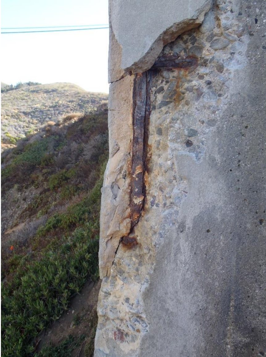
Figure 1-5 Photo of Garrapata Creek Bridge Rail Deterioration
