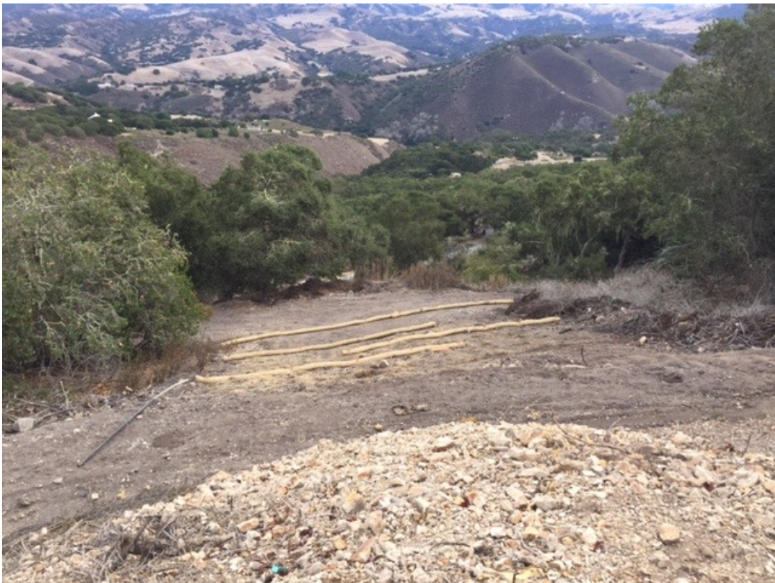
Figure 14. Straw wattles have recently been installed in lower section of slope. Additional erosion and sedimentation control and slope stabilization BMP's provided in this report should be implemented.
