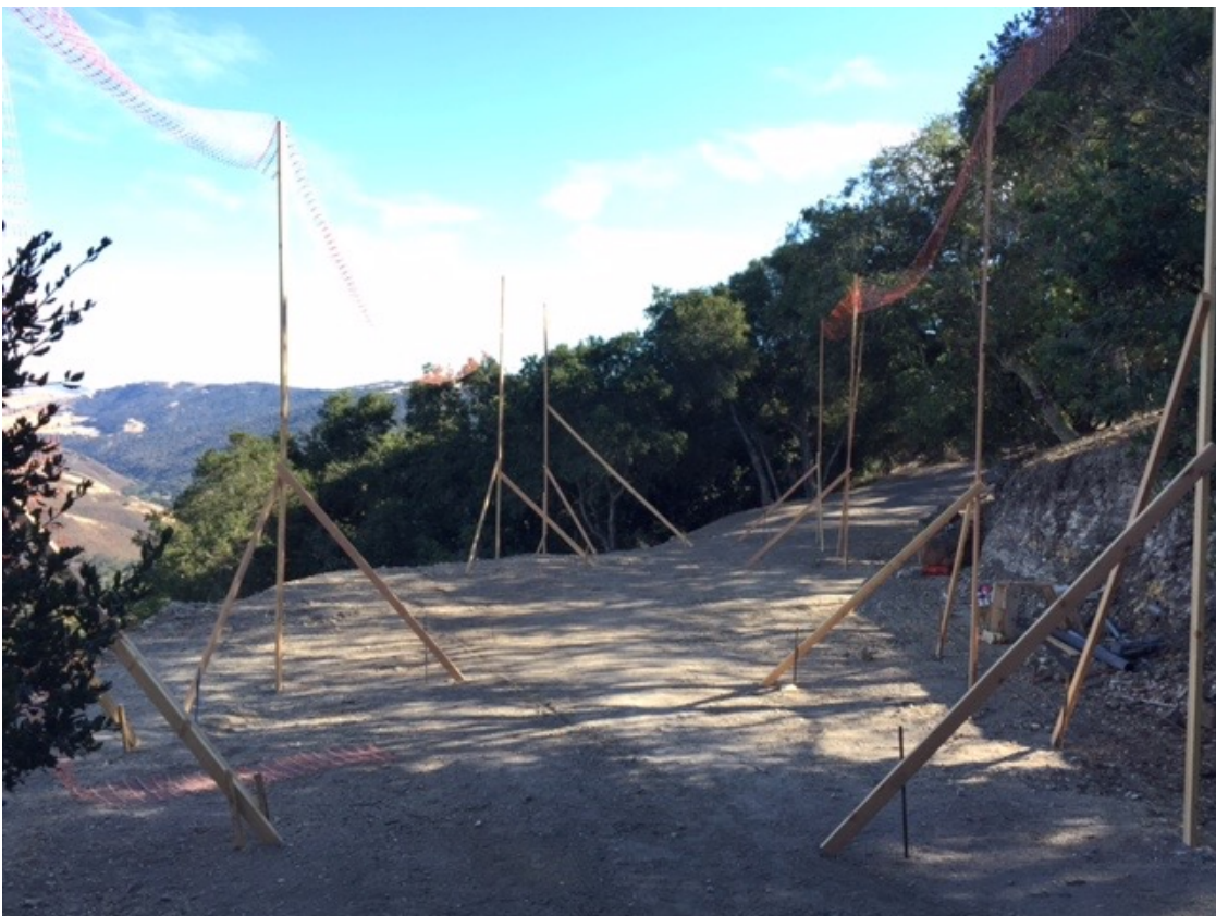
Figure 4. Building pad/terrace for proposed homesite. Retain, but apply woodchip or rice straw mulch to exposed flatter surfaces.
