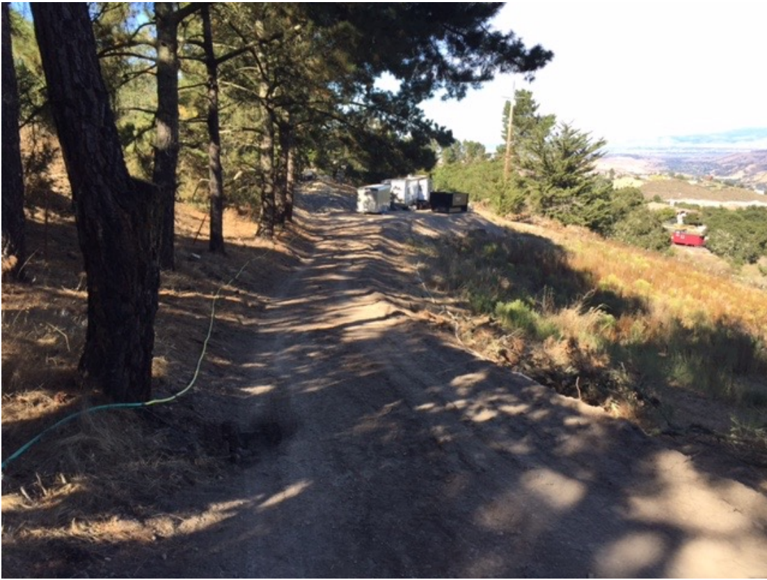
Figure 3. Graded road along upper west part of property provides access to a few trailers. It should be noted that a road existed here prior to the most recent non-permitted grading. Retain and winterize road and install silt fence along downslope perimeter of road and graded pad where trailers are located.
