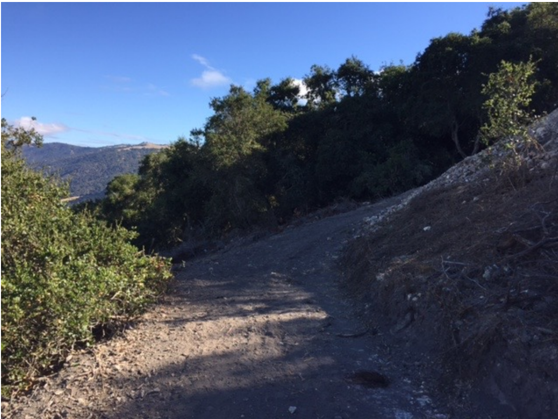
Figure 10. Shape and outslope narrow road/path into surrounding slope prior to applying and installing soil stabilization measures. Retain small oak sapling visible near right edge of photo.
