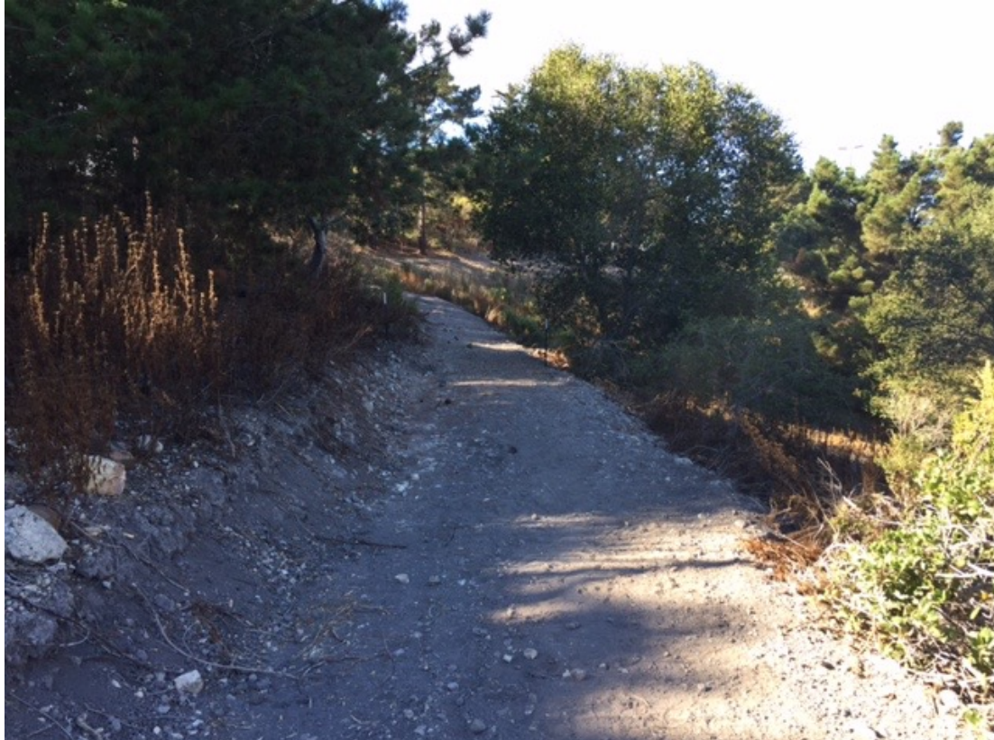
Figure 8. Outslope narrow road/path and install earthen or sand bag water bars every 50 feet to divert concentrated runoff off of exposed soil surfaces. Also apply native seed mix and rice straw or woodchip mulch to protect and stabilize exposed soil surfaces.
