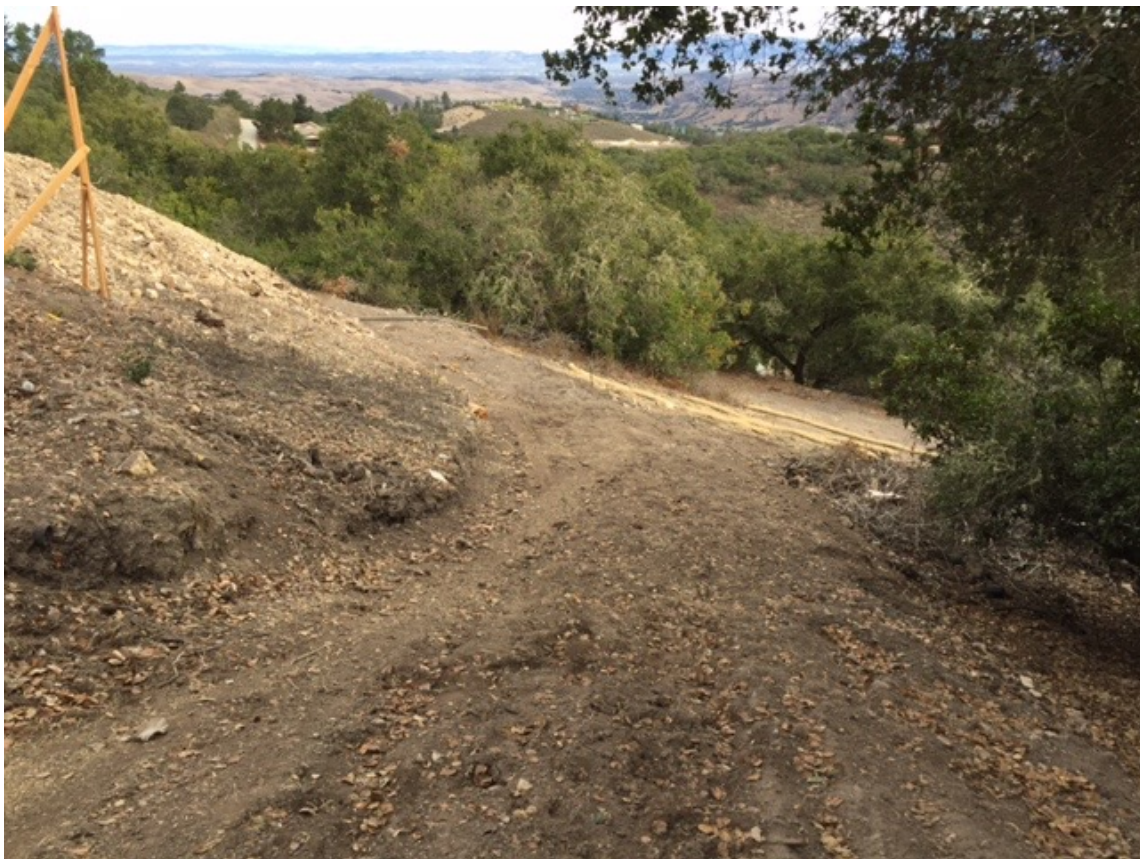
Figure 12. Restore lower road/path and apply native seed mix and soil stabilization measures to exposed slope. As of late, straw wattles have been installed toward lower section of slope (right of center).
