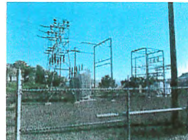
Photo 8. A typical substation with step-up transformer
