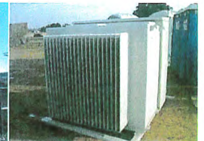
Photo 9. A step-up transformer
