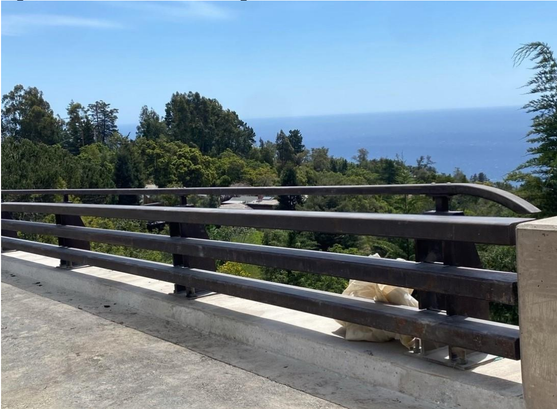
Figure 1-3 Stained ST-75B Bridge Rail
