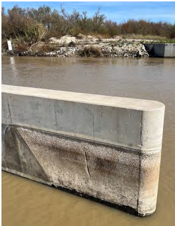
Figure 1: Gash in abutment
