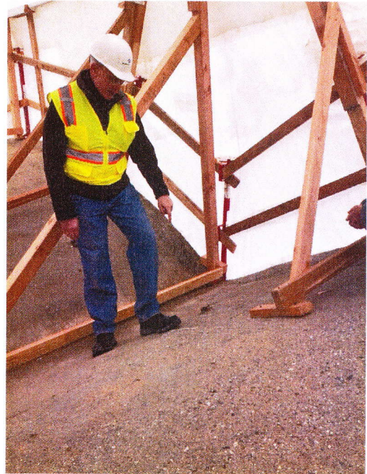
Steel frame embedded and protruding through the concrete roof shell
