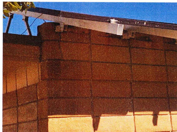
Garage roof parapet cracked below solar panel and along parapet top
