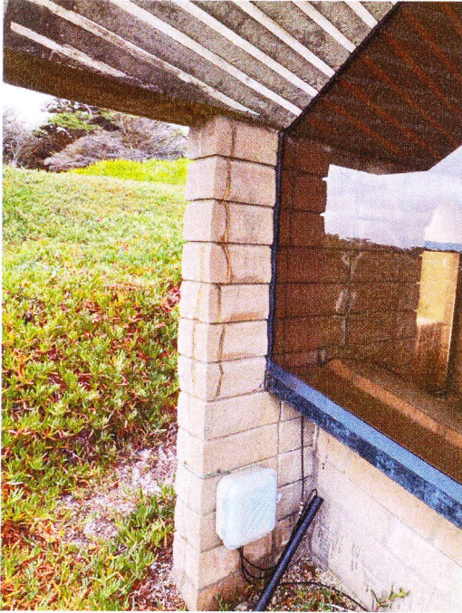
Cracked and previously repaired
