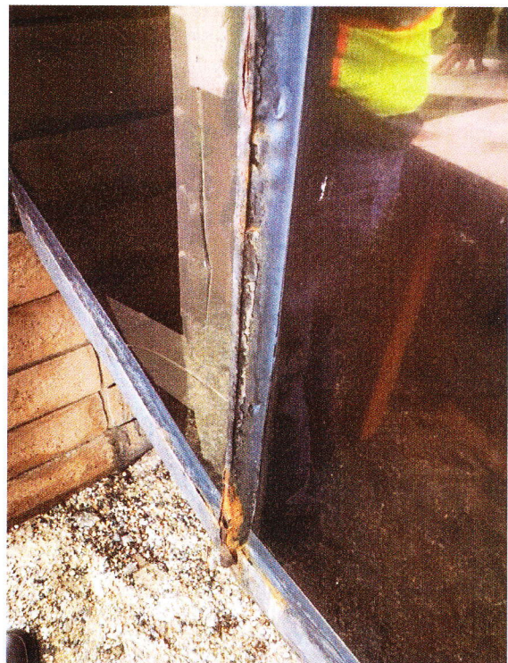
Considerable corrosion of mullions and sill
