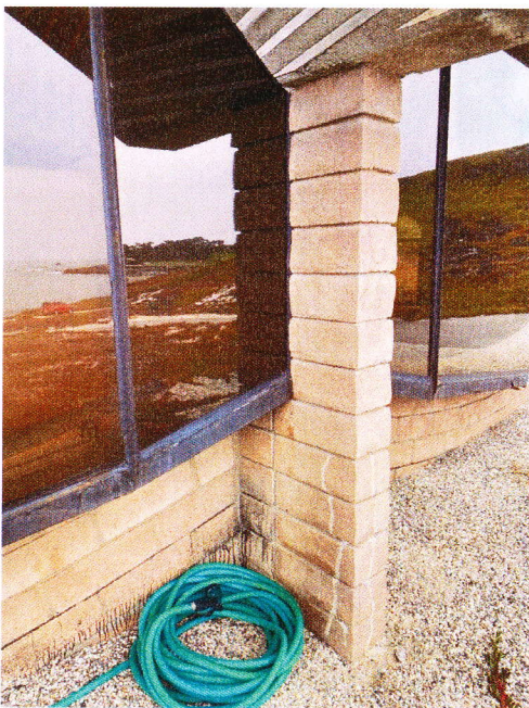
Moisture intrusion from grade as well
